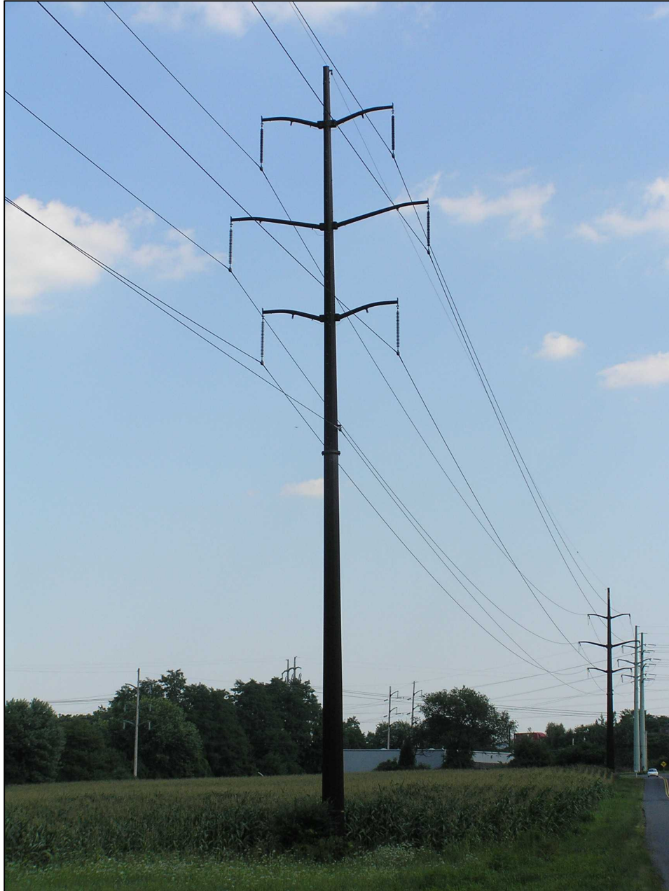
Figure 2. Example of monopole to be used on Achela Connector line.
