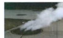
Picture to the left indicates a possible steam leak venting out of a manhole.
