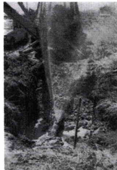
Photo courtesy of Hughes Supply - Utilities Services Group.
