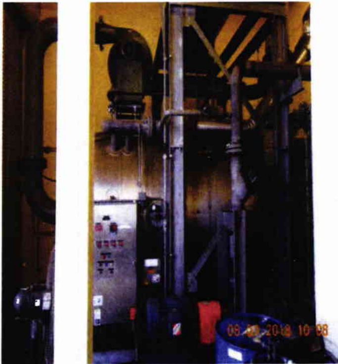
Sludge Drying Equipment
