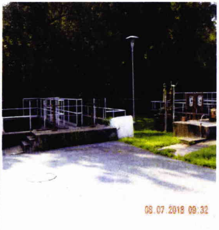
Original Contact Tanks (not used)
