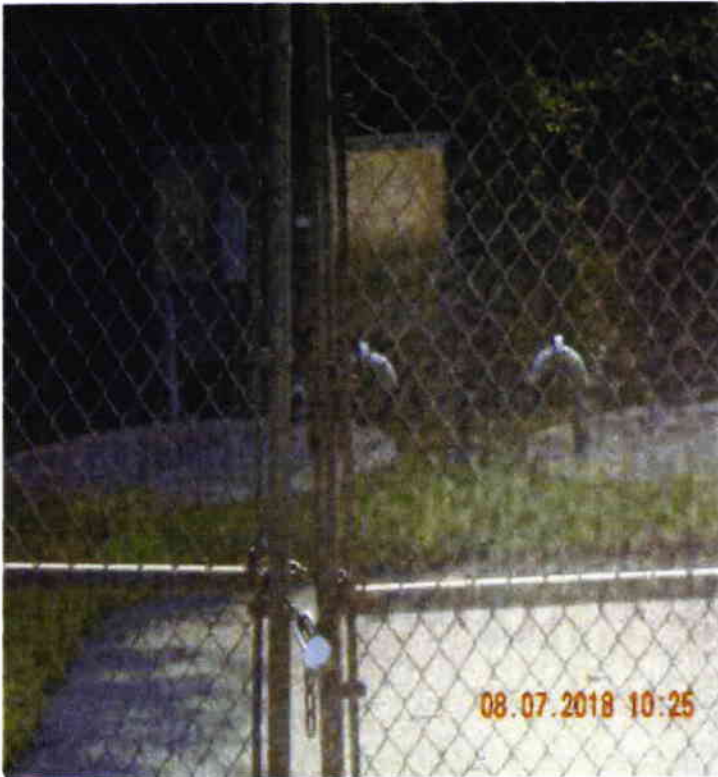
Buddies Place Pump Station
