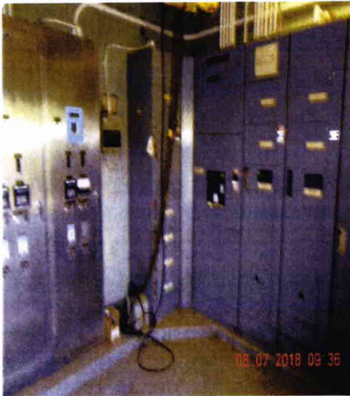
Original Construction – Wet Well Control Panel
