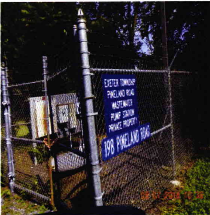
Pineland Pump Station
