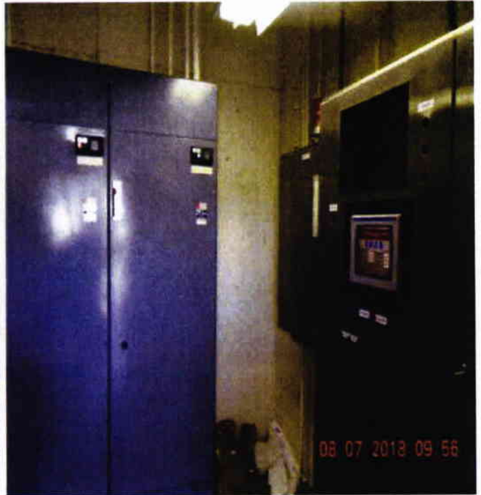
Blower Control Panel
