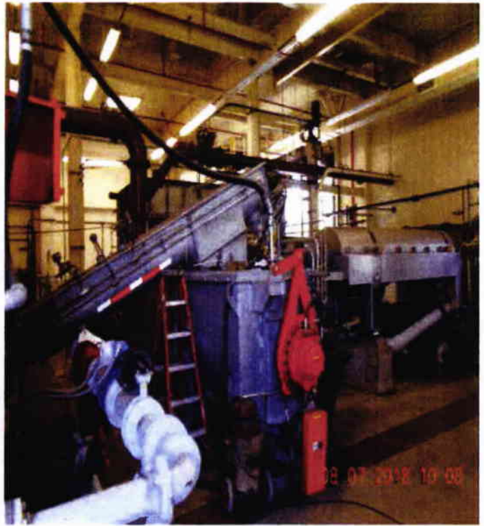
Sludge Drying Equipment
