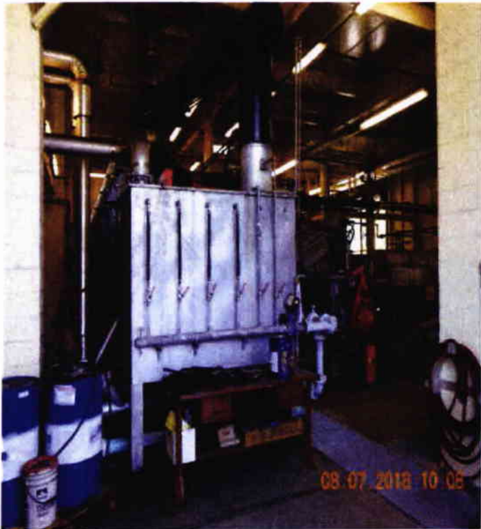
Sludge Drying Equipment
