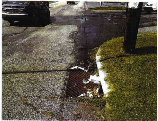
Catch Basin E-PO3 with litter present
