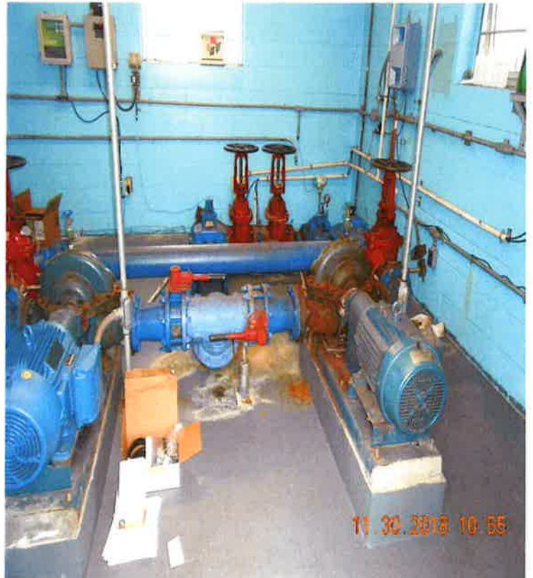
Tank Booster Pumps
