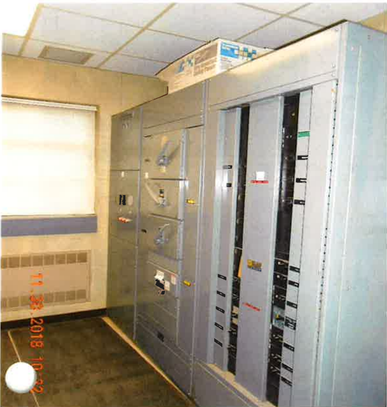
Control Panel Steelton Plant Inspection Pictures
