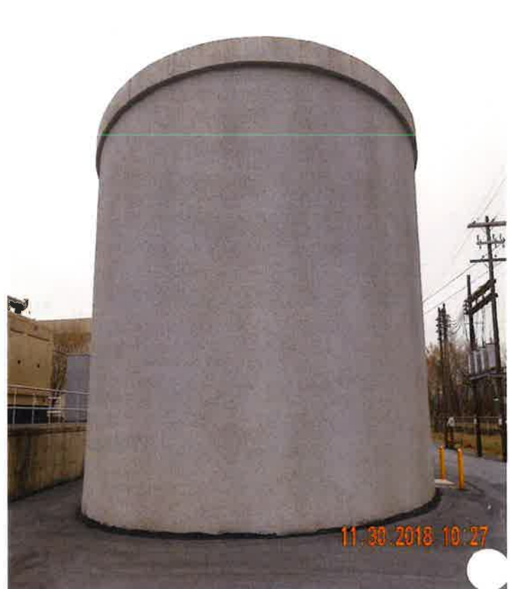
Chlorine Contact Tank (2017)
