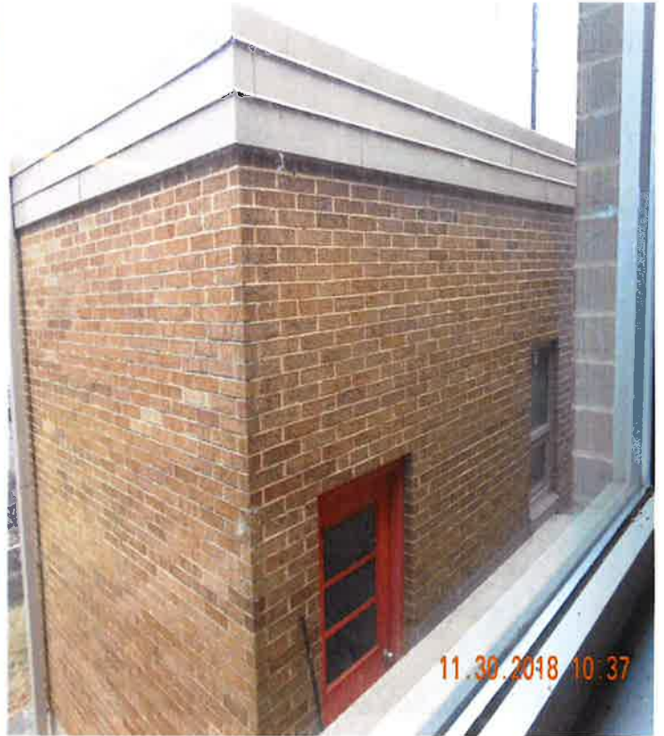
Back Wash Station
