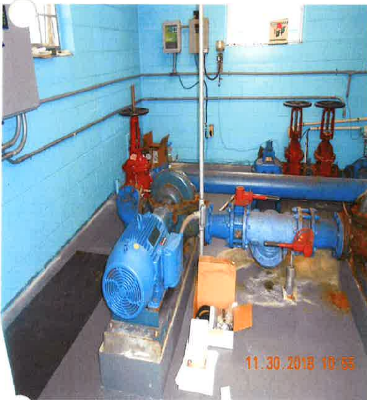
Tank Booster Pumps
