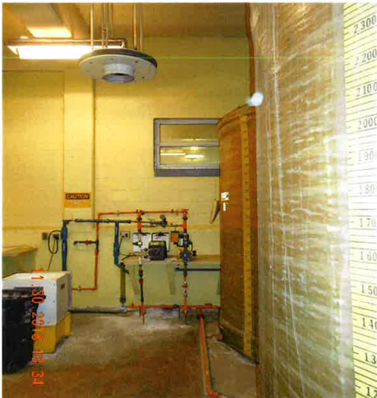
Steelton Plant Inspection Pictures Chemical Room
