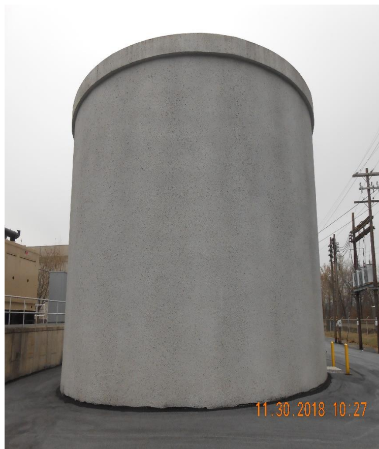
Chlorine Contact Tank (2017)
