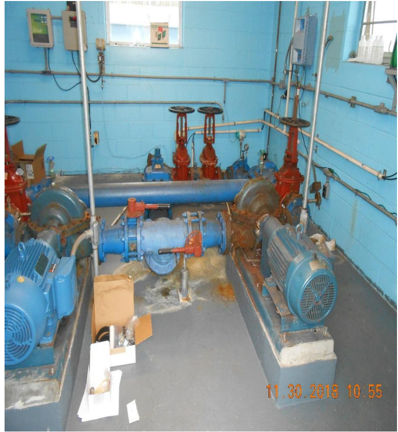
Tank Booster Pumps
