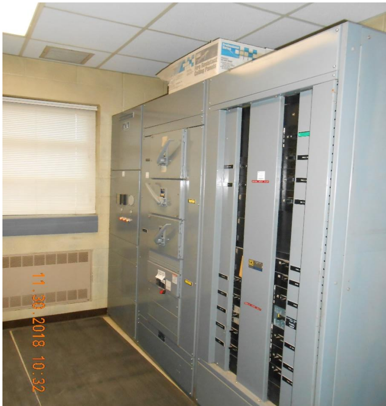
Control Panel Steelton Plant Inspection Pictures
