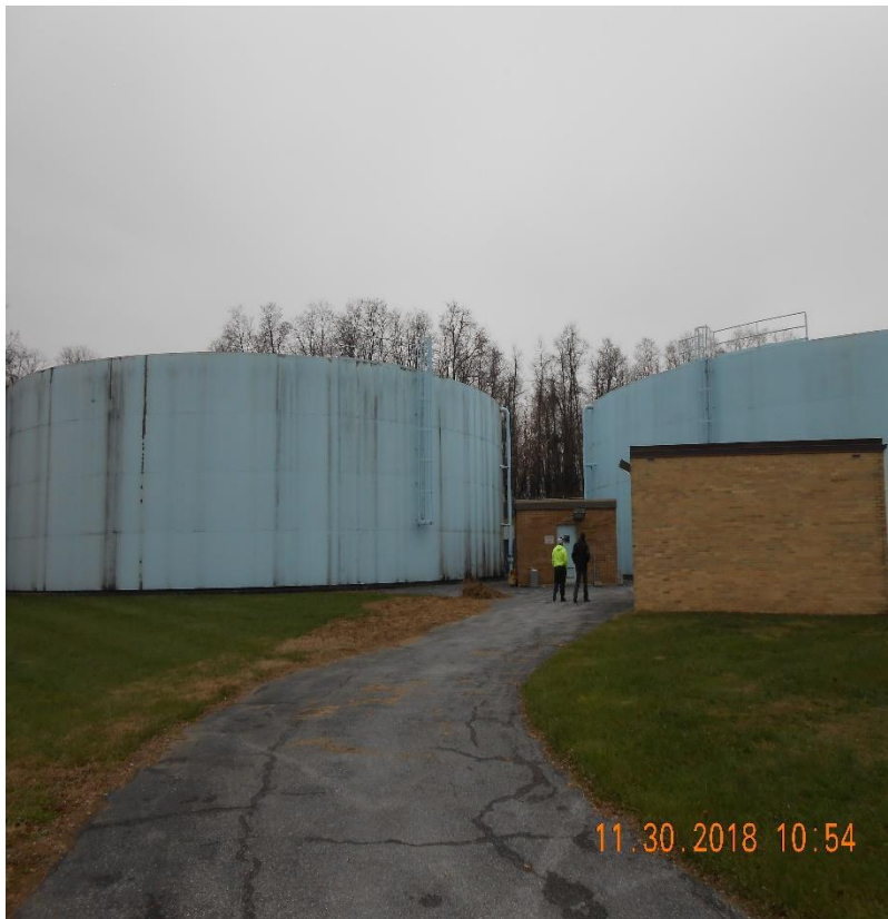
2 Million Gallon Tanks
