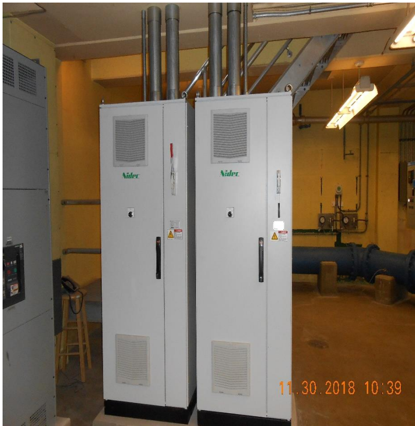
Piping Gallery & Booster Pumps Steelton Plant Inspection Pictures
