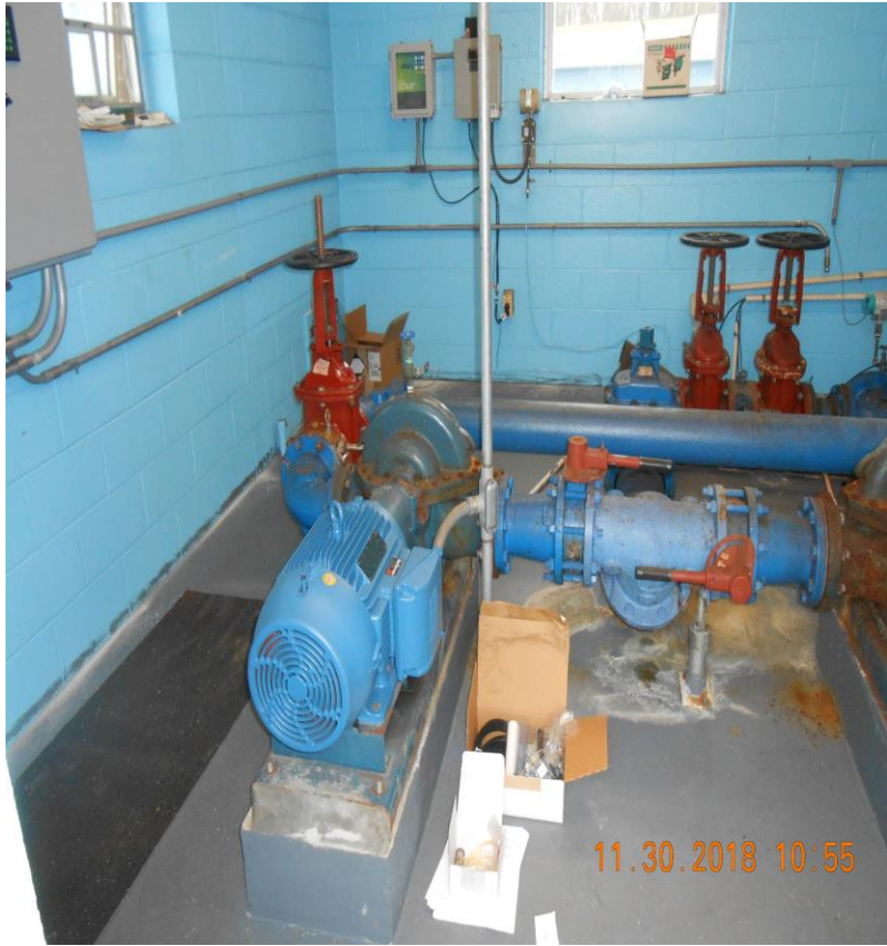
Tank Booster Pumps
