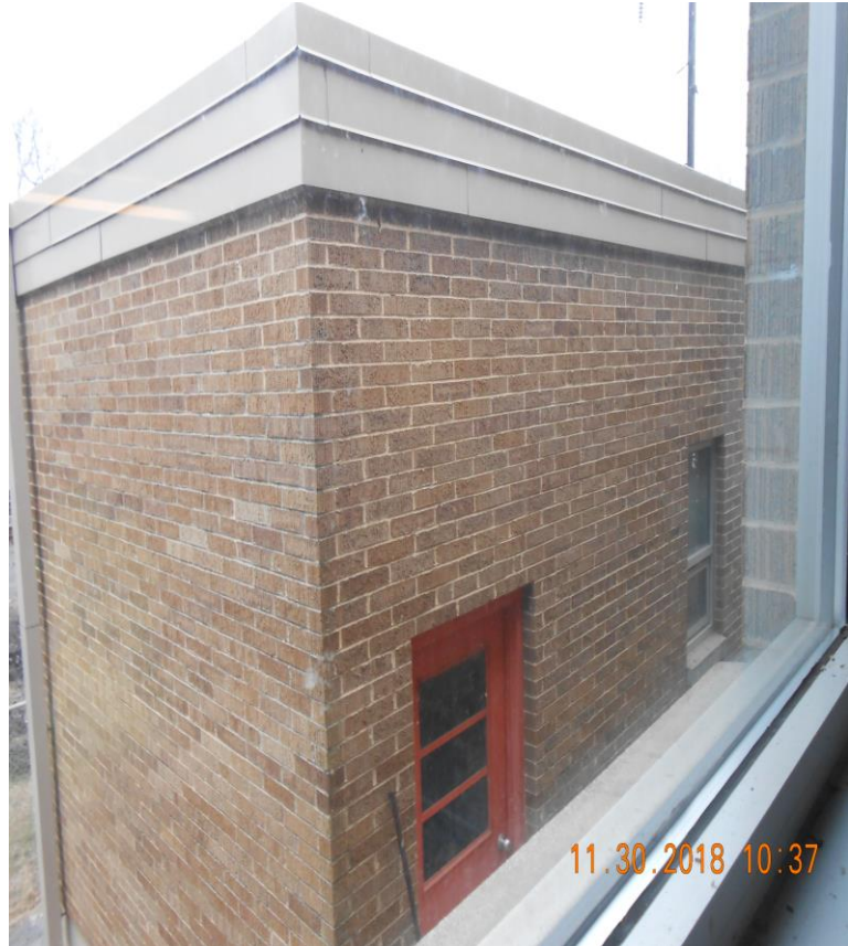
Back Wash Station
