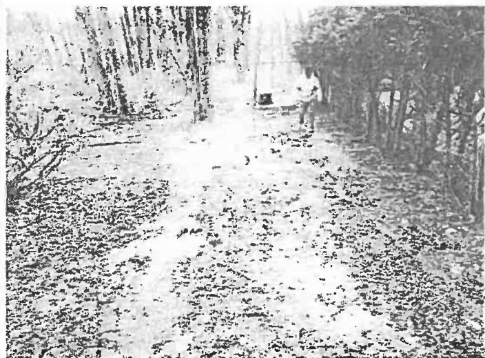
11. Lime put down on the ground near the Xylem portable pump used to pump out of the last manhole on the Stoney Creek No. 2 Interceptor.
