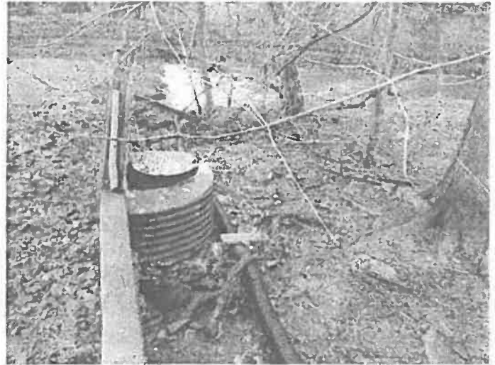
14. Some sewage solids around the manhole.
