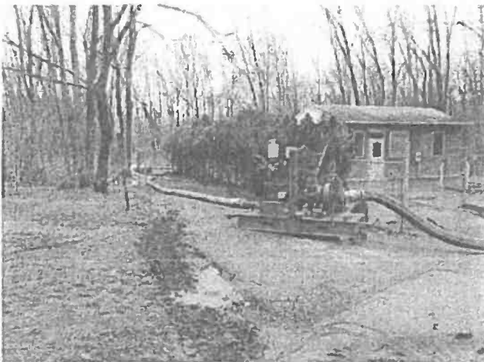
11. The Second Xylem Pump discharging from manhole on the Stoney Creek Interceptor in the pump station driveway.
