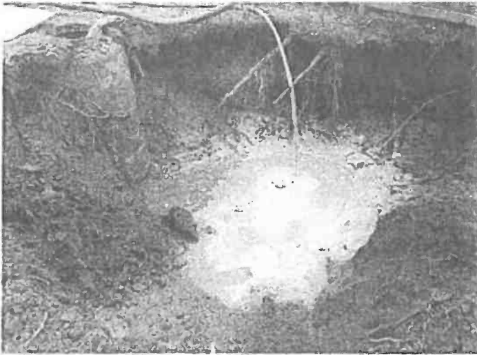
1. The beginning of the excavation near manhole #2 on the 24 inch Section of the Stoney Creek 2. Interceptor, 02/25/16.
