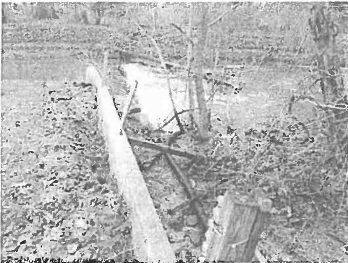
13. Manhole 2A overflowing to Stoney Creek, 02/25/15.
