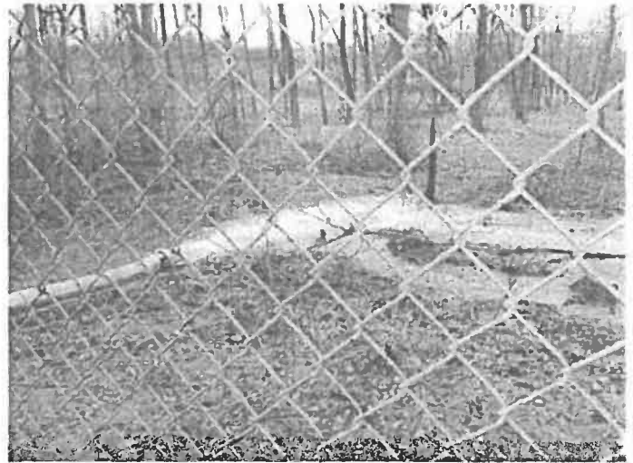
16. The stream of sewage flowing out of the Xylem Pumps onto the ground and to Stoney Creek.
