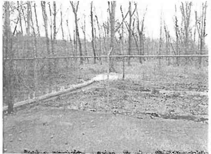
8. The second Xylem Pump discharging to the woods and creek from the manhole on the Stoney Creek Interceptor immediately upstream of the wet well.
