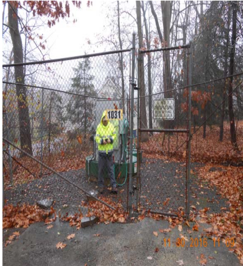
Schultz Road Pump Station
