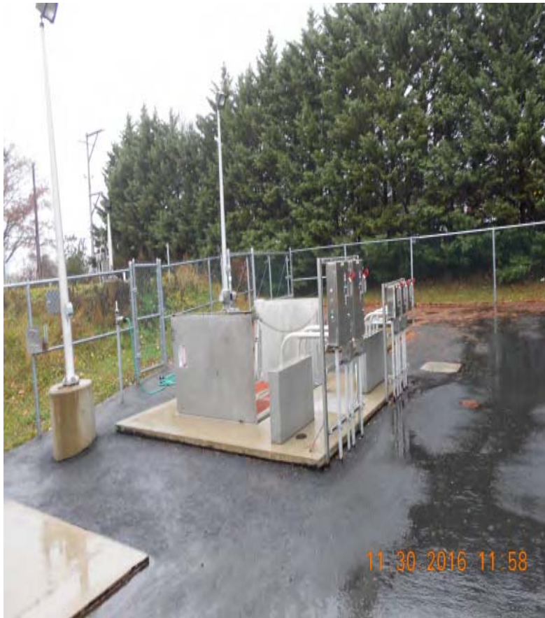
Einstein Pump Station
