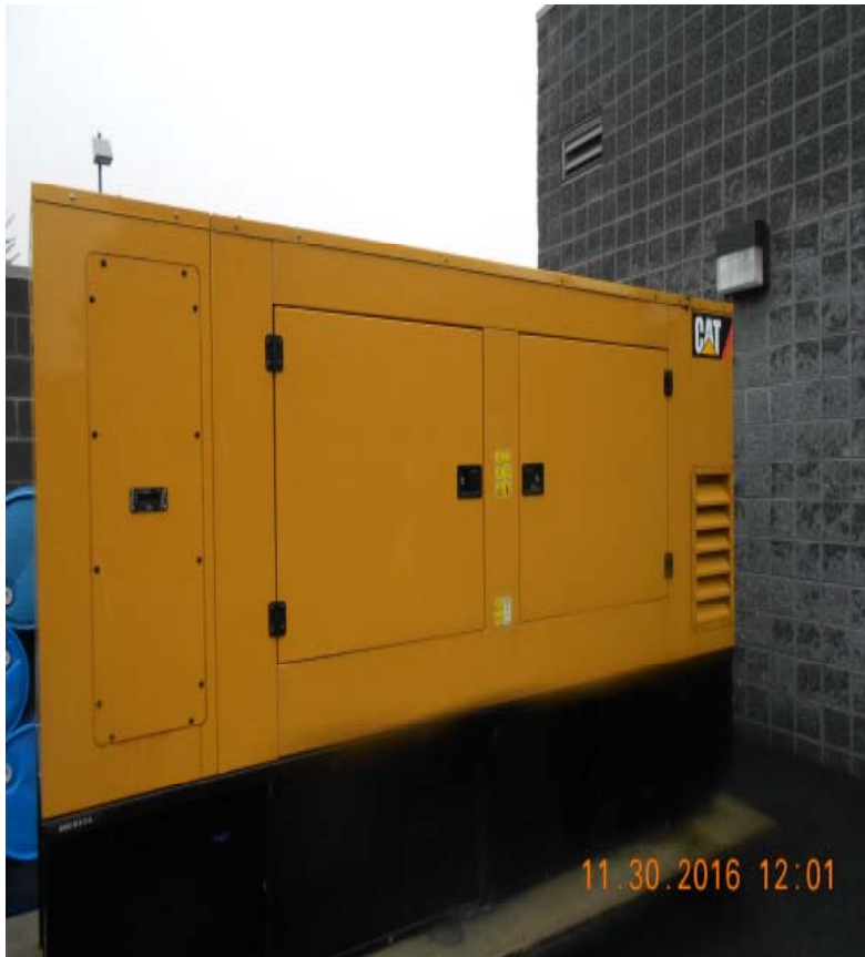
Einstein Pump Station
