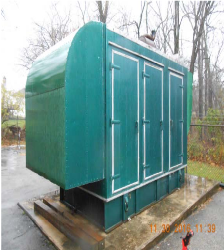
Germantown Pike Pump Station
