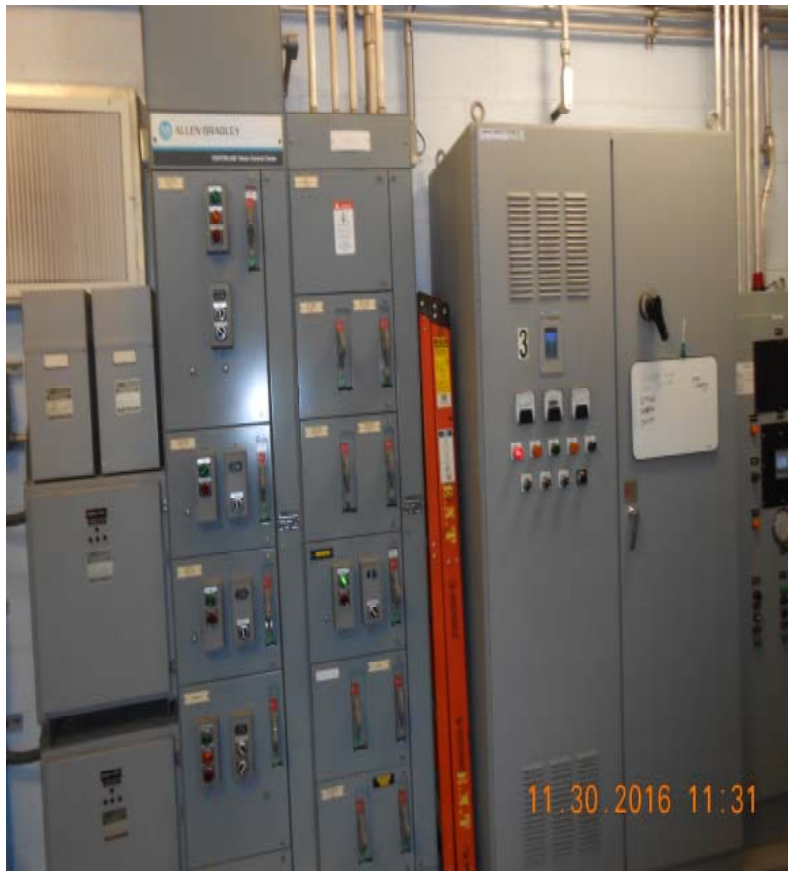
Germantown Pike Pump Station
