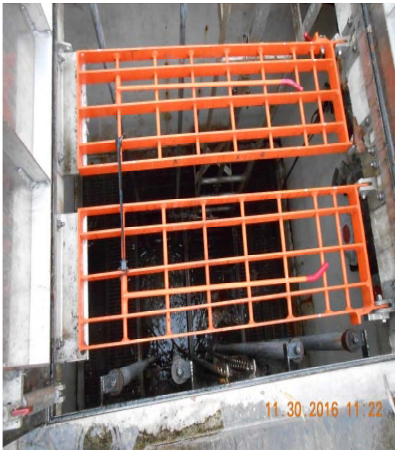
Burnside Ave. Pump Station East Norriton Inspections
