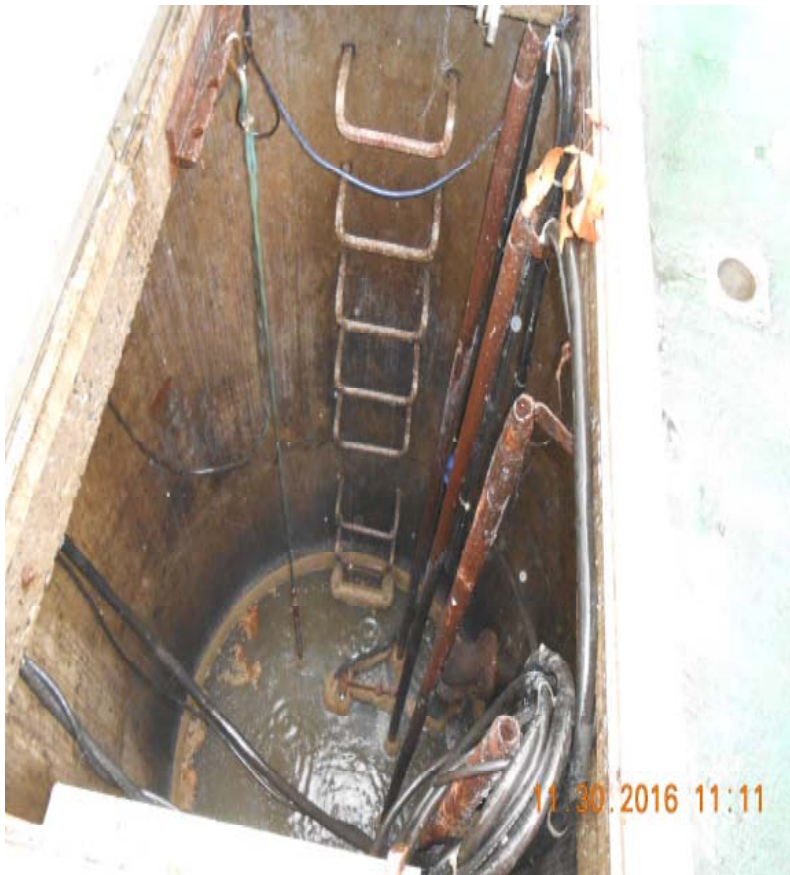
Schultz Road Pump Station
