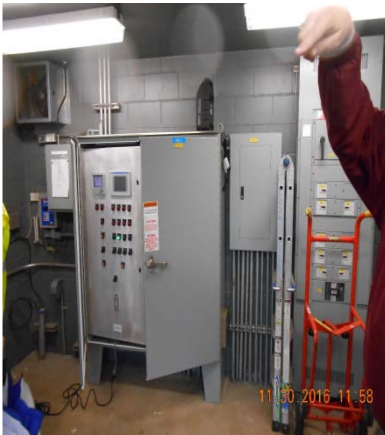
East Norriton Inspections Einstein Pump Station
