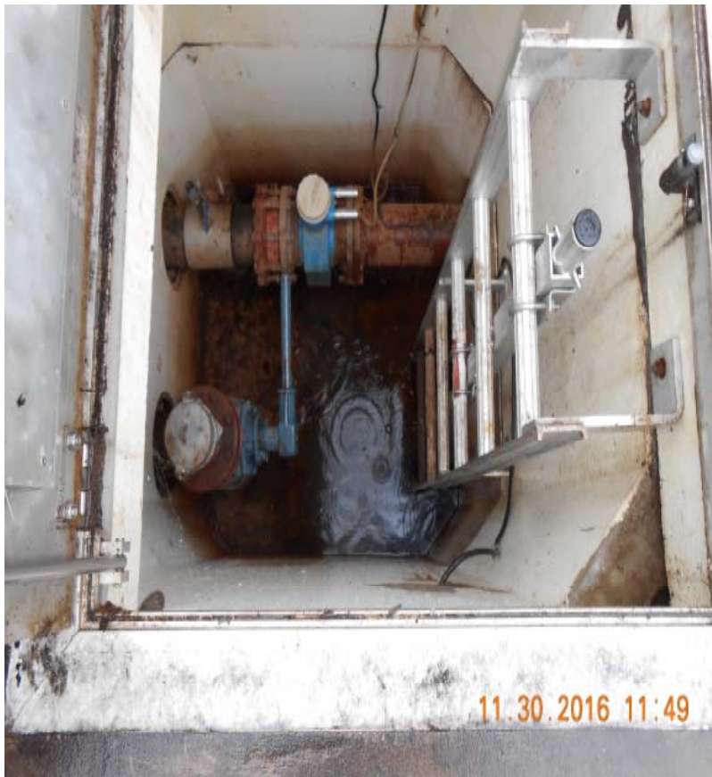
Germantown Pike Pump Station
