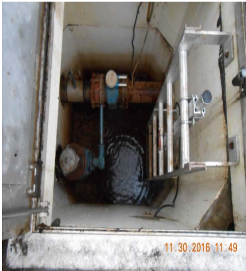
Whitehall Pump Station
