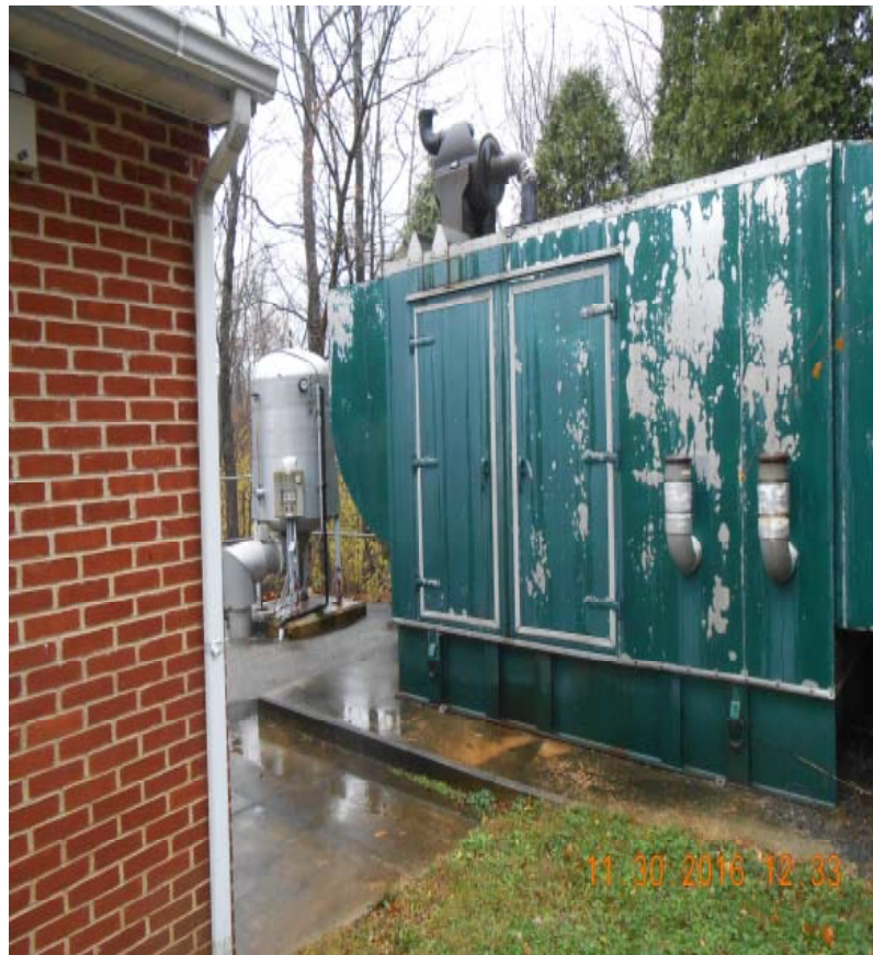
Timberlake Pump Station
