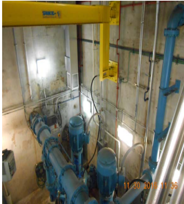
Germantown Pike Pump Station
