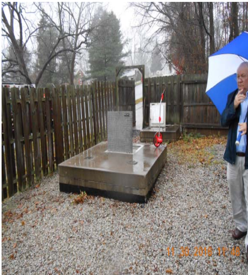
Whitehall Pump Station
