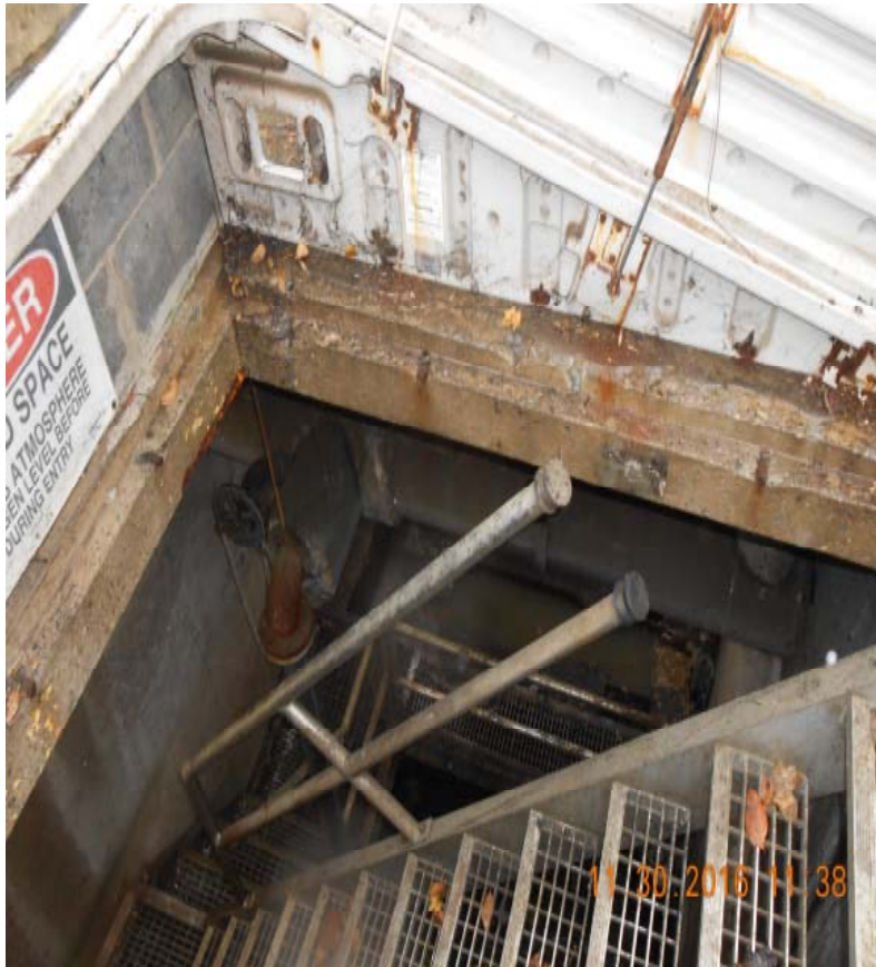
Germantown Pike Pump Station
