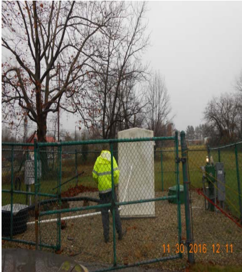
Whitehall Pump Station
