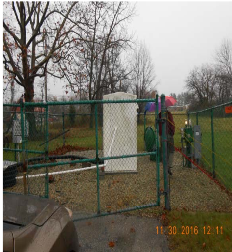
Whitehall Pump Station
