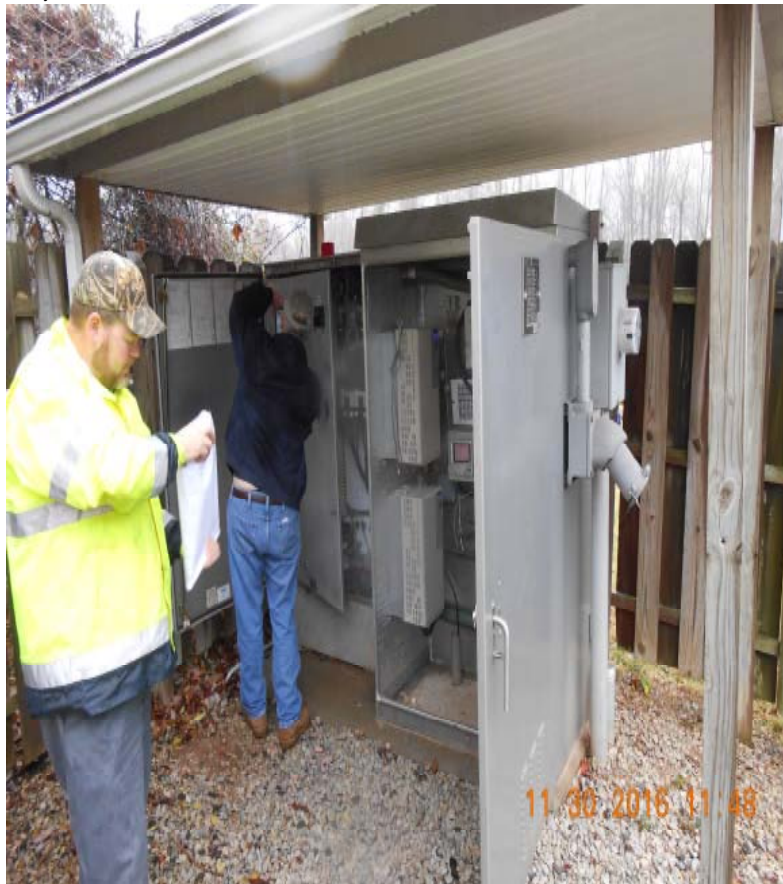
Whitehall Pump Station
