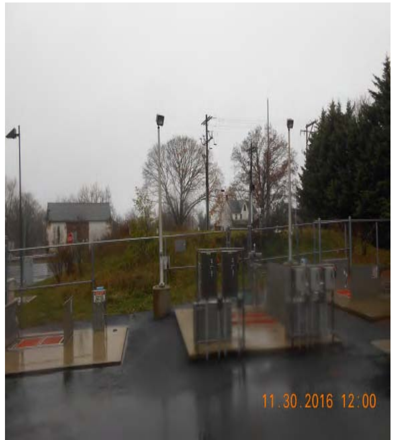
Einstein Pump Station
