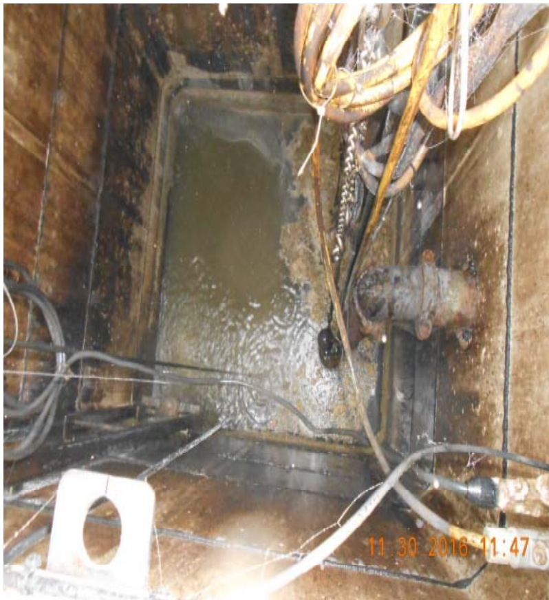
Whitehall Pump Station
