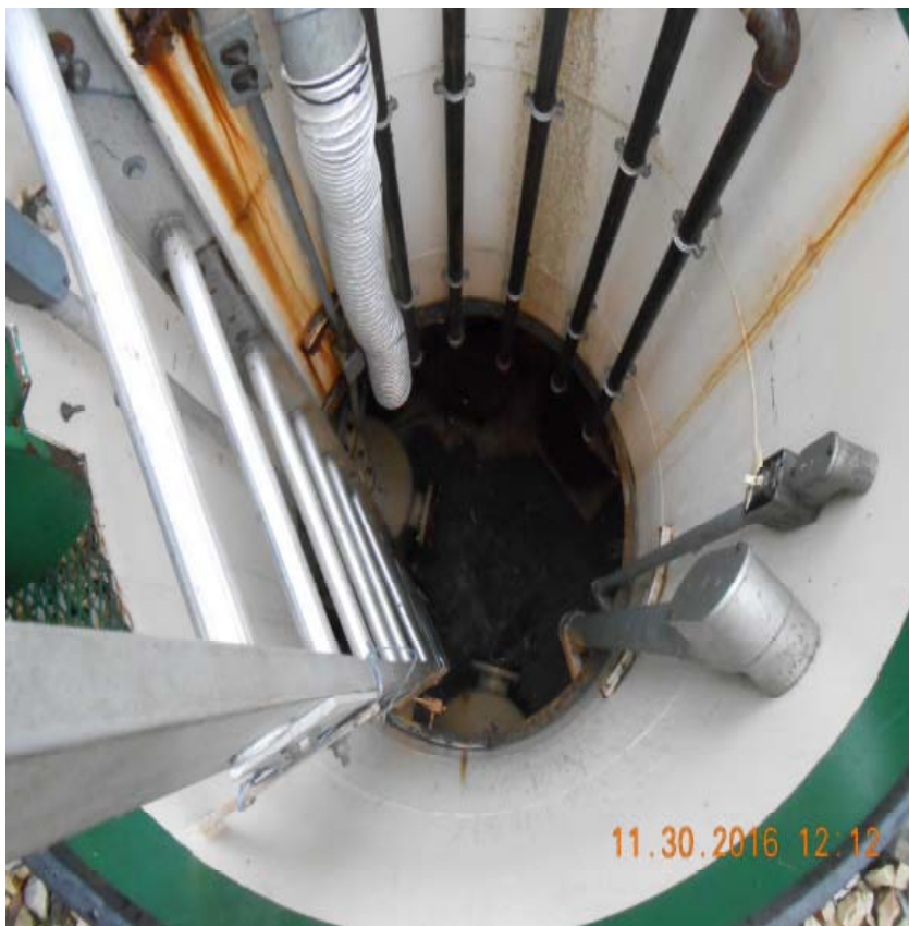
Whitehall Pump Station East Norriton Inspections
