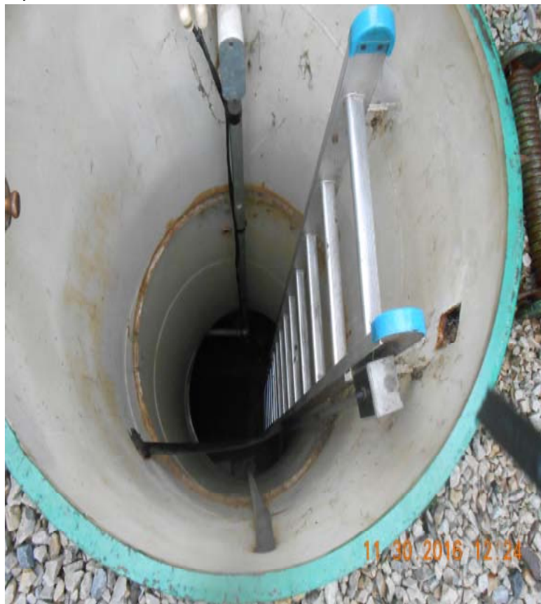
Felton Road Pump Station
