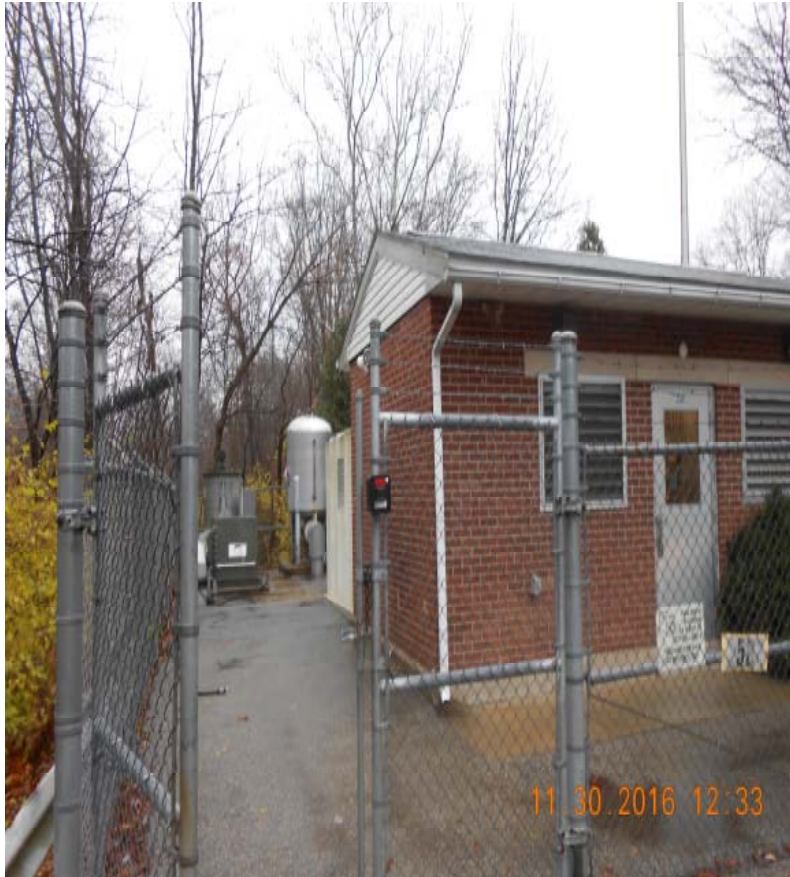
Timberlake Pump Station
