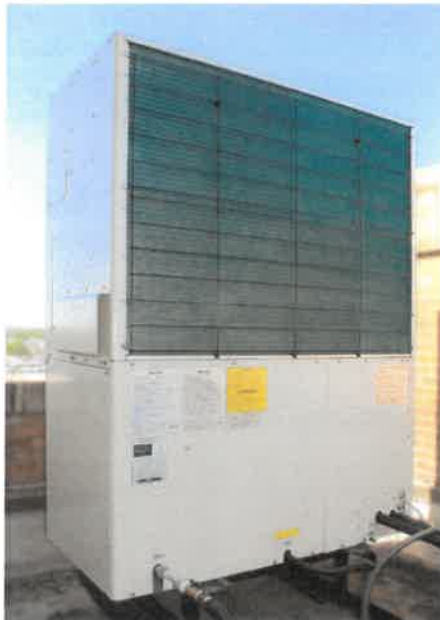
△ 10-ton Yanmar natural gas VRF heat pump located on the Bok Building rooftop.
