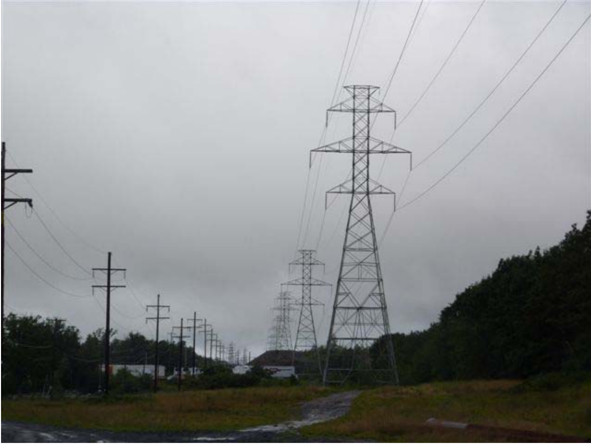
Figure 1: Typical Susquehanna-Harwood #1 & #2 230 kV Towers
