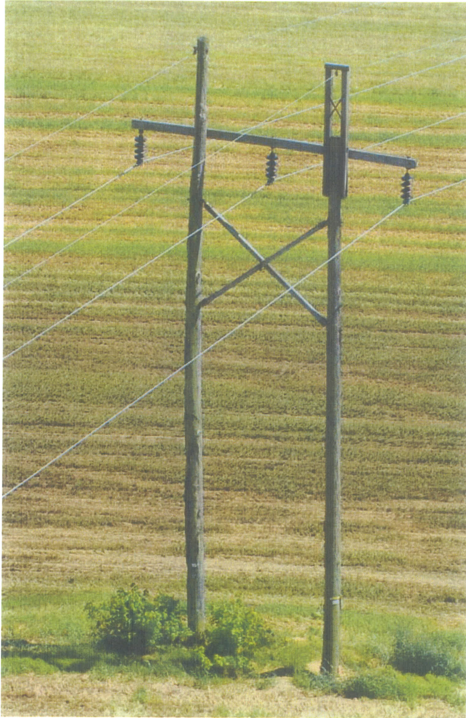
Typical H-Frame Structure on Blooming Grove – Honesdale Line
