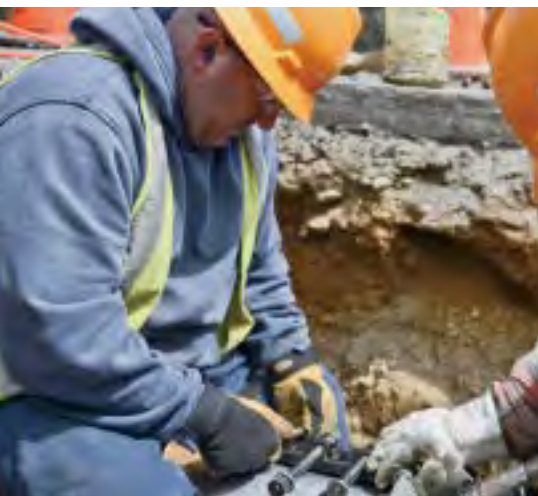
(Left) Gas Fitter Todd M. Miraglio repairs the gas system in Rockland County.
