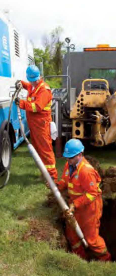
(Upper left) Mechanic A Alexander Hernandez works on our extensive electric cable system. (Left) Mechanic A Kenneth E. Gilleo III and Outside Plant Mechanic George B. Shute at work on the gas system. (Right) Youngsters learn about marine ecology of the East River at the World Science Festival, sponsored in part by Con Edison.
