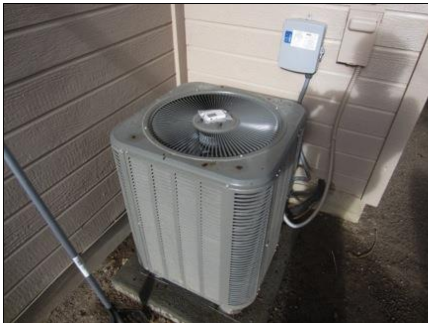
Figure 28. Motor Logger on Condenser
