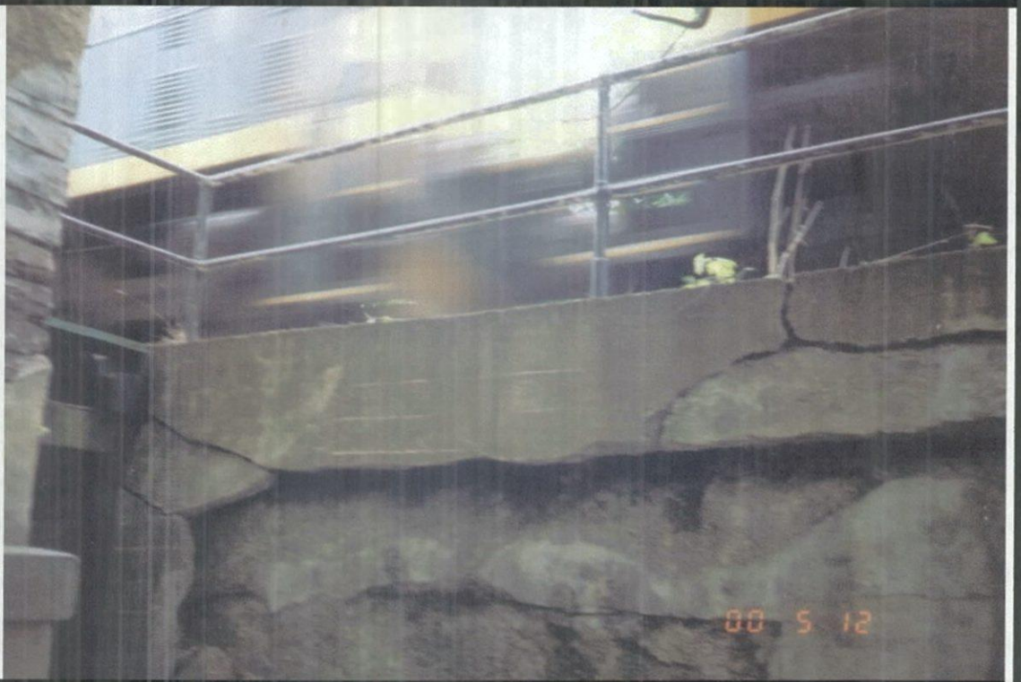
First Collapse Photo Date: 5/12/00
