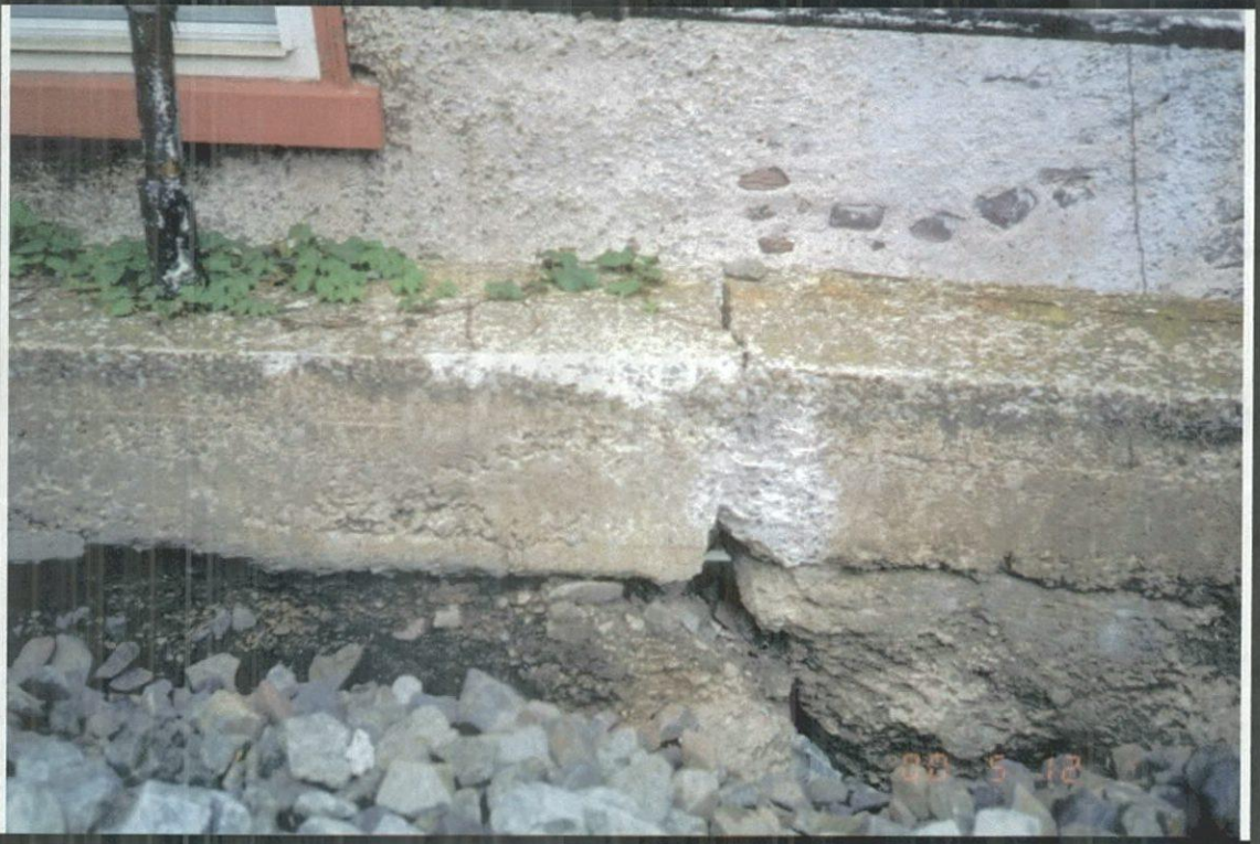
First Collapse Photo Date: 5/12/00
