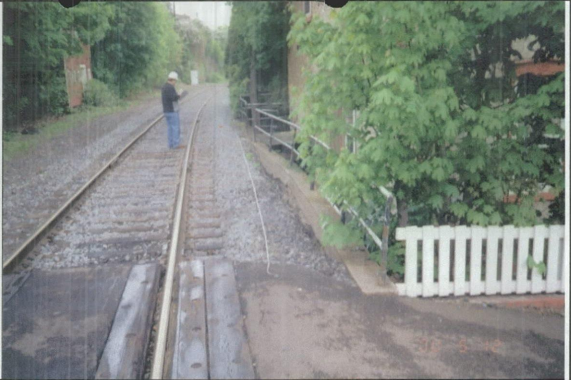
First Collapse Photo Date: 5/12/00
