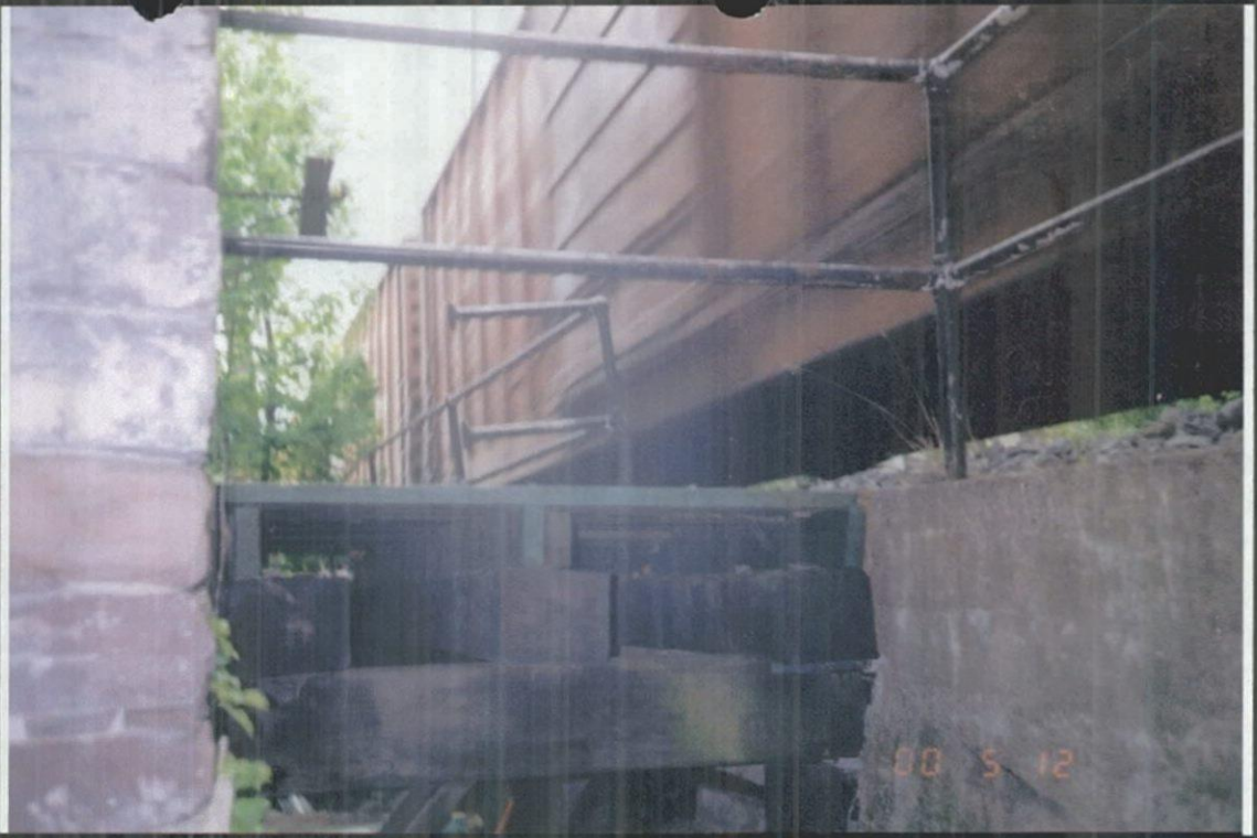
First Collapse Photo Date: 5/12/00
