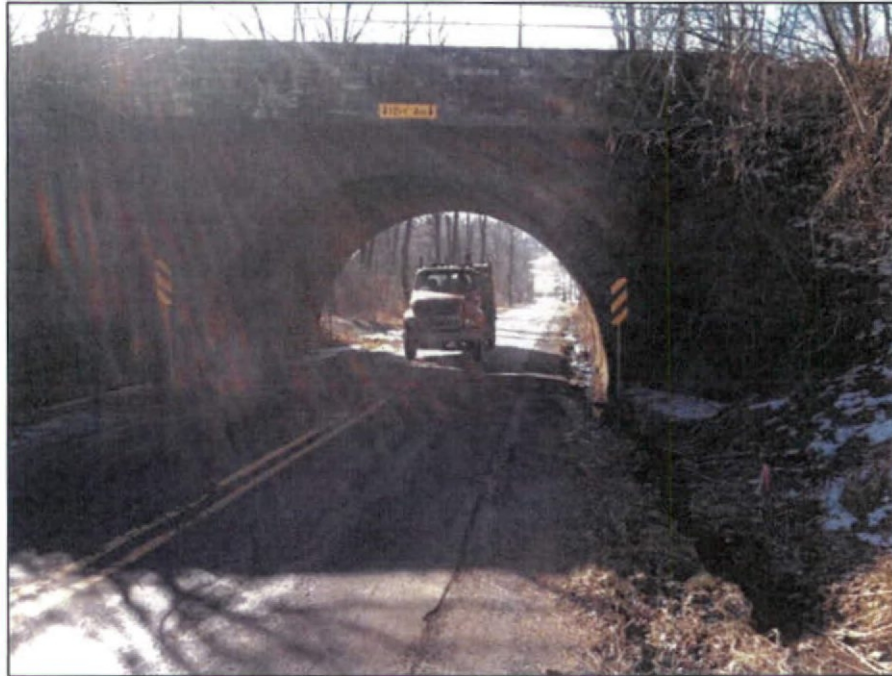
Photo 7 – Northbound truck traveling through underpass. View from north side of underpass looking south.
