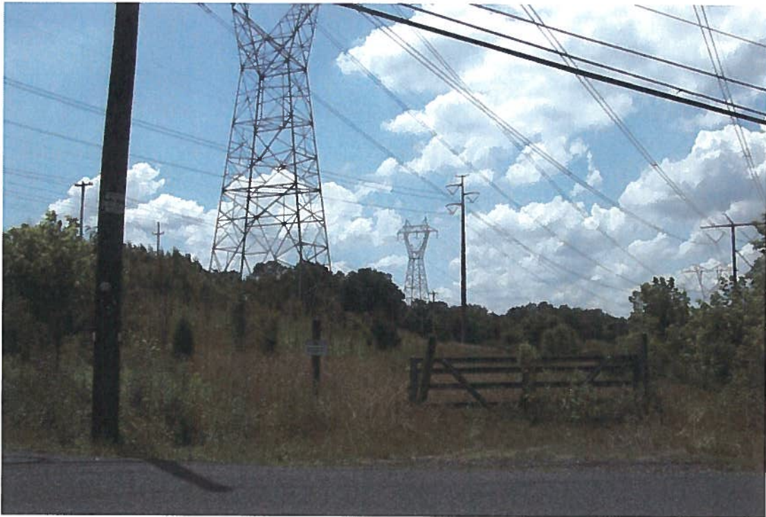
VIEW FACING WEST ALONG THE CORRIDOR, FROM THE EAST END, AS SEEN FROM PERKIOMEN CREEK ROAD.
