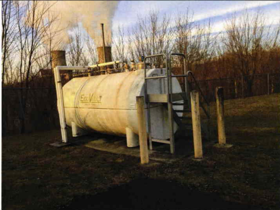
22 Possum Hollow WWTP- Outside Oil Tank
