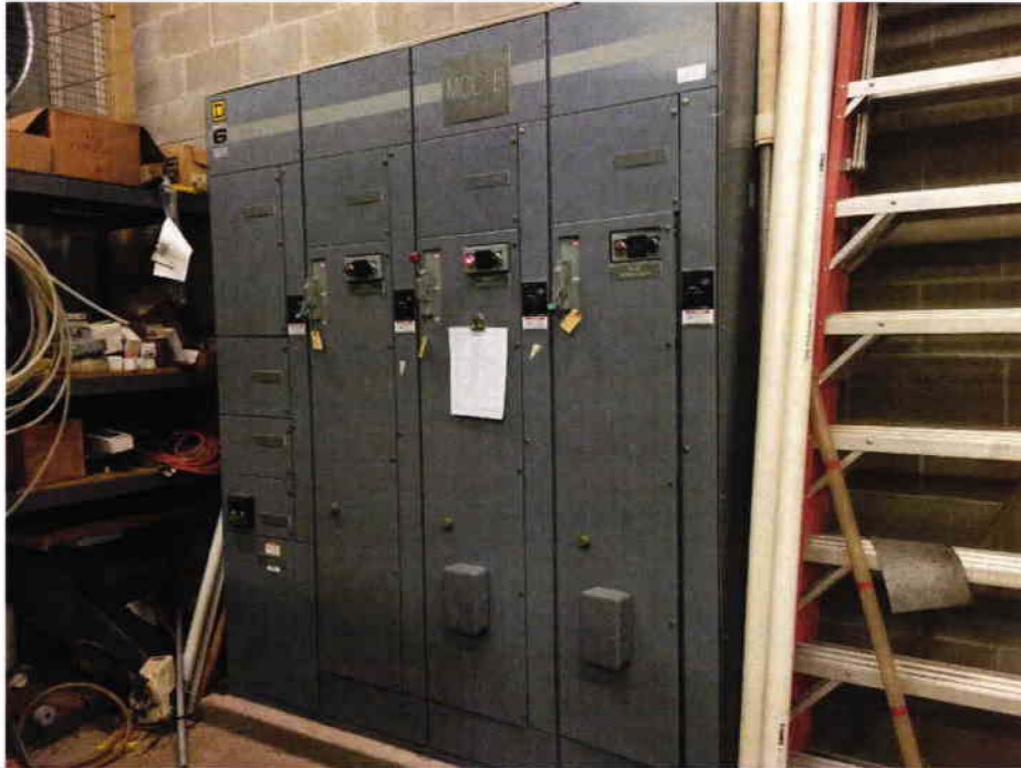
19 Possum Hollow WWTP- Blower MCC
