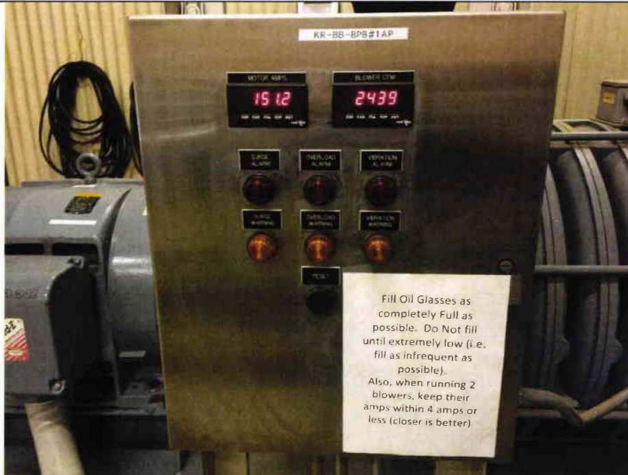
16 Blower Control Panel
