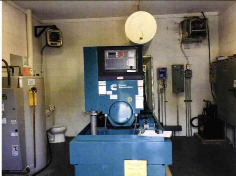
4 Pump Station #19 – Building Interior.
