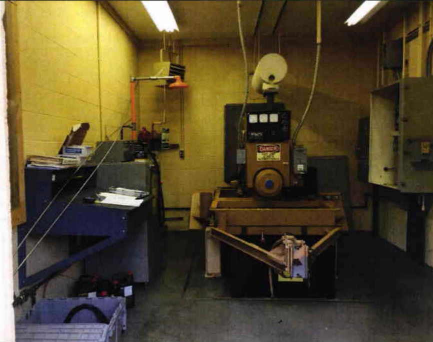
4 Pump Station #7 – Building Interior.
