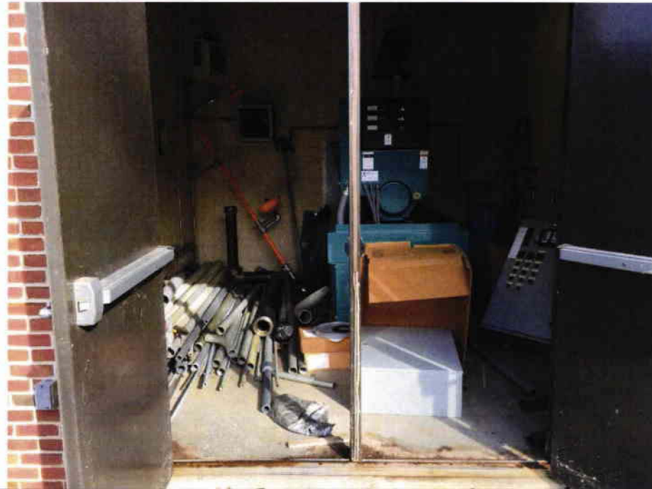
3 Pump Station #9 –Building Interior.
