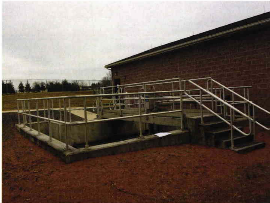
3 Aerated Grit Chamber at Headworks
