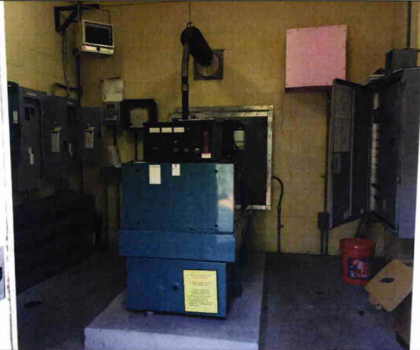
4 Pump Station #13 – Building Interior.
