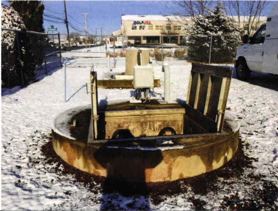
1 Pump Station #10 – Wet Well Exterior.
