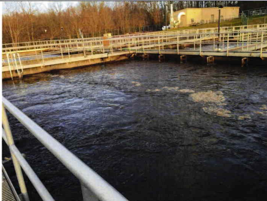
20 Possum Hollow WWTP- SBR Unit Aeration Chamber
