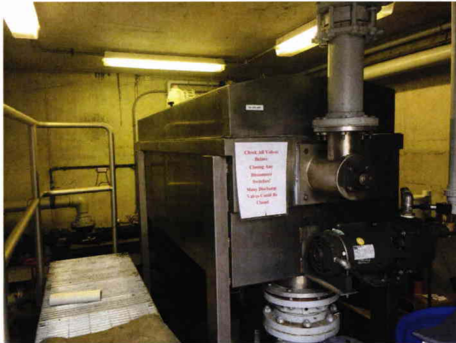
11 | Sludge Thickener Unit
