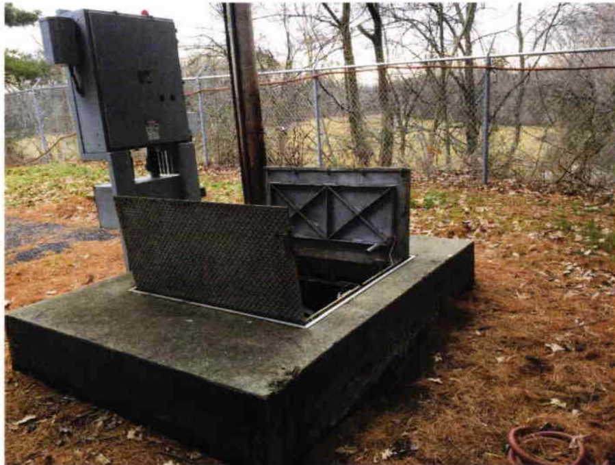
3 Pump Station #7 – Wet Well Exterior.
