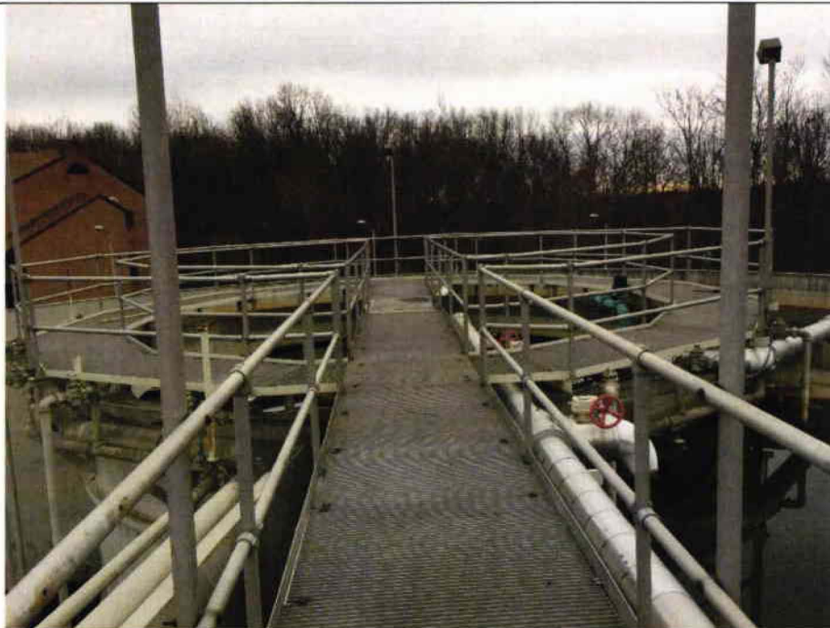
6 | Out of Service Sludge Digester
