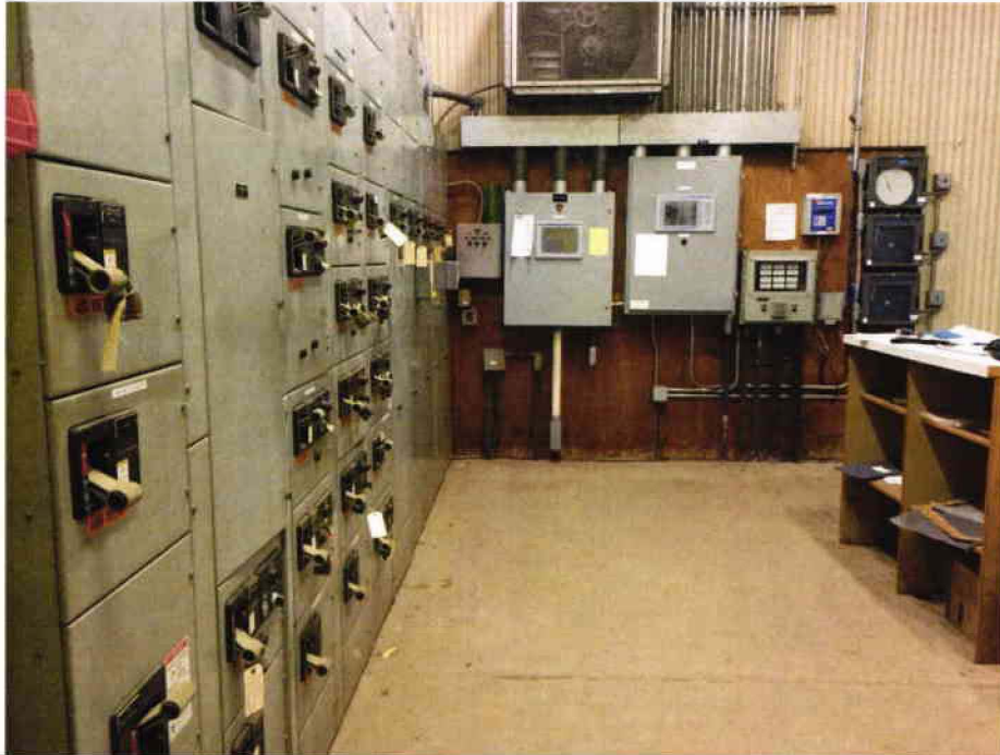
19 Building MCC, Blower Control Panel, Discharge Flow Meter and Chart Recorder
