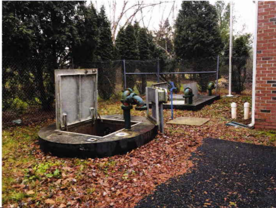
1 Pump Station #14 – Wet Well Exterior.
