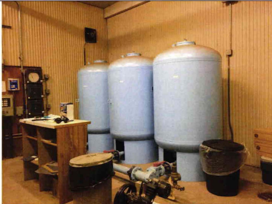
18 Yard Water Receiving Tanks
