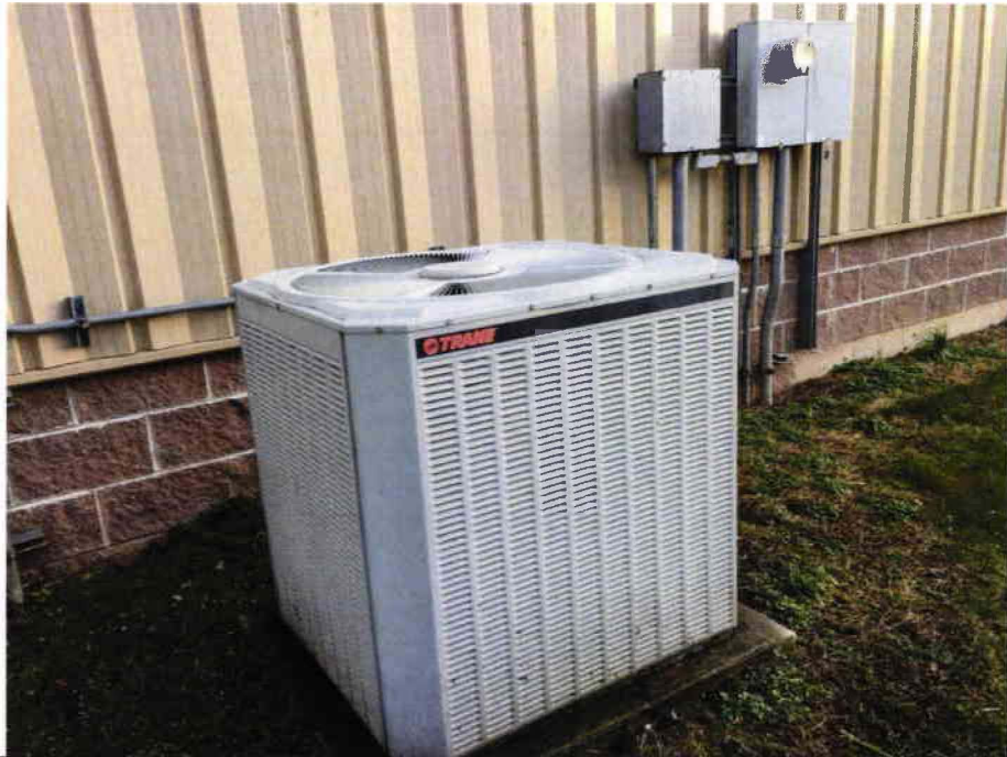
23 | Possum Hollow WWTP- Heat Pump
