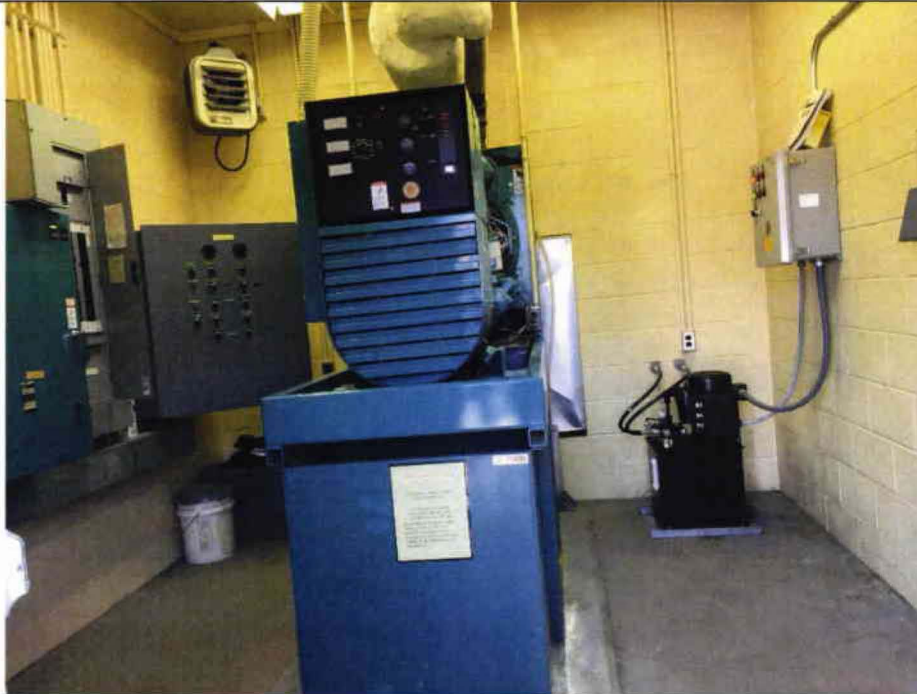
4 Pump Station #1 – Building Interior.
