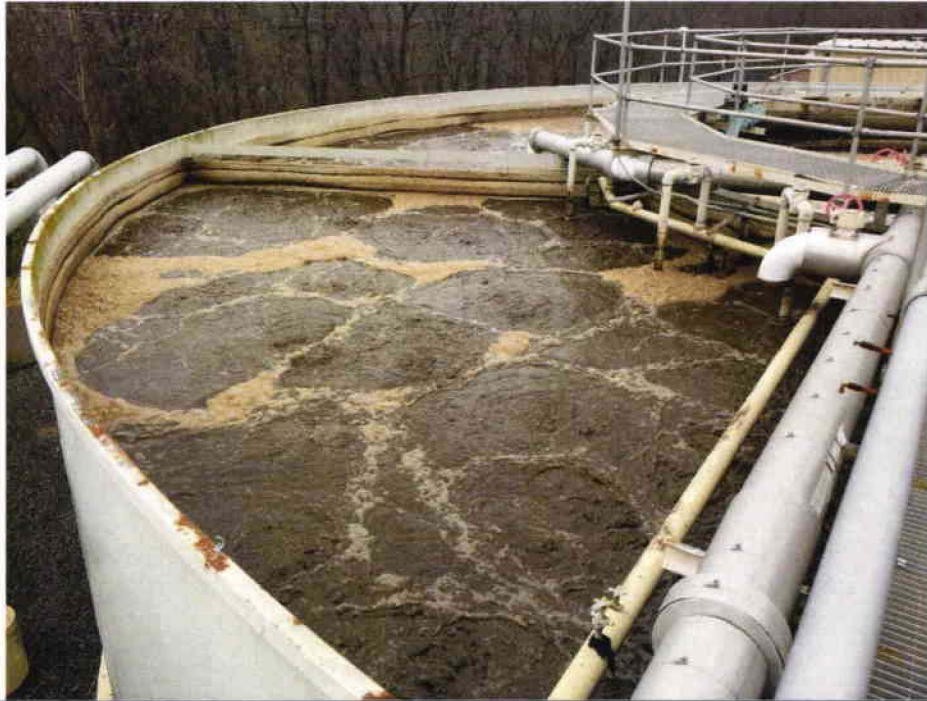
7 Sludge Digester Aeration Chamber
