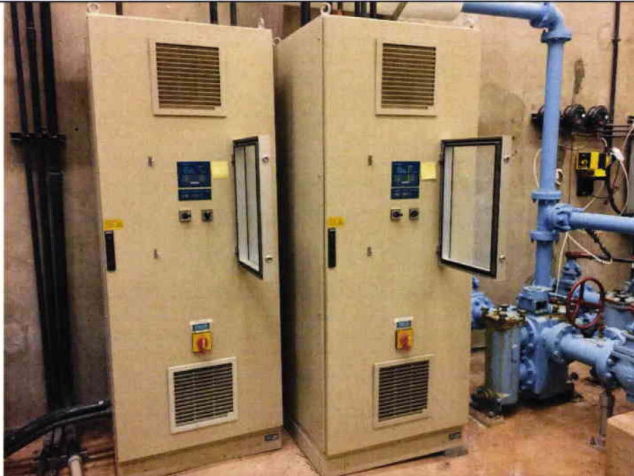
8 Possum Hollow WWTP- UV Units Control Panels
