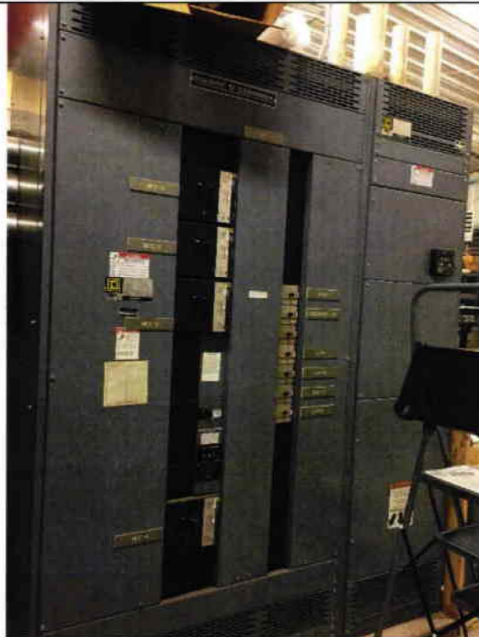
16 Possum Hollow WWTP- Building MCC
