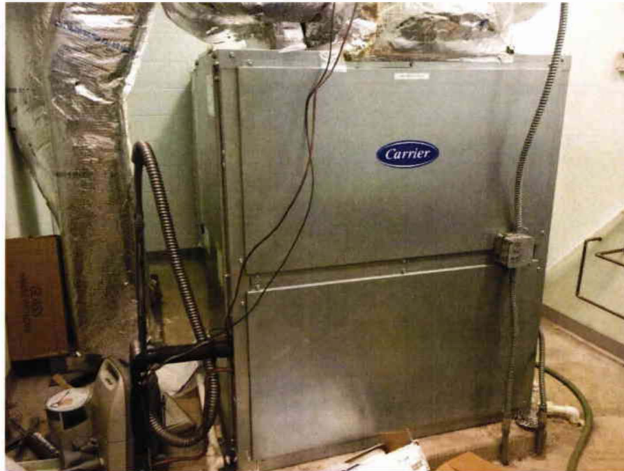
39 | Office Building Air Handler
