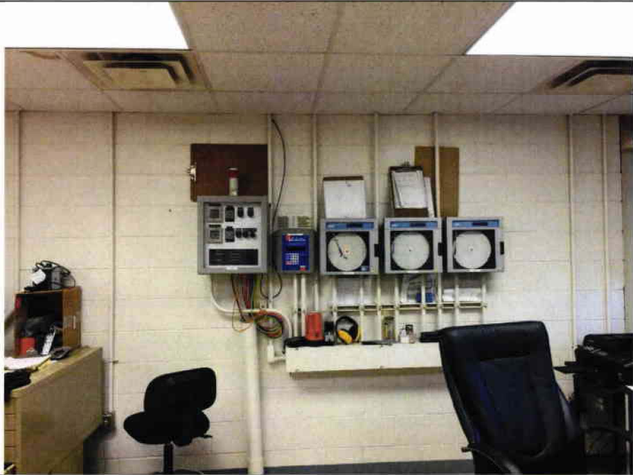
12 | Possum Hollow WWTP- Flow Recorder and Chart Recorders
