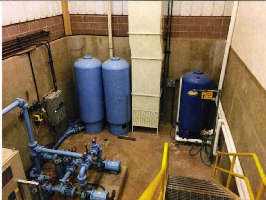
10 Possum Hollow WWTP- Yard Water Pump and Receiving Tanks (left) , Potable Water Tank (right)
