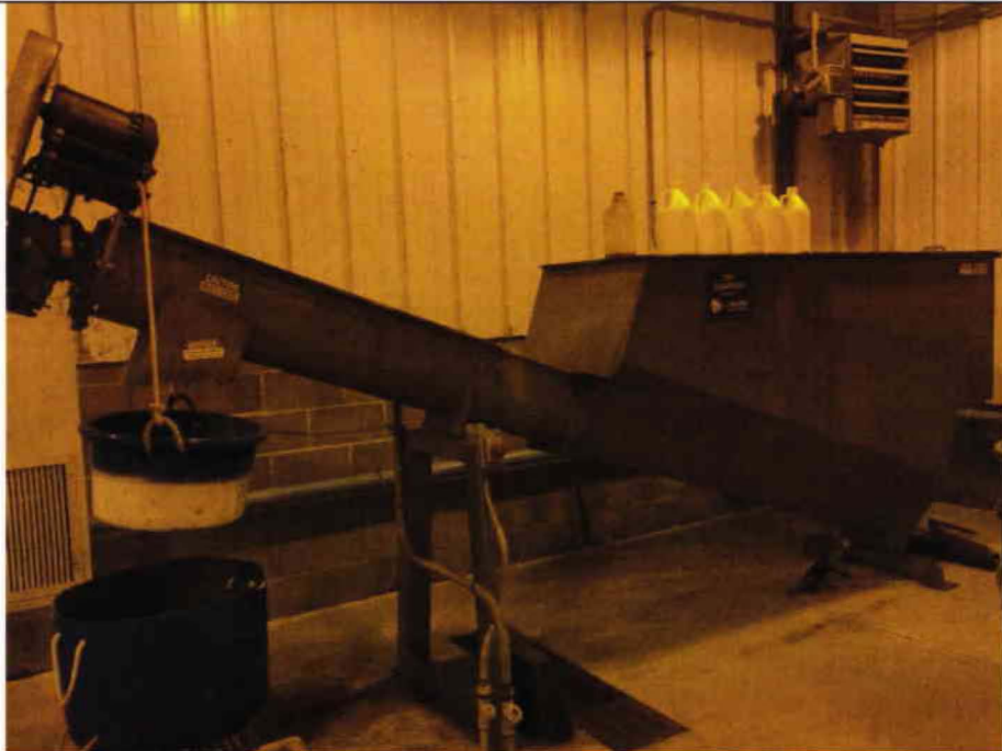
6 | Possum Hollow WWTP- Grit Classifier
