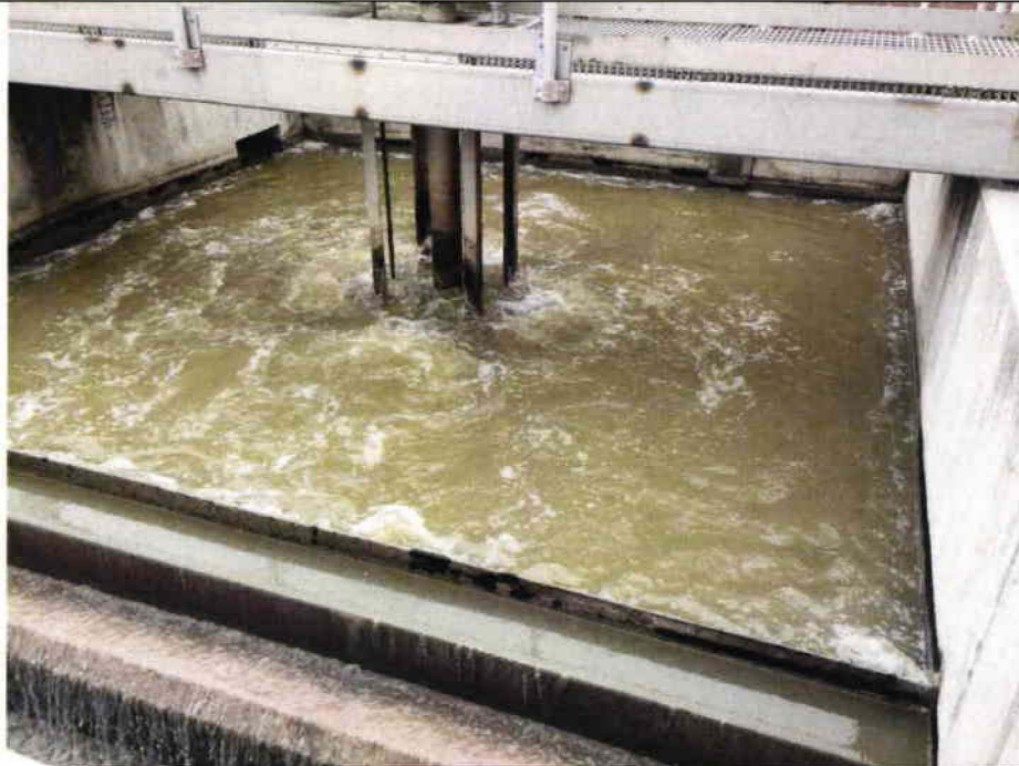
4 Aerated Grit Chamber at Headworks
