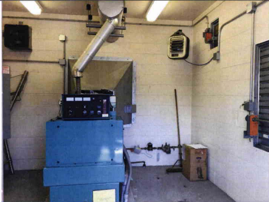
4 Pump Station #15 – Building Interior.
