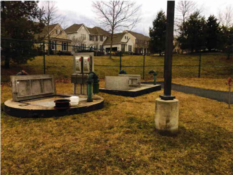
1 Pump Station #18 – Wet Well Exterior.
