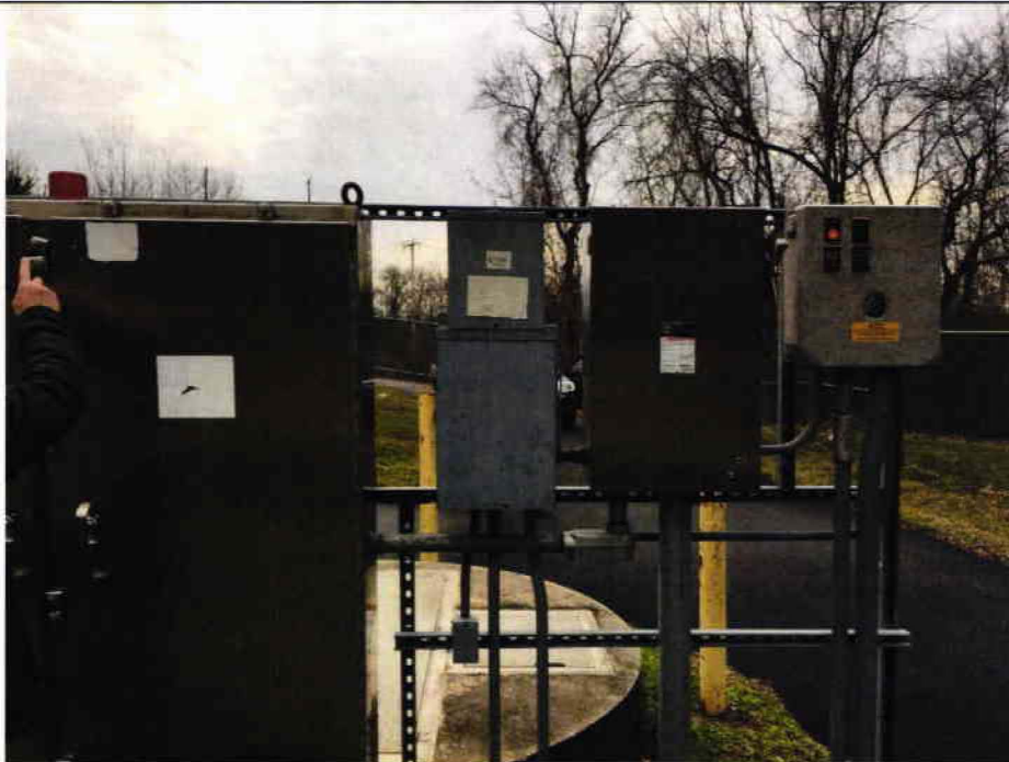
4 Pump Station #16 – Control Panel.
