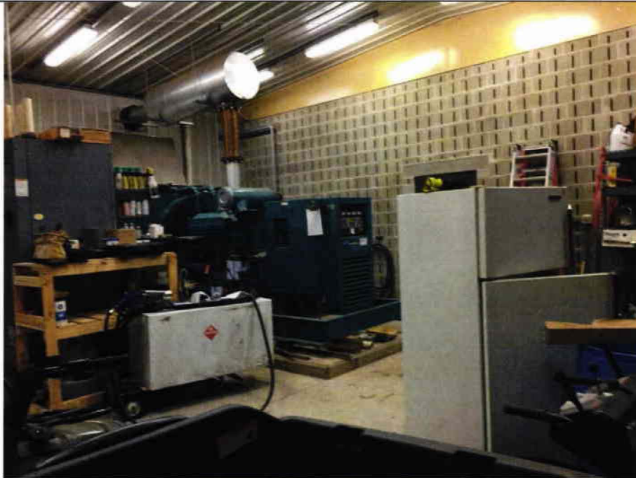
14 Possum Hollow WWTP- Facility Generator Room
