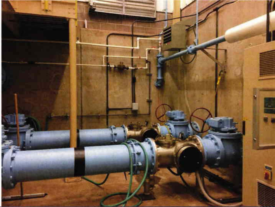
7 Possum Hollow WWTP- Inline UV Units
