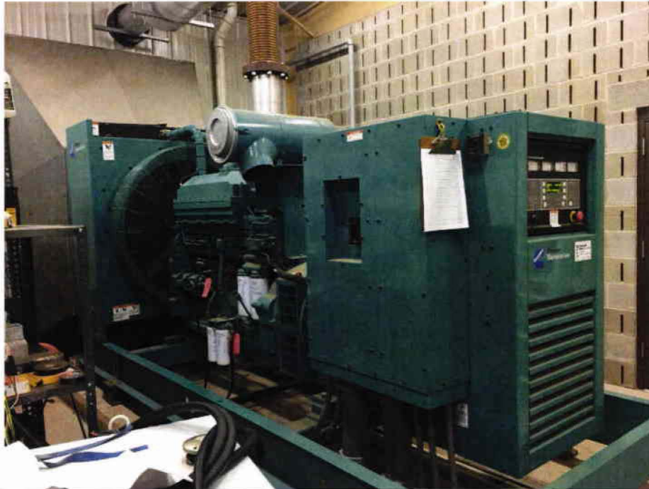
17 Possum Hollow WWTP- Generator
