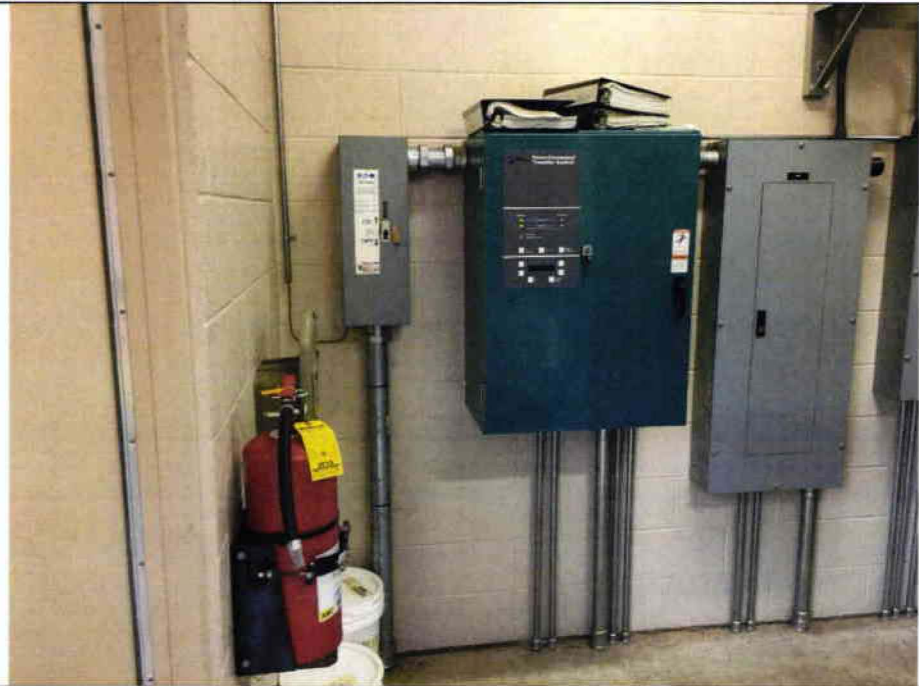
4 Pump Station #18 – Building Interior.
