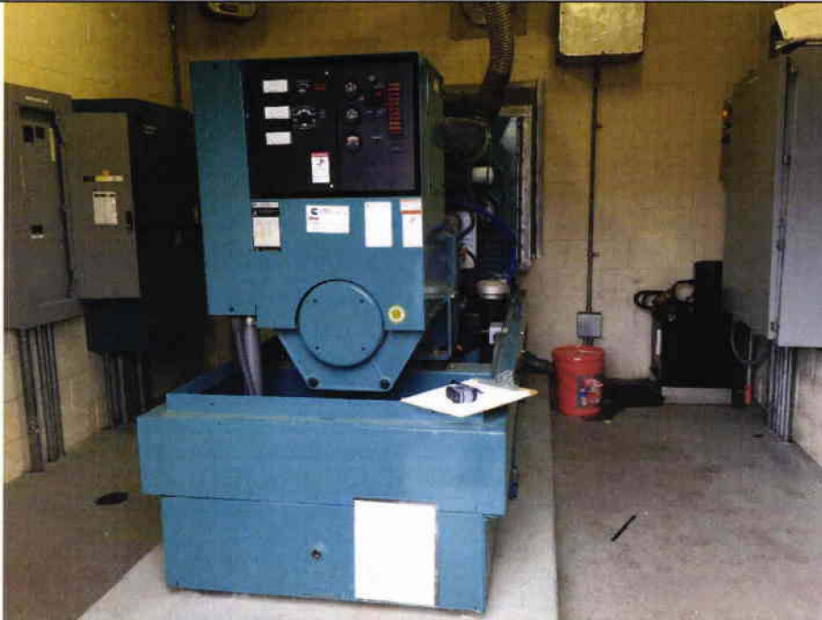
4 Pump Station #12 – Building Interior
