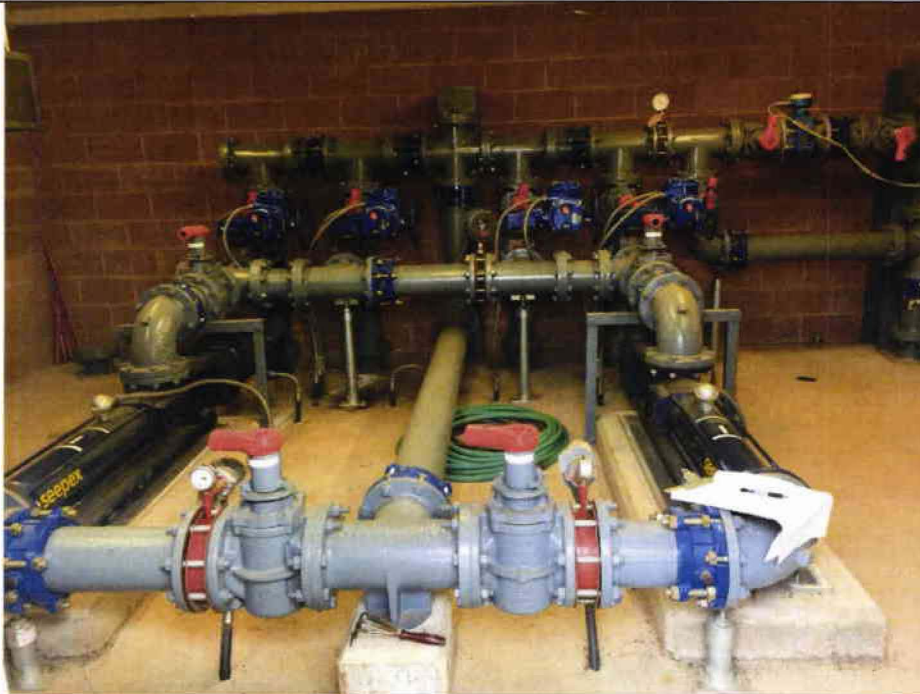
28 | WAS Sludge Pump Building Interior
