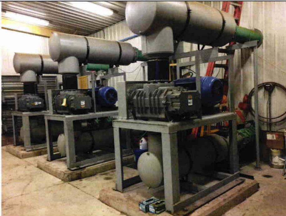
18 Possum Hollow WWTP- Blowers
