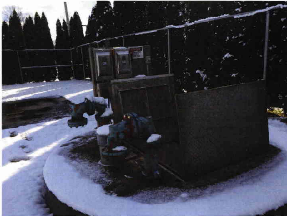
3 Pump Station #19 – Wet Well Exterior.
