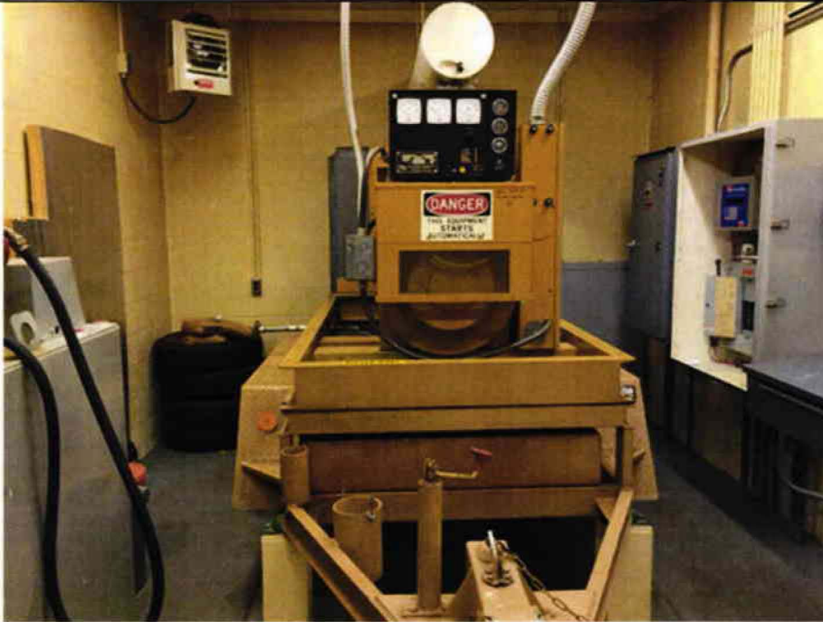
4 Pump Station #3 – Building Interior.
