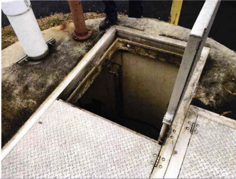
3 Pump Station #17 – Wet Well Exterior.
