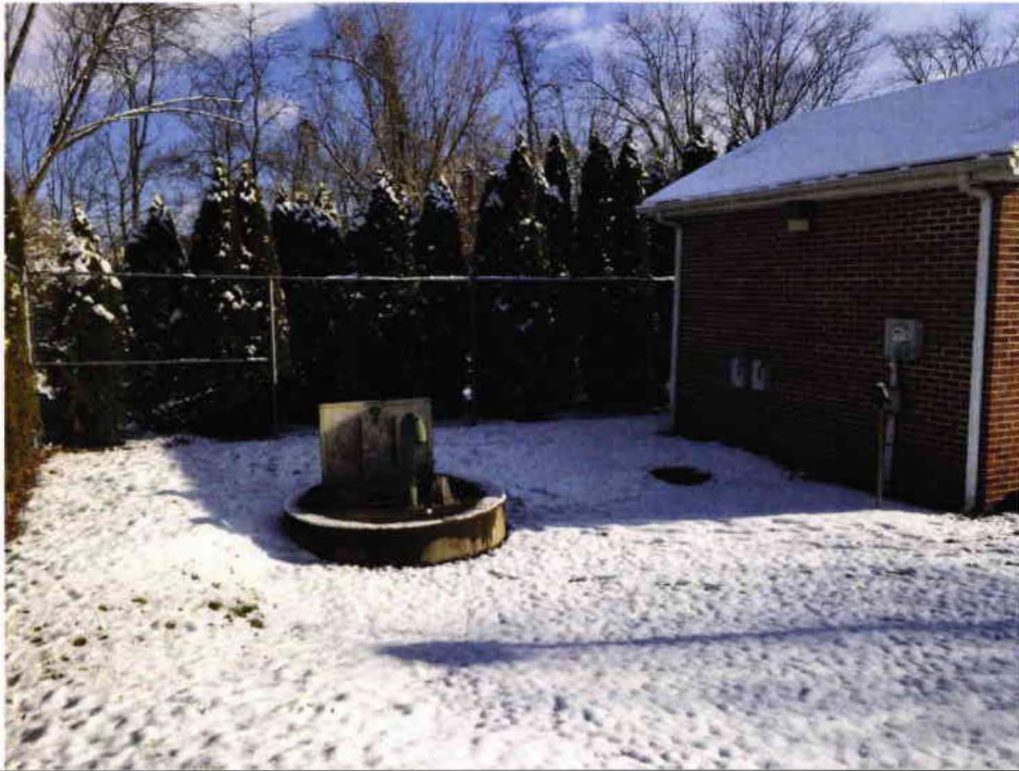
1 Pump Station #15 – Wet Well Exterior.
