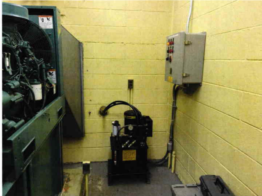
3 Pump Station #4 – Building Interior
