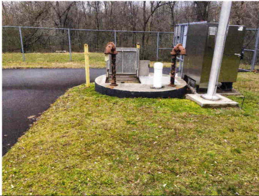
3 Pump Station #16 – Wet Well Exterior.
