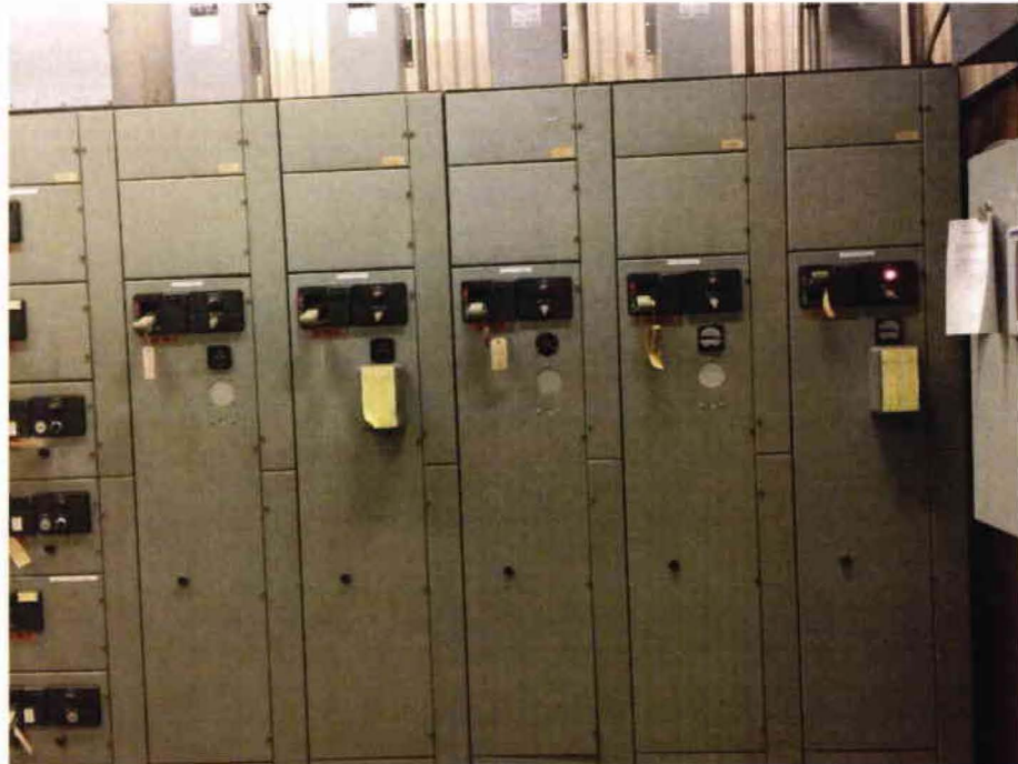
17 Blower MCC and Disconnect Switches
