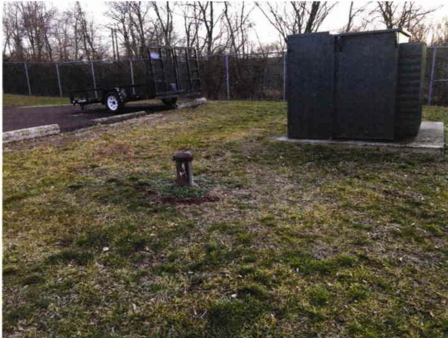
25 Possum Hollow WWTP- Yard Well Pump and PECO Transformer
