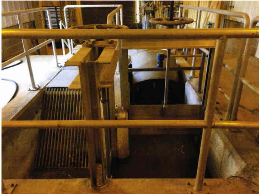
5 | Possum Hollow WWTP- Head Works Influent Screen Unit
