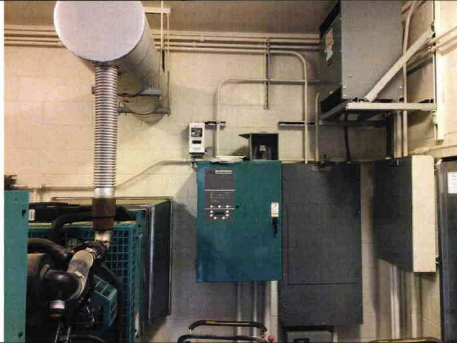
4 Pump Station #17 – Building Interior.
