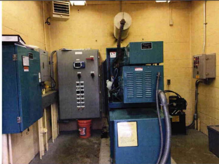
4 Pump Station #4 – Building Interior
