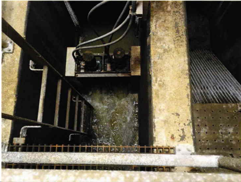
7 Pump Station #6 – Wet Well
