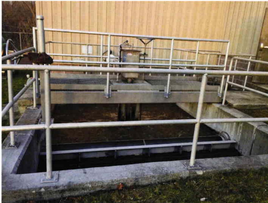
3 Possum Hollow WWTP- Aerated Grit Chamber
