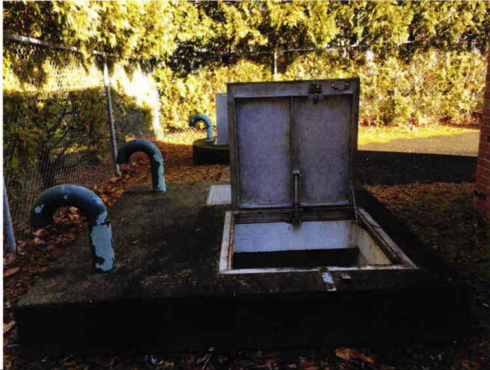
1 Pump Station #13 – Wet Well Exterior.
