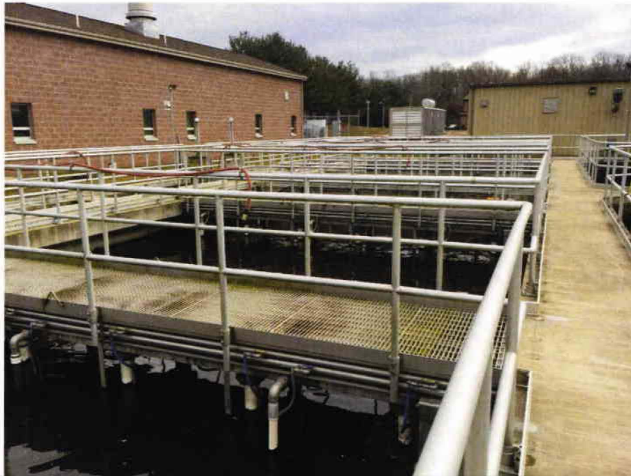
23 SBR Treatment Chambers
