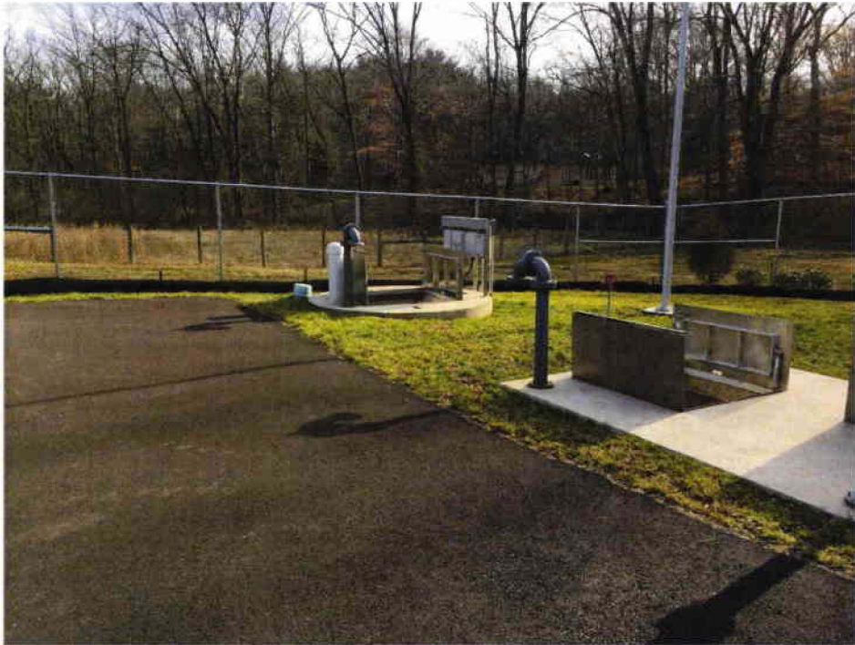
1 Pump Station #20 – Wet Well Exterior.
