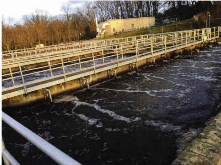
21 Possum Hollow WWTP- SBR Unit Aeration Chamber
