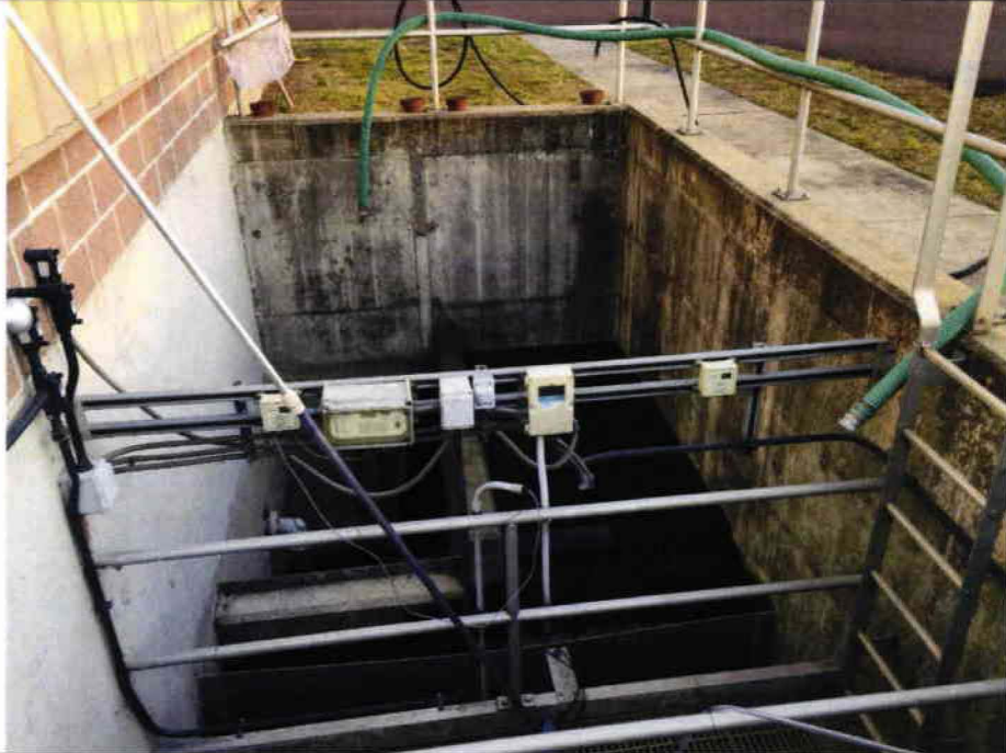
24 | Possum Hollow WWTP- Discharge Chamber
