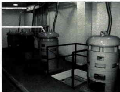
W.W.T.P. PUMP STATION (DRY WELL) FLOOR EL. 718.59 DEMOLITION PHOTOGRAPH PS6-G REFERENCE PLAN PS3-A
