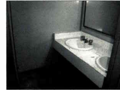
TICO BUILDING STORAGE ROOM WOMENS ROOM DEMOLITION PHOTOGRAPH TB4-J REFERENCE PLAN TB2-A
