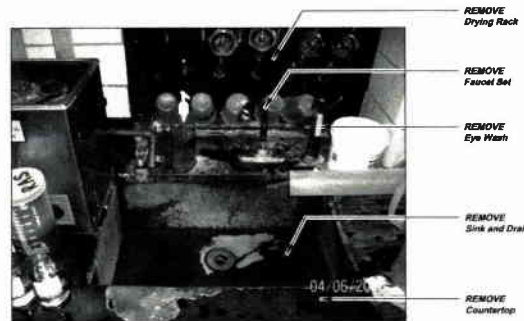
INTERIOR LABORATORY (BASE CABINET EAST WALL) DEMOLITION PHOTOGRAPH LA3-G REFERENCE PLAN LA1-A
