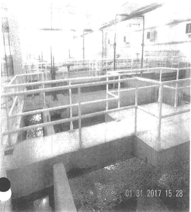
Duquesne Sewage Treatment Plant
