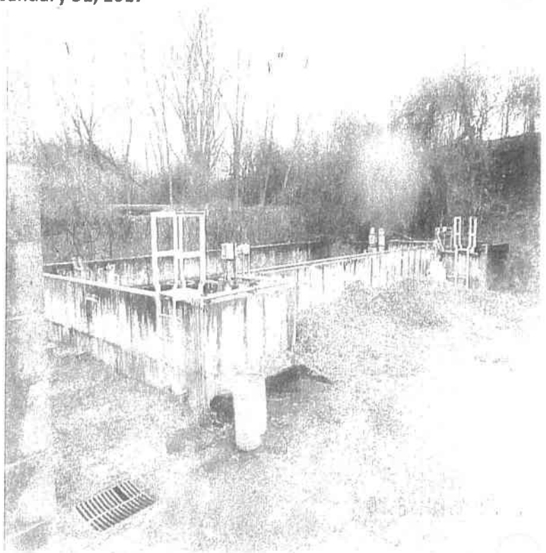
DSTP – Sludge Tank
