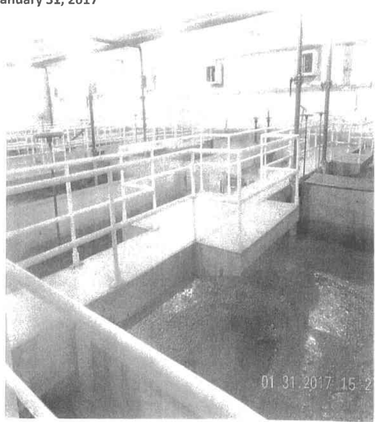
Duquesne Sewage Treatment Plant
