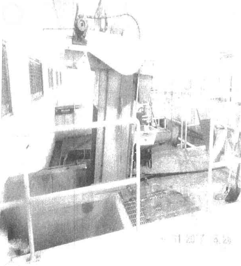
Duquesne Sewage Treatment Plant
