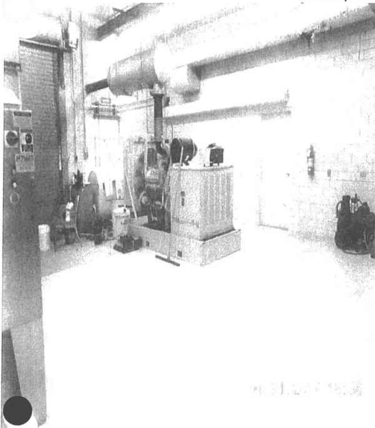
DSTP – Emergency Generator
