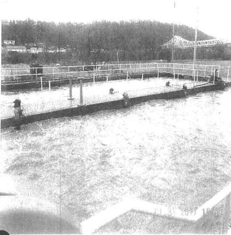
Dravosbury Treatment Plant
