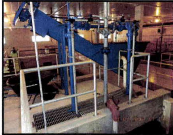
Grit Removal System Photograph 6.2
