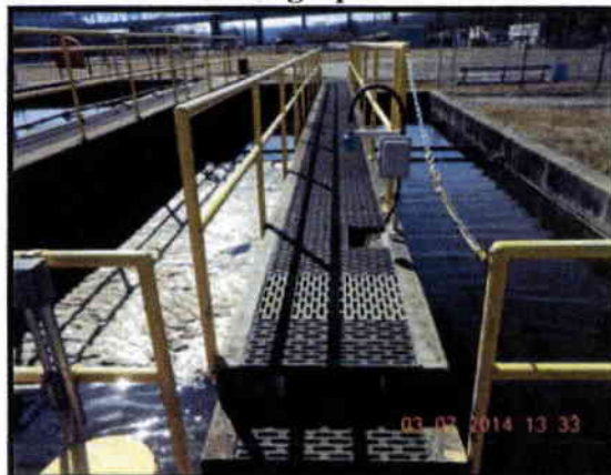
Final Clarifiers Photograph 6.3
