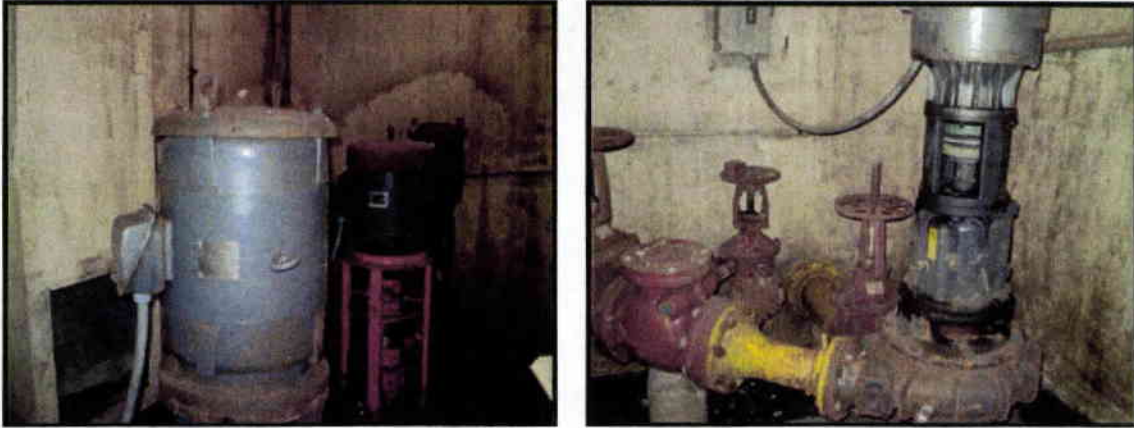
Raw Sewage Pumps Photograph 6.2
