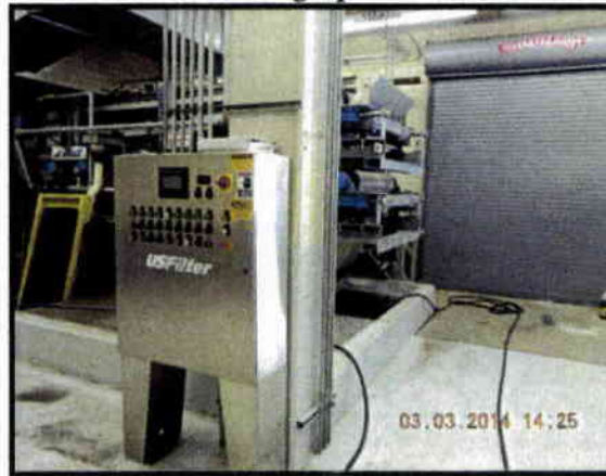
Belt Filter Press Photograph 6.6
