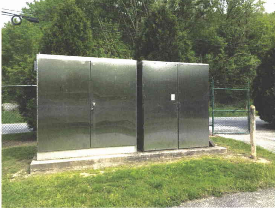
Pump Control Panels
