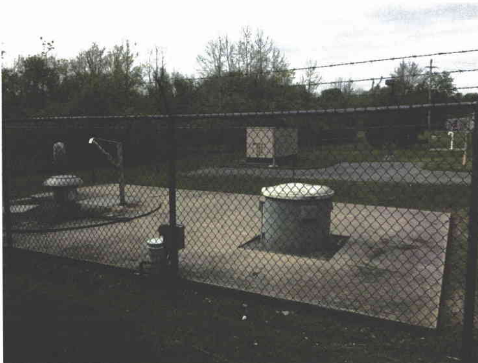
Wet Well and Valve Pit
