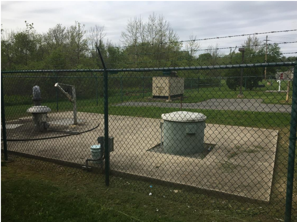
Wet Well and Valve Pit
