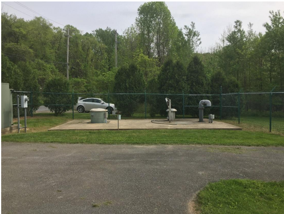
Valve Pit and Wet Well
