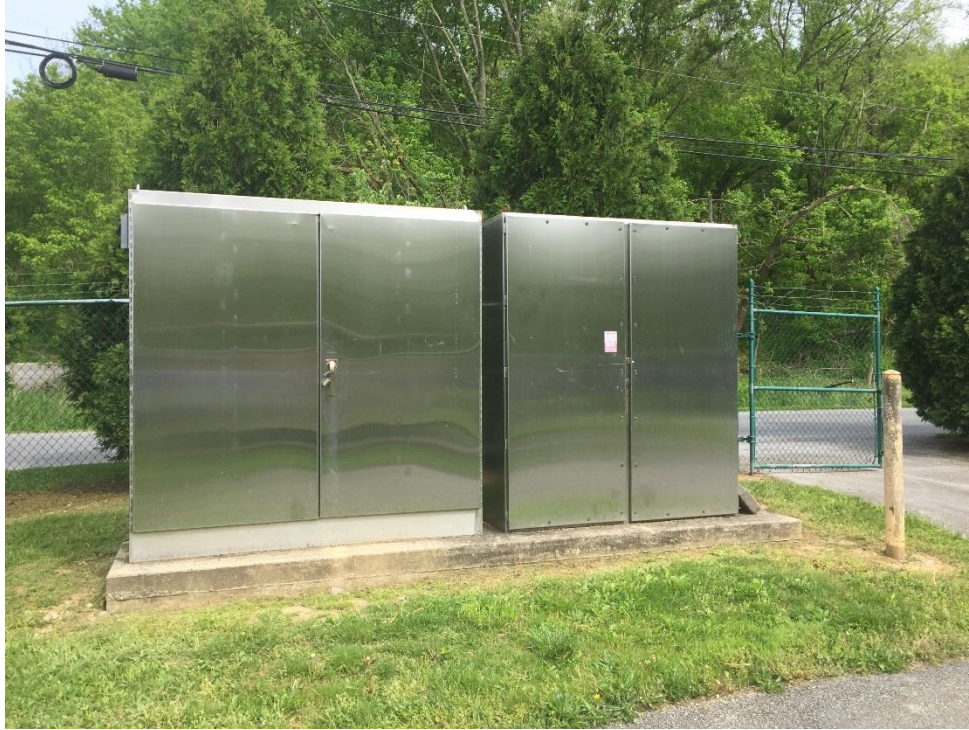
Pump Control Panels
