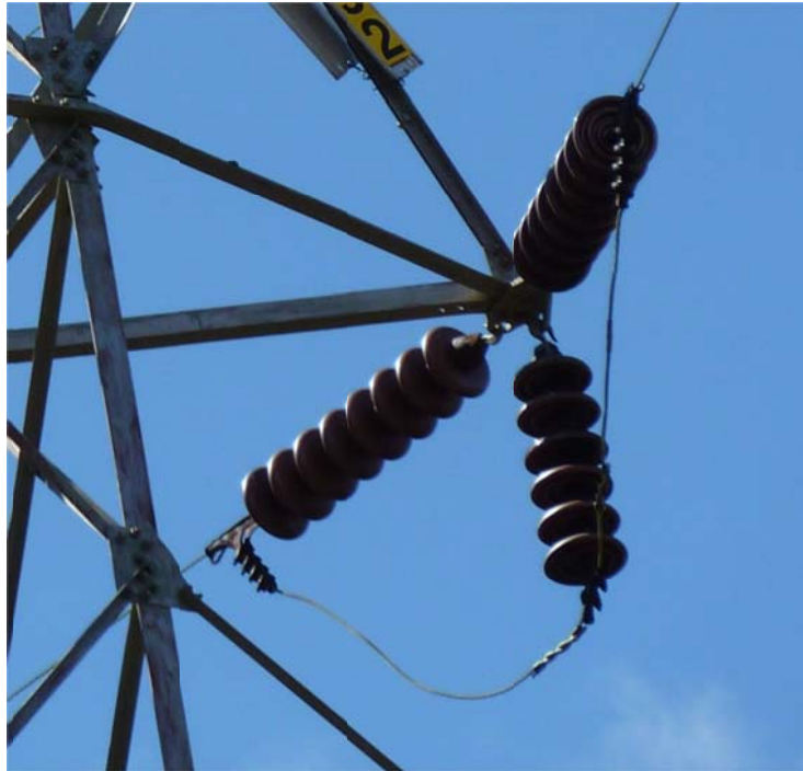
Photo 7 – Heavy corrosion typical strain insulator string on lattice tower
