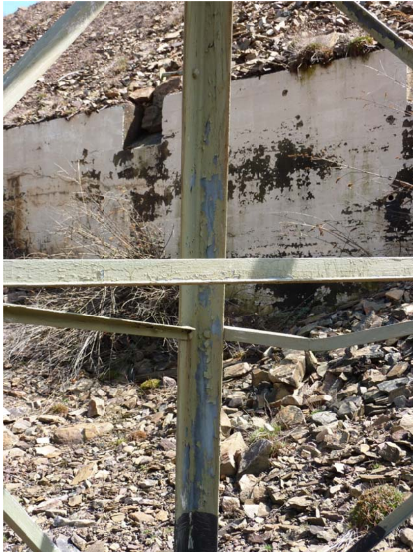
Photo 8 – Fair paint conditions, only peeling at bottom of tower
