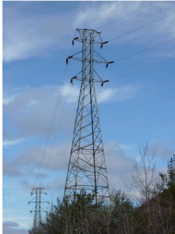
Photo 2 – Typical steel lattice tower
