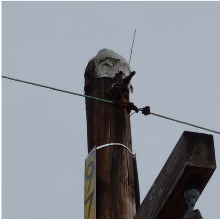
Photo 4 – Typical Shield Wire Saddle Clamp Connection (hardware corroded)
