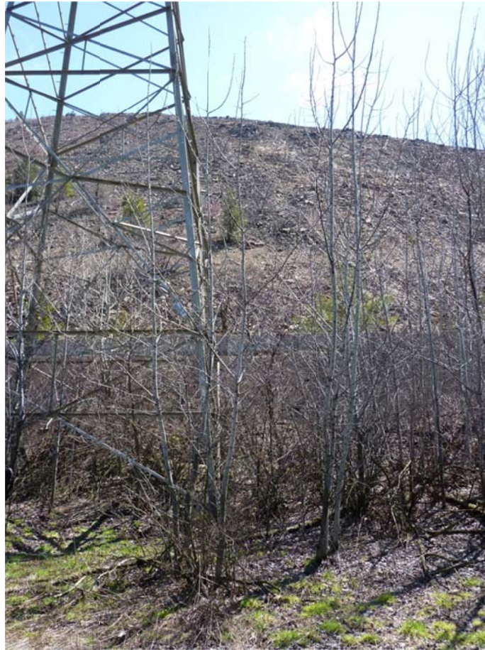
Photo 10 – Poor vegetation conditions (Structure Inspection No. 70)
