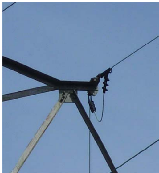
Photo 5 – Typical Shield Wire Strain Clamp Connection (jumped but not bonded to tower and hardware very corroded)
