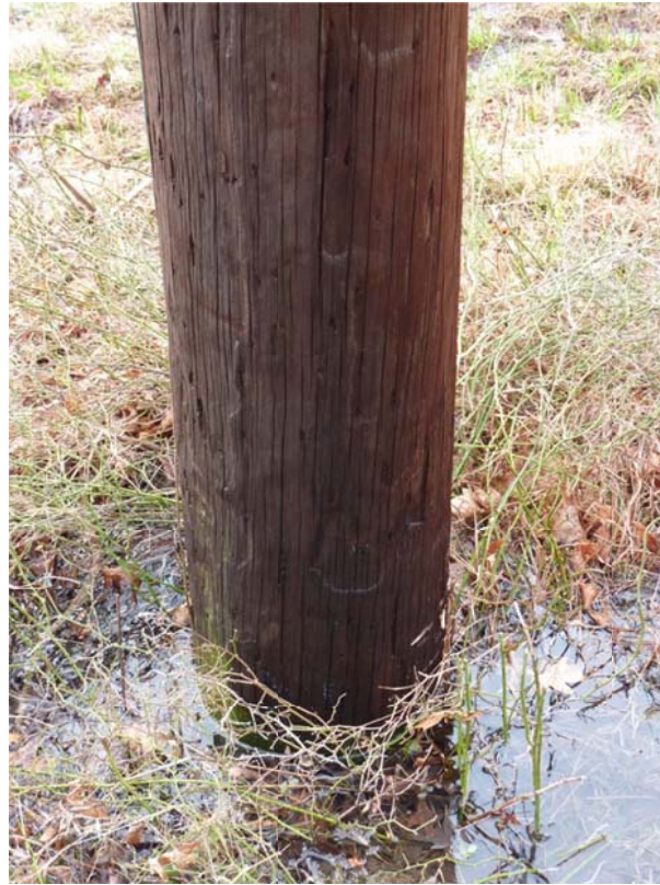
Photo 3 –Typical wood pole located in standing water
