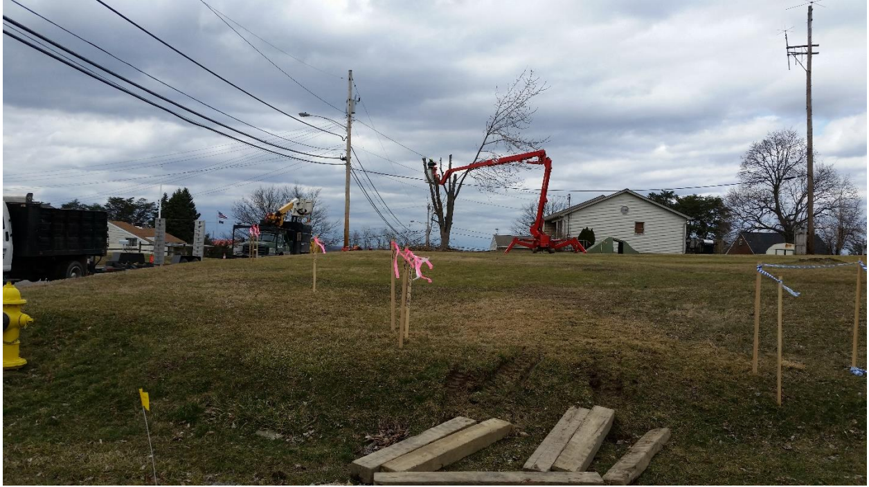
Zimmerman Drive, Aliquippa, PA. National Fuel cut down the tree in the front yard. The pipeline will be installed where the tree used to be, roughly 30 feet from the front door. Would you buy this house?
