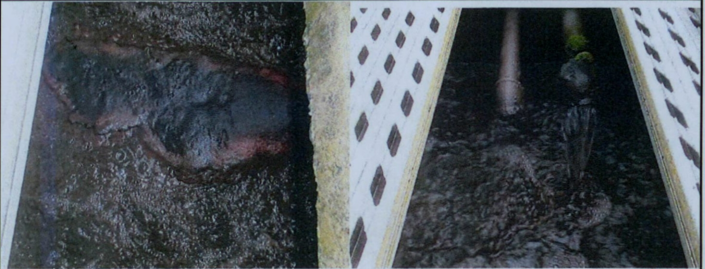
Image 1: Photo taken by Michael Benham on 6/21/2018. Shows solids accumulation in first aeration tank.
