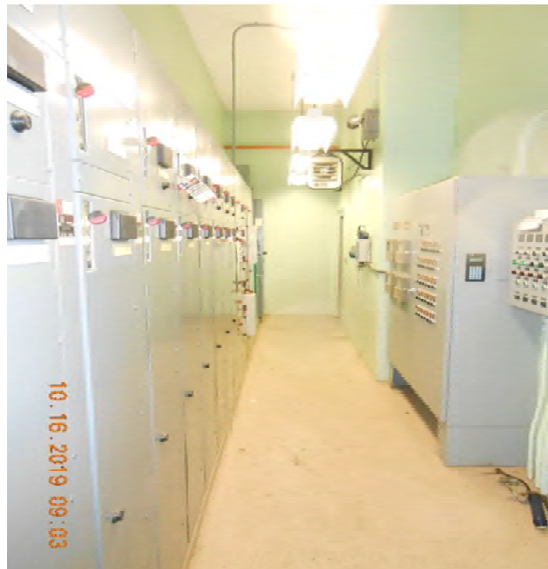
Kinzua WWTP - Pump Control Room
