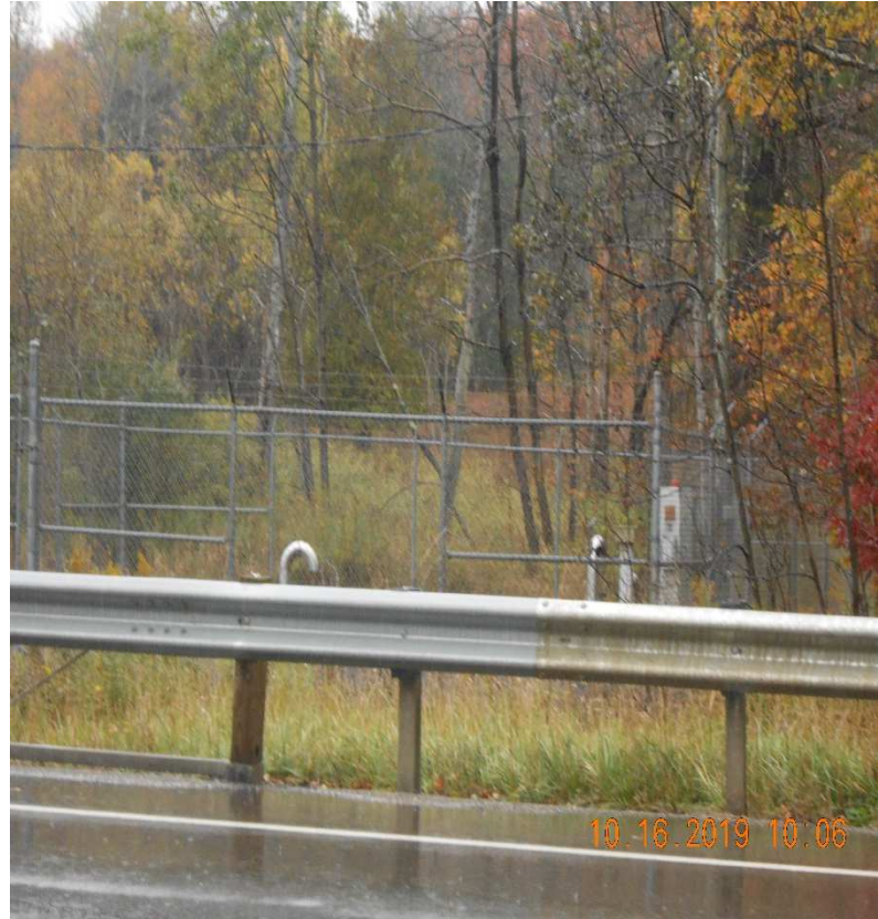
Rt. 66 Pump Station Flows to Pine St. WWTP
