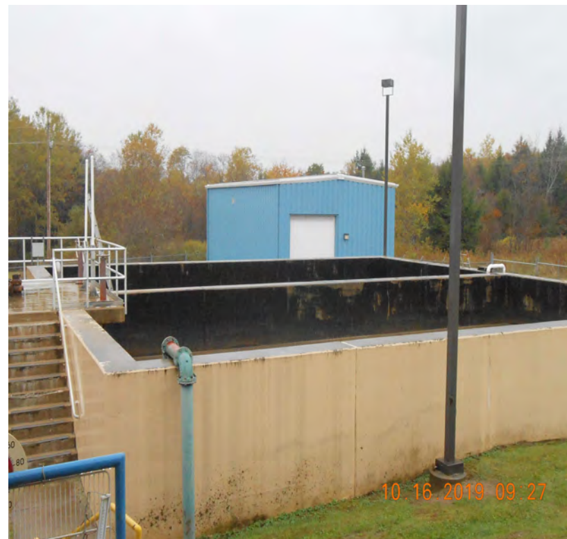
Pine St. WWTP – Digesters
