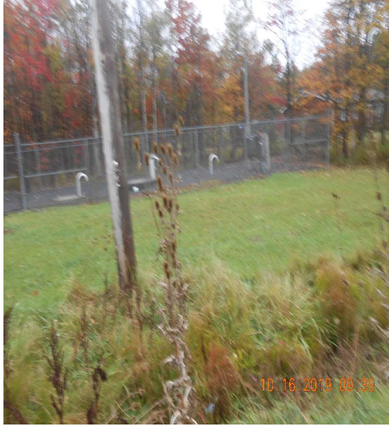
Rt. 6 Pump Station Flows to Pine St. WWTP
