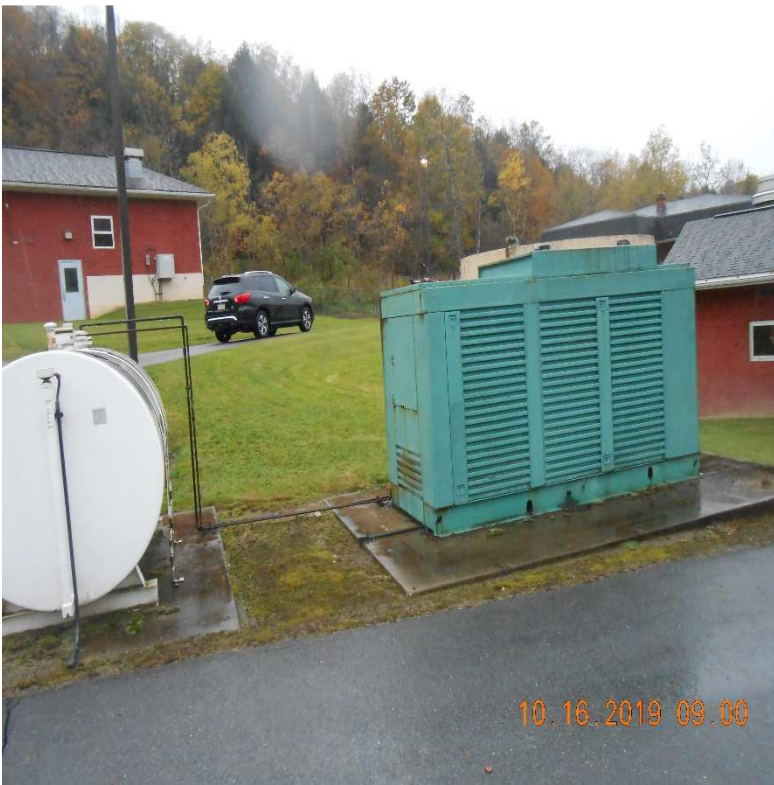
Kinzua-WWTP - Back-up Power
