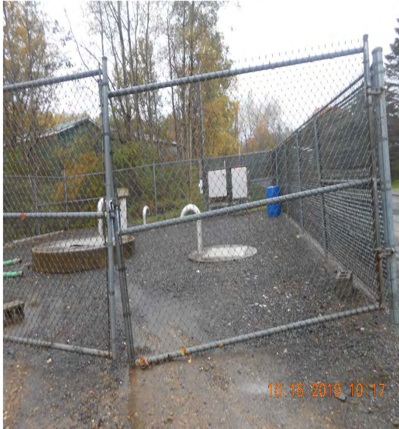
Pond St. Pump Station Flows to Kinzua WWTP
