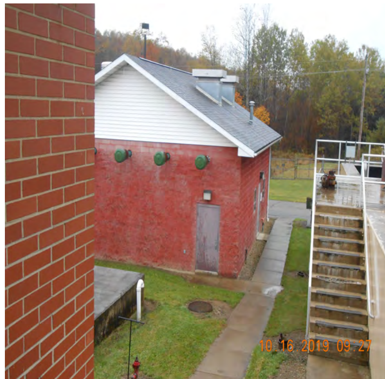
Pine St. WWTP – Blower Building
