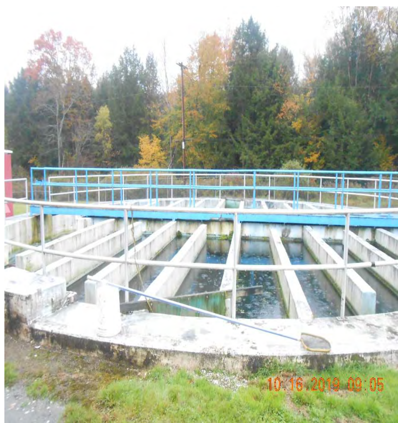
Kinzua WWTP - Chlorine Contact Tank
