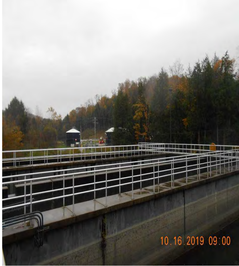
Kinzua WWTP SBR – Treatment
