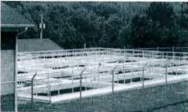
600,000 GPD (peak capacity of 2MGD) stream discharge Hastings Area Sewer Authority, Cambria County, PA
