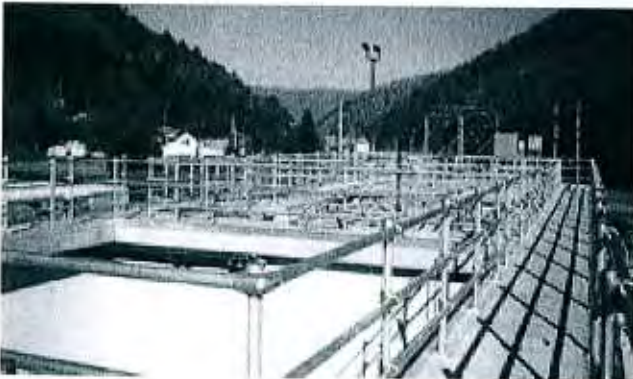
67,000 GPD, lagoon discharge Eaglesmere, Sullivan County, PA
