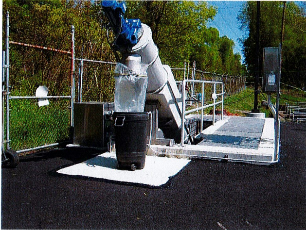
Figure 17 – Influent Screen Unit (Upper Grinder Station)
