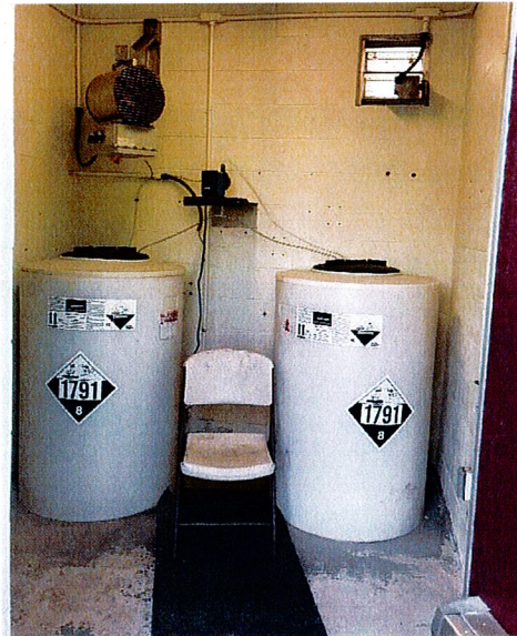
Figure 8 – Chlorine Storage and dosing room
