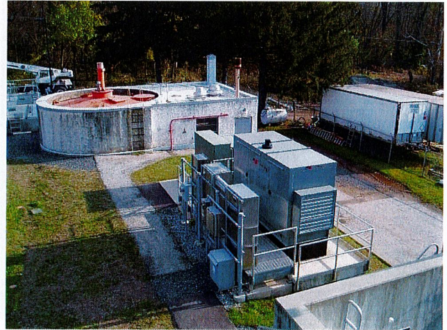
Figure 2 – Emergency Generator and Sludge Digester
