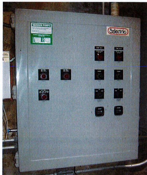
Figure 8 – Pump Control Panel (now located on deck)
