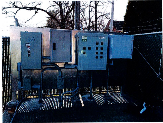
Figure 2 – Pump Control Panels
