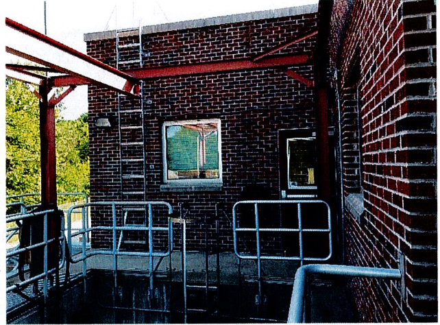
Figure 6 – Office entrance and wetwell
