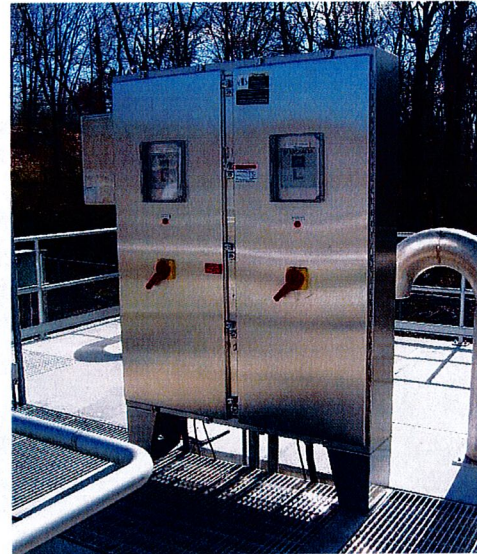
Figure 14 – Secondary Recirculation Pump Station VFDs
