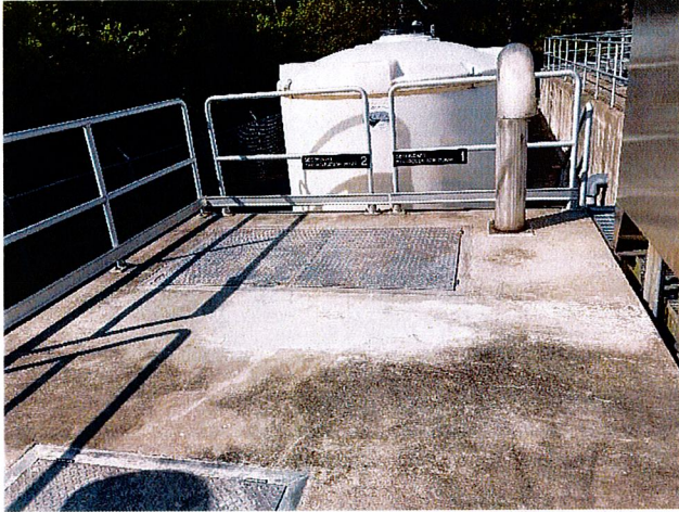
Figure 13 –Secondary Recirculation Pump Station
