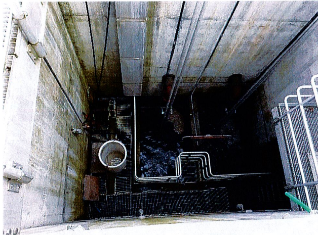
Figure 7 – Raw Sewage Pumps
