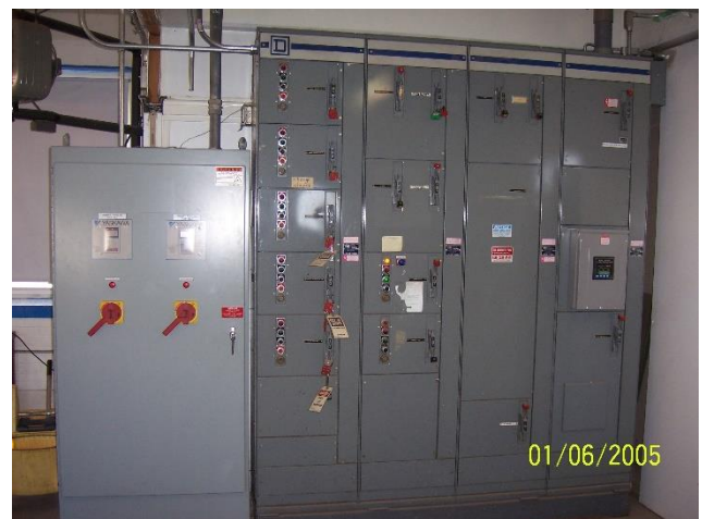
Figure 16 – Primary Recirculation Pumps VFDs and MCC in Lab Building
