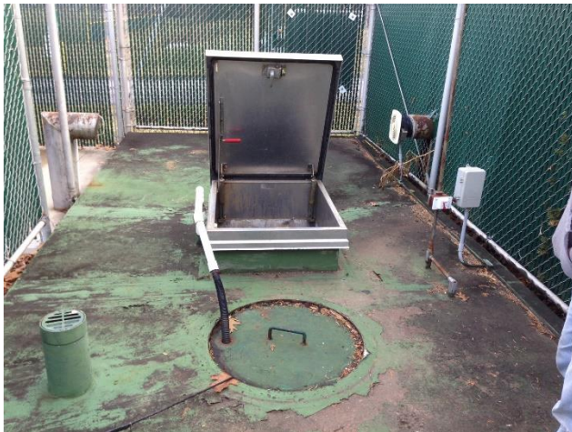
Figure 3 – Dry Pit Entry Hatchway
