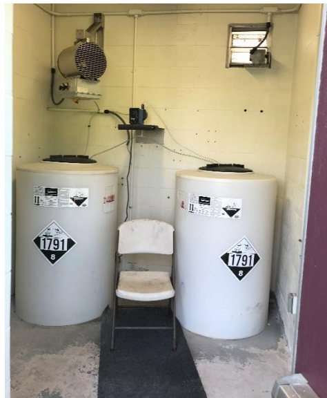
Figure 8 – Chlorine Storage and dosing room
