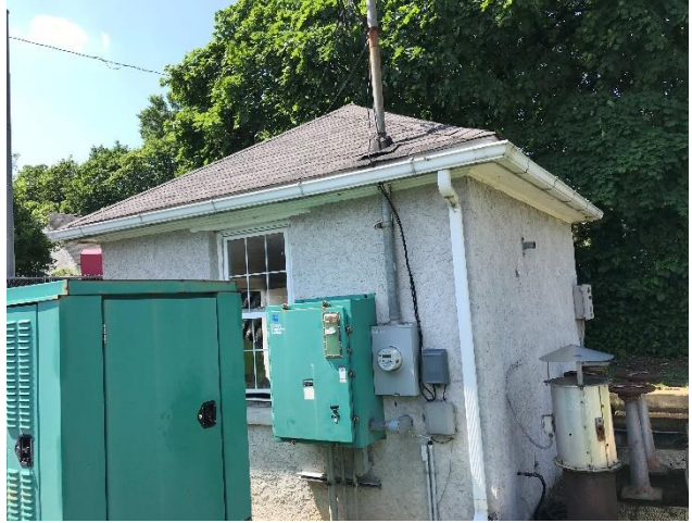
Figure 2 – Building, Generator and ATS
