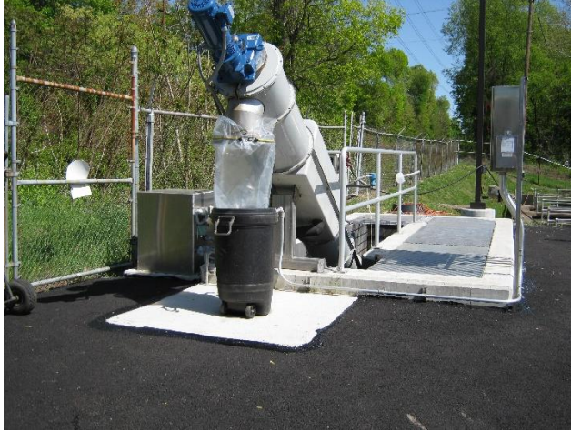
Figure 17 – Influent Screen Unit (Upper Grinder Station)
