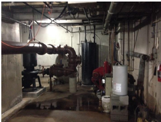
Figure 15 – Lab Building. Basement – Primary Recirculation pump and Sludge Transfer Pump
