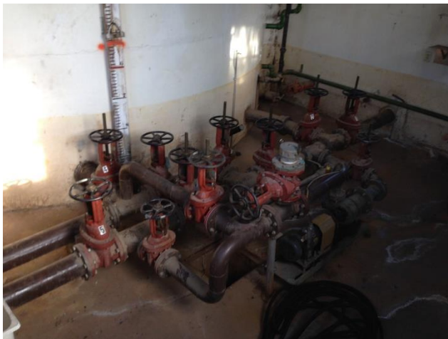
Figure 19 – Digester Building Control Room
