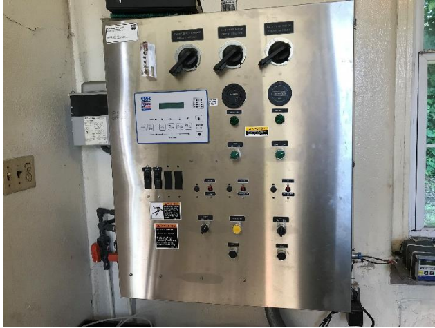
Figure 5 – Pump Control Panel
