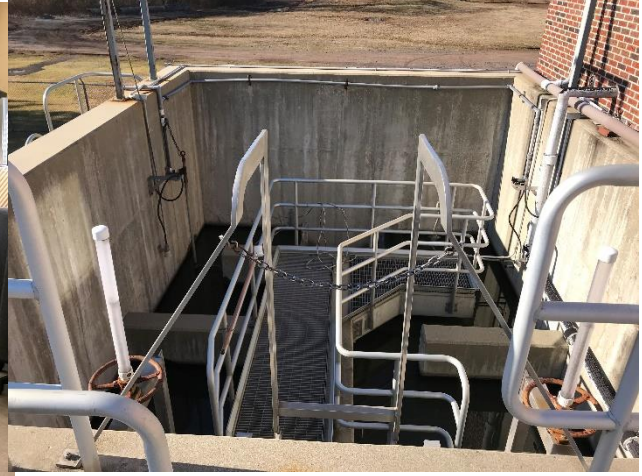
Figure 10 – Chlorine Contact Basin
