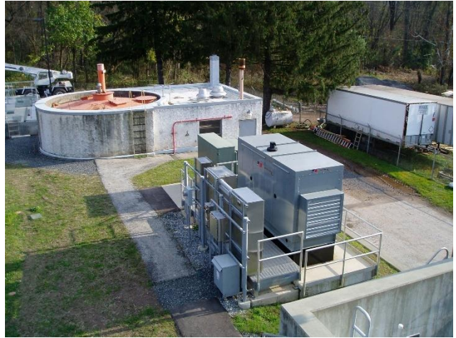
Figure 2 – Emergency Generator and Sludge Digester
