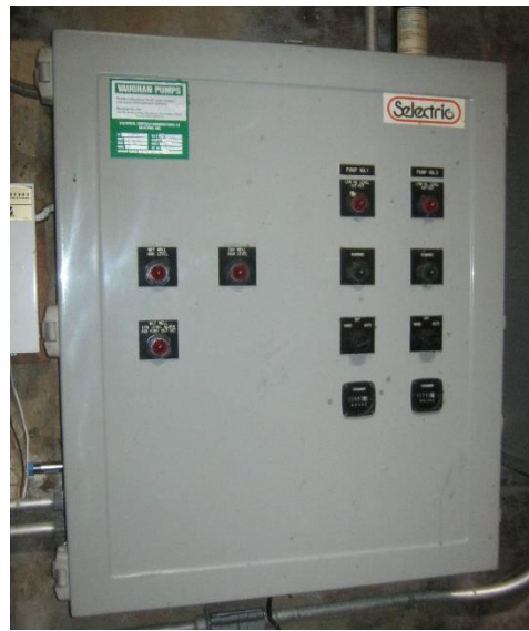
Figure 8 – Pump Control Panel (now located on deck)
