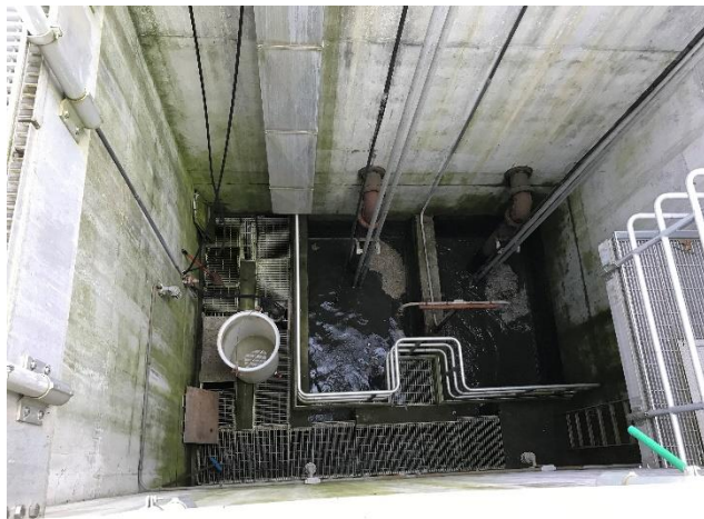
Figure 7 – Raw Sewage Pumps
