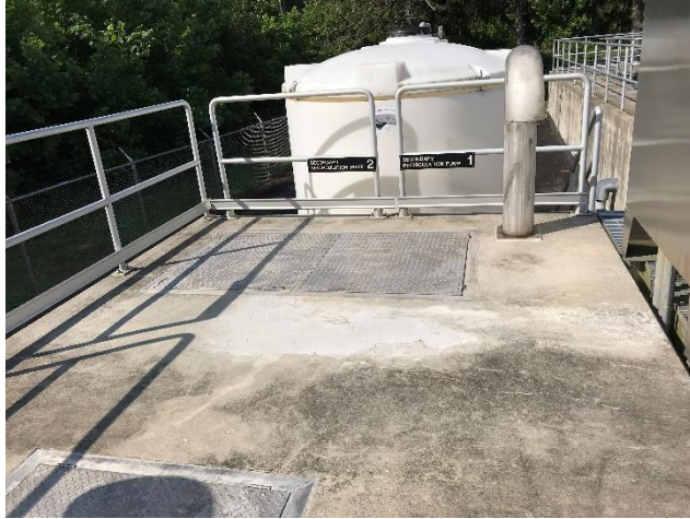
Figure 13 –Secondary Recirculation Pump Station
