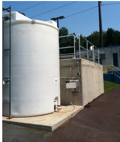
Figure 12 – PAC storage and Dosing System
