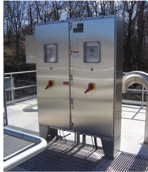
Figure 14 – Secondary Recirculation Pump Station VFDs
