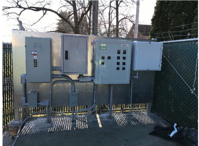
Figure 2 – Pump Control Panels
