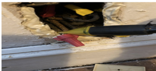
Figure 1 Gelson tested wires attached to the receptacle apt #3. They had no power
