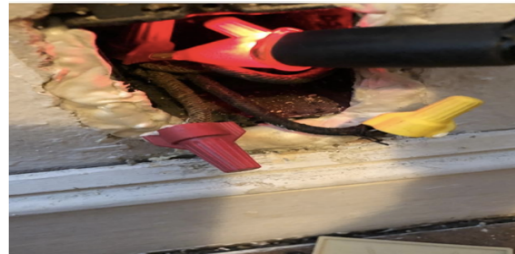
Figure 2 Gelson tested wires and showed power. Those were the two extra wires left behind the receptacle that had power connected to apt #1.
