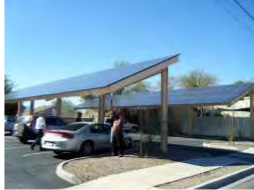
An example of solar panels installed over a parking area
