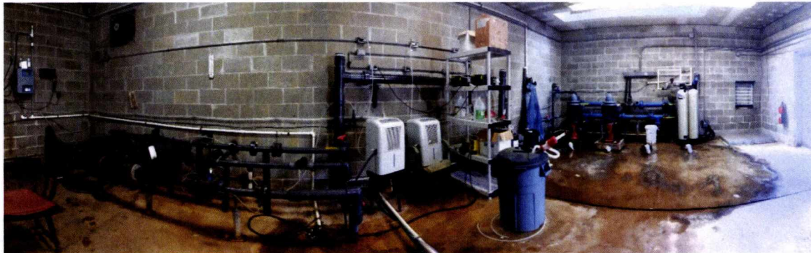
Figure 8 – WTP, internal piping
