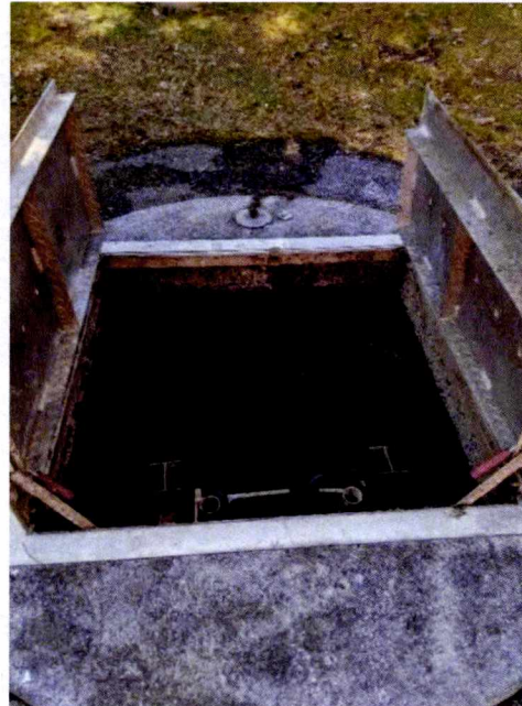
Figure 2 – Wet Well Interior with Trash Rack
