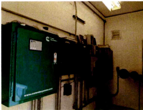
Figure 3 – Control Panel & Electrical
