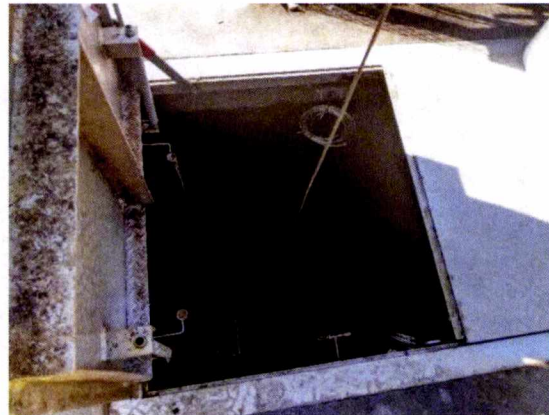
Figure 2 – Wet Well Interior
