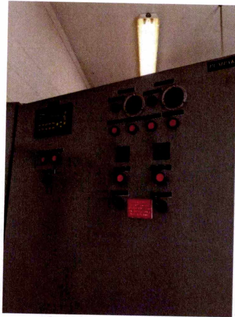
Figure 2 – Pump Control Panel
