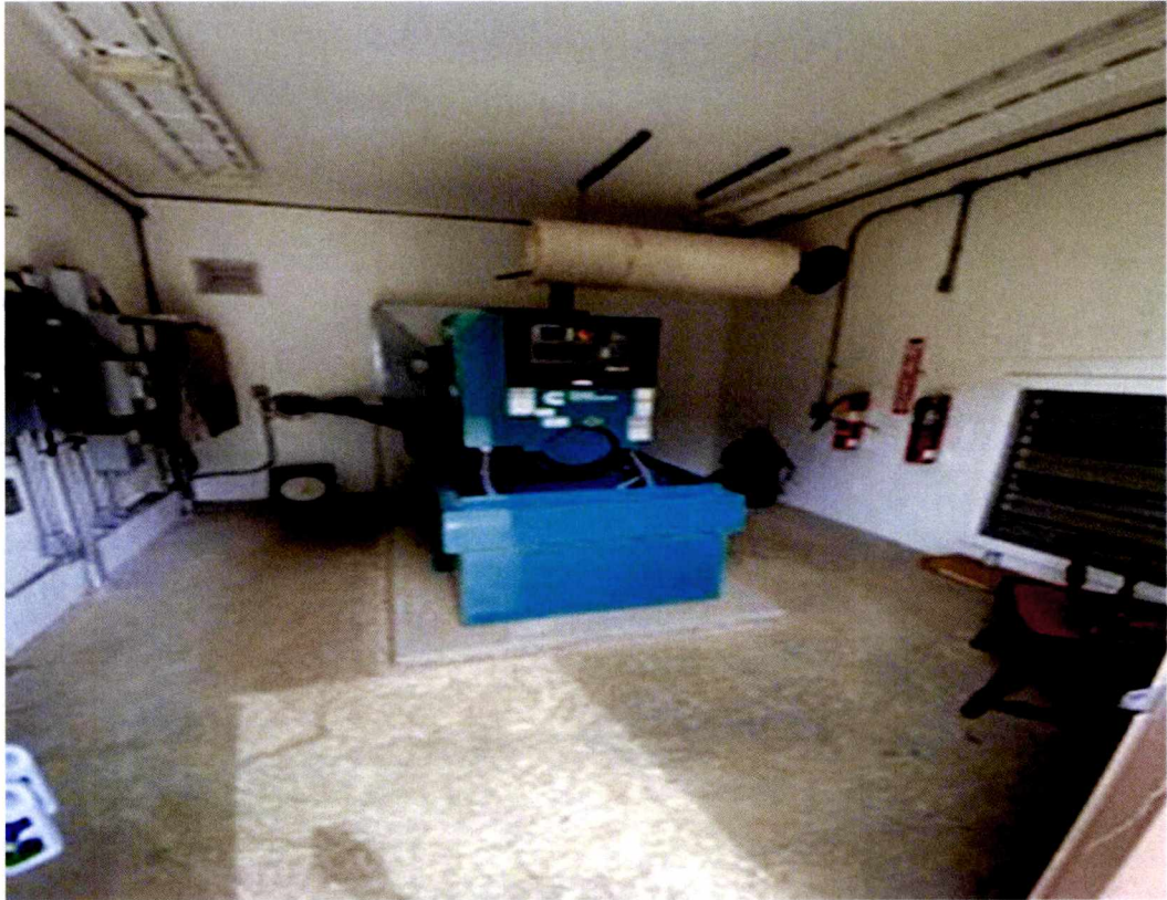
Round Hill #1 Sewer Pump House
