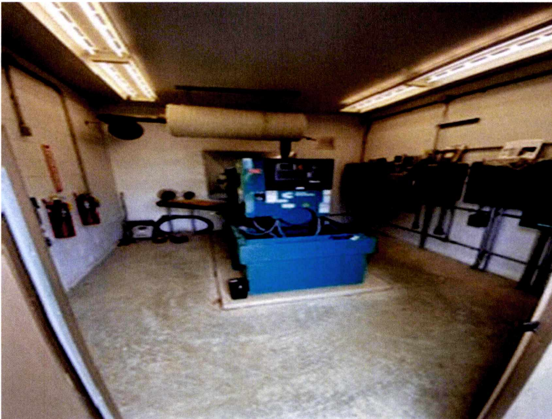
Round Hill #2 Sewer Pump Station
