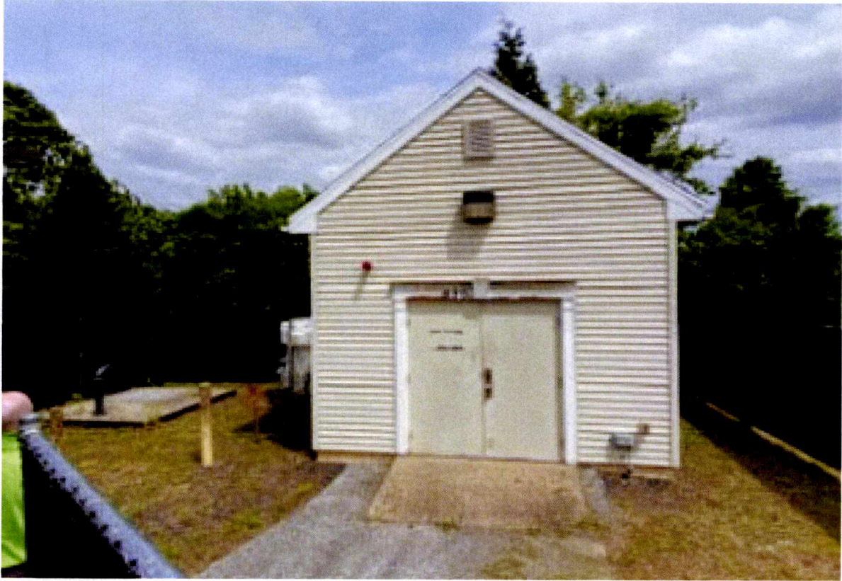
Hill View Sewer Pump Station
