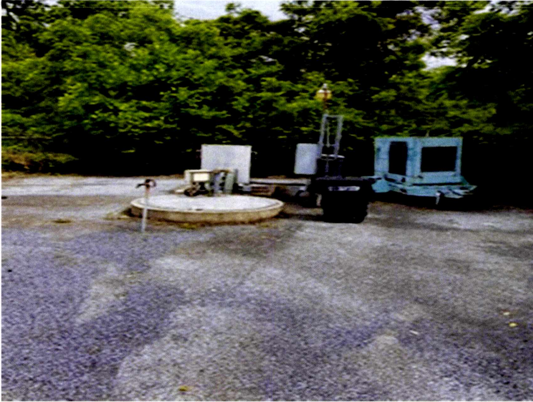
Highland Corporate Center Sewer Pump Station
