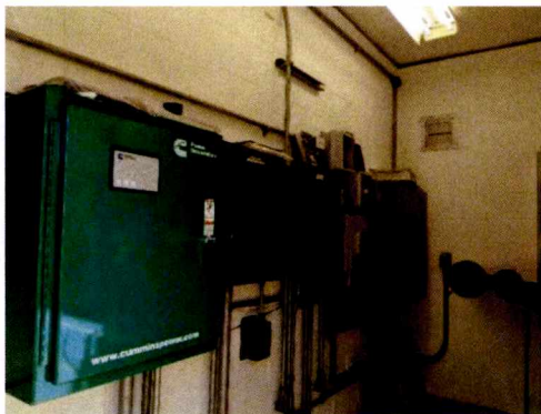
Figure 3 – Control Panel & Electrical
