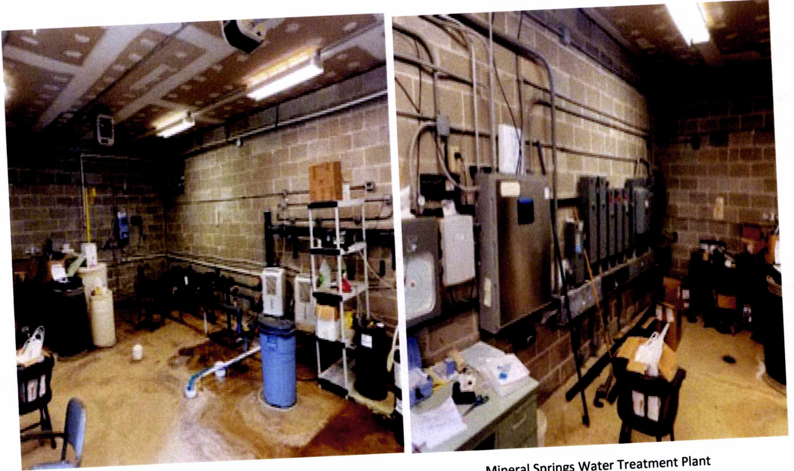
Mineral Springs Water Treatment Plant
