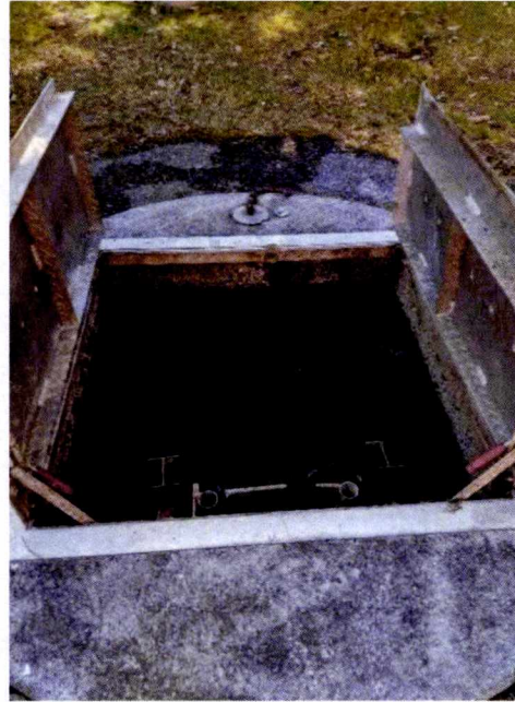
Figure 2 – Wet Well Interior with Trash Rack
