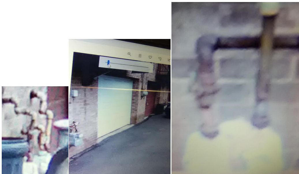
CONDITION OF THE GAS LINE PIPES DURING THIS COMPLAINT 2012 UP TO 1/22/2020.
