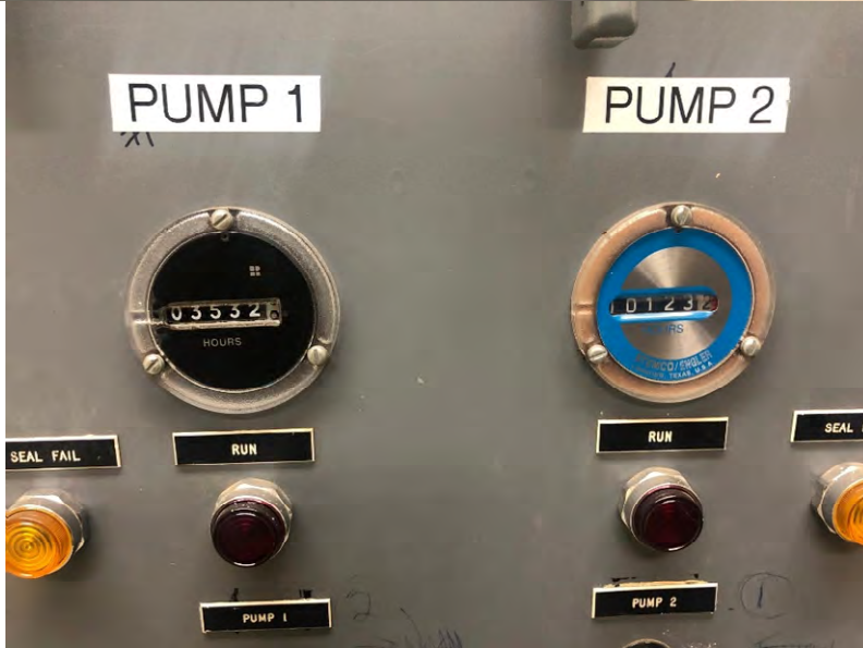
Duplex Pump Control Panel
