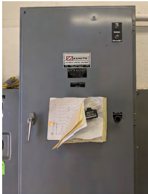
Automatic Transfer Switch
