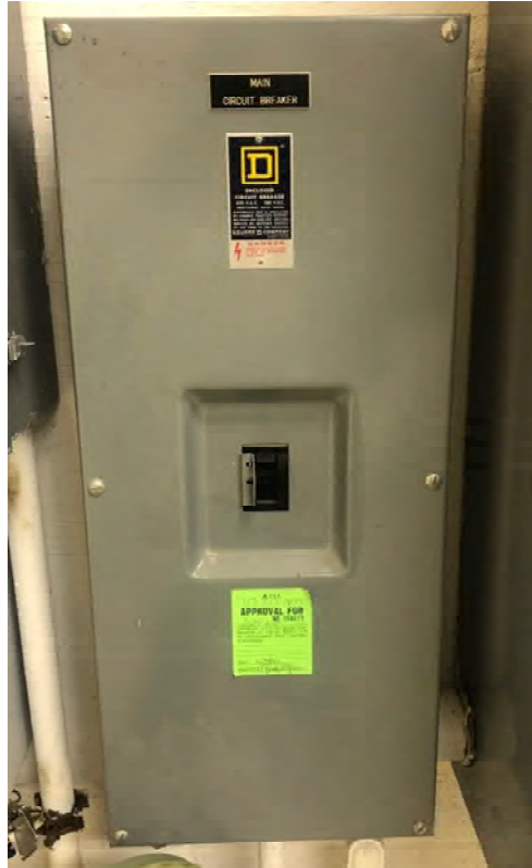
Main Circuit Breaker
