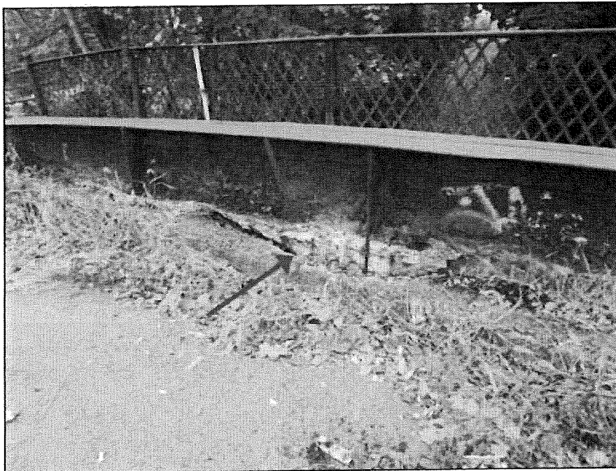
Visible settlement along the right curb at the far end.
