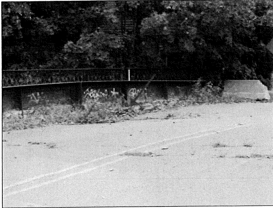
View of the top side right floorbeam and girder 2 failed connection. (visible deck settlement at midspan)
