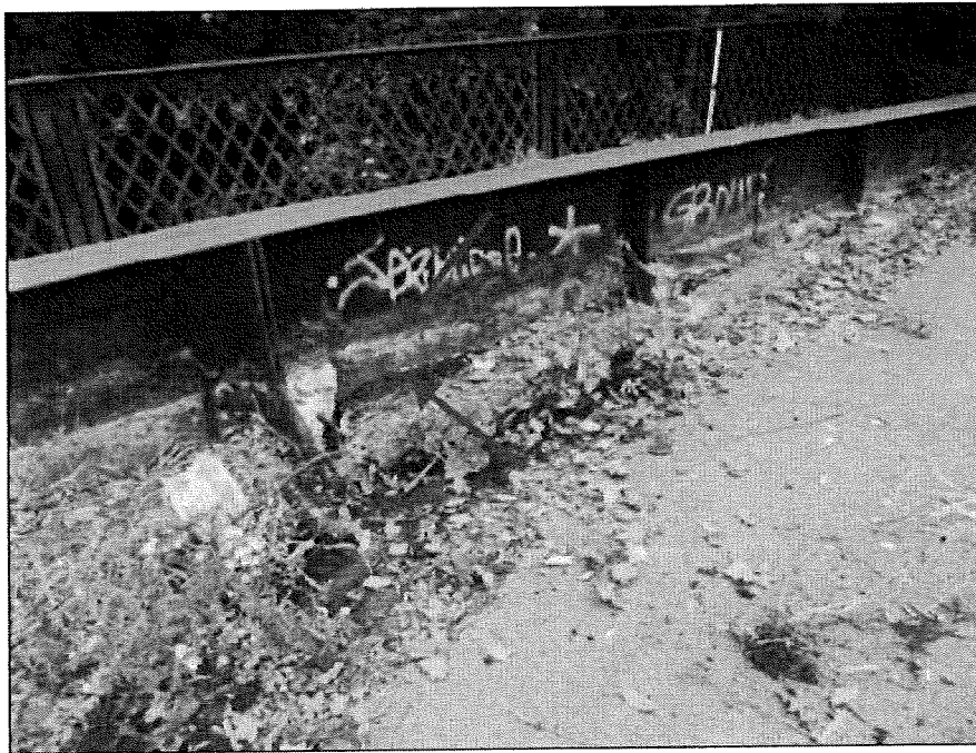
Visible 5" deck settlement along the right curb at midspan.
