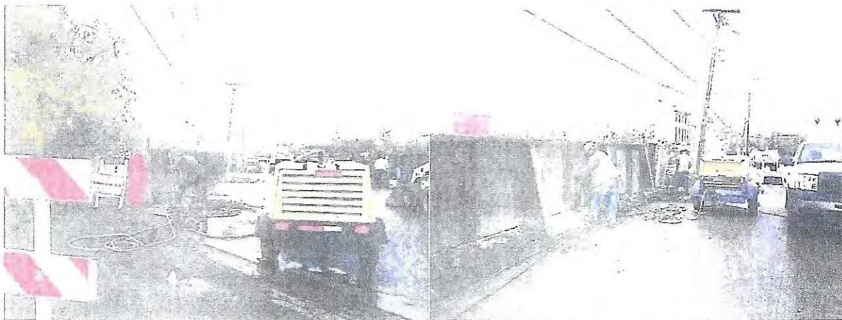
1. Laborers working without proper PPE
