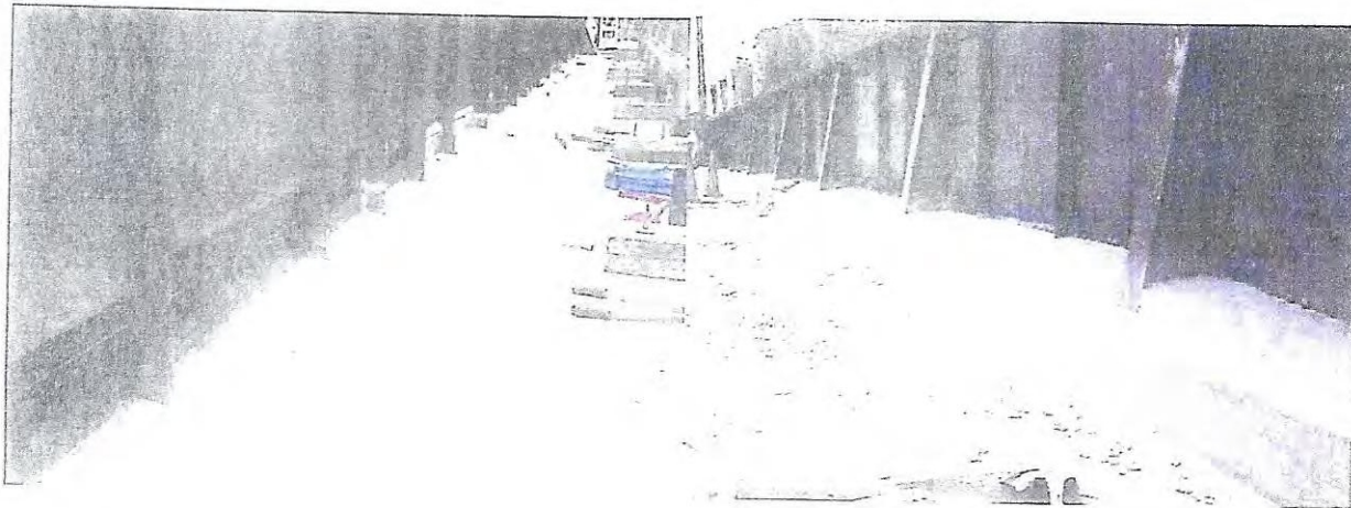
3. S. through girder - conc. sidewalk installation 4. S. through girder - conc. curb installation
