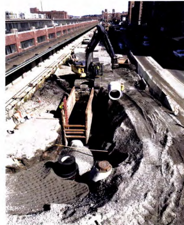
Smallman Street Sewer
