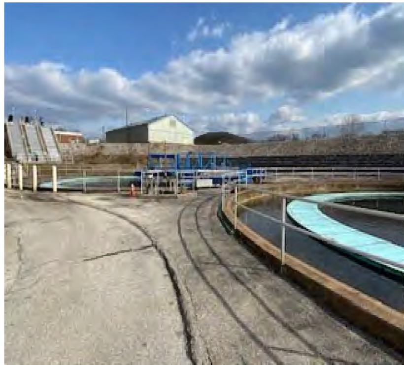
Clarifier for train 2
