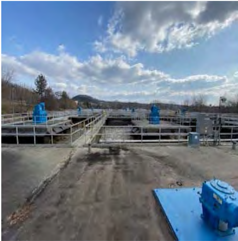
A/O Tanks train 3
