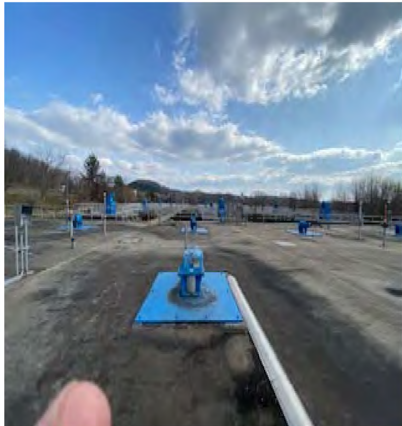
A/O Tanks train 3
