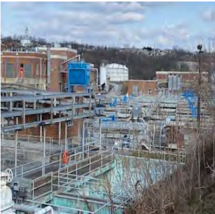
A/O Tanks – Train (2) approximately 16 million Incinerator daily flow processed
