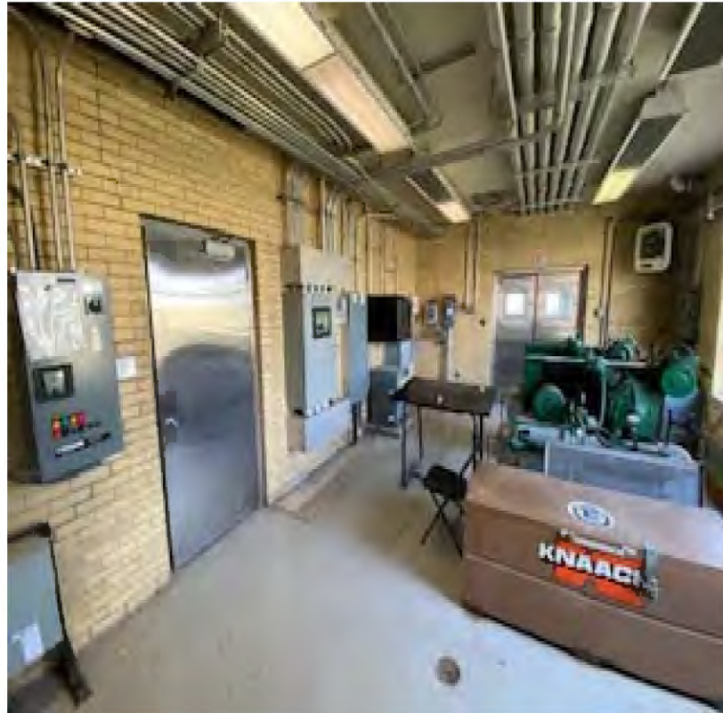
Inside the Turbine Building
