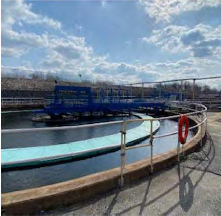
Clarifier for train 2
