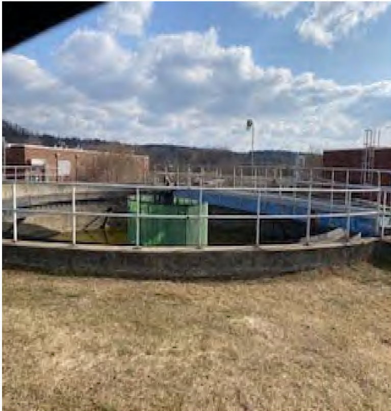
Old Clarifiers (Out of Service)
