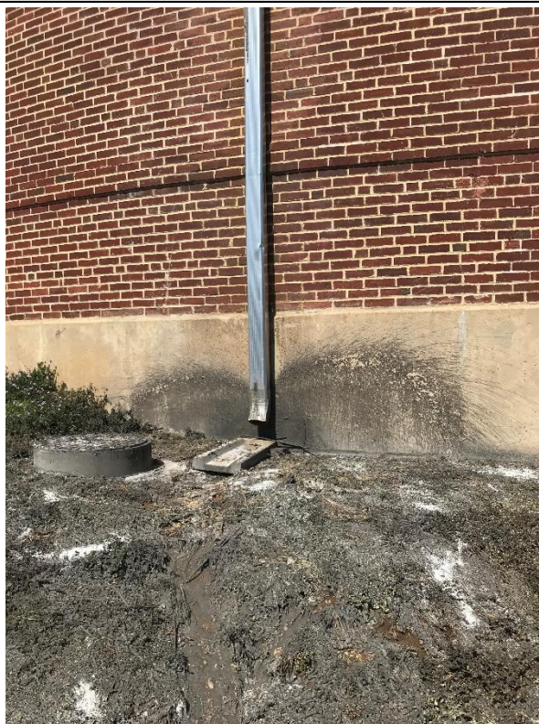
Photo 7. Closeup of where wastewater had discharged at Digester #1. Photo taken by Ashley Chong.
