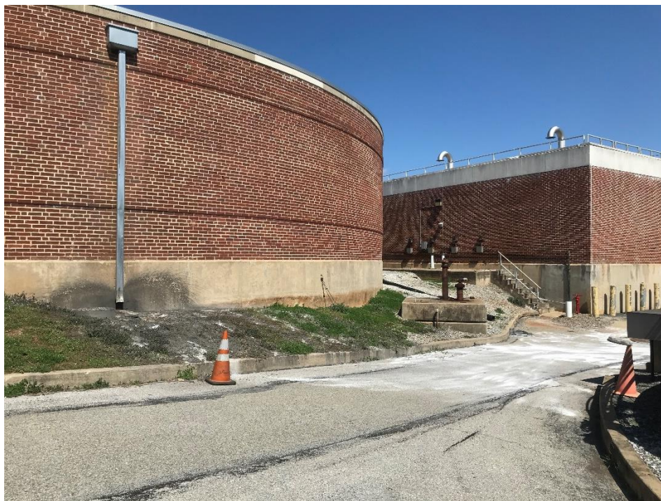
Photo 6. Stormwater drain for Digester #1 which wastewater had entered and discharged from. Photo taken by Ashley Chong.
