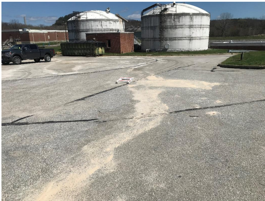
Photo 4. Lime applied to paved lot where wastewater had discharged to. Photo taken by Ashley Chong.
