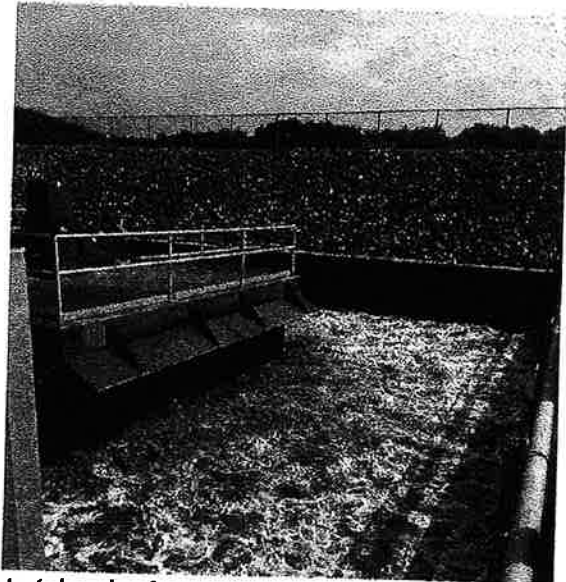
Photo taken by Austen Randecker – Aeration basin in Train #2 with foam still present on 08/15/2019
