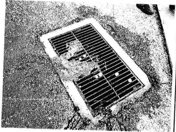
Sewage remnants on top of stormdrain. Photo taken by Austin Pardoe on 2/25/2016.
