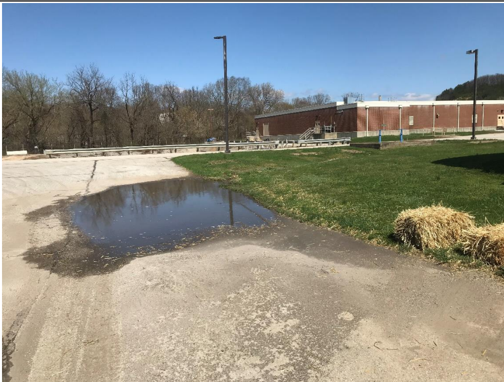
Photo 5. Low area where wastewater had pooled. Photo taken by Ashley Chong.
