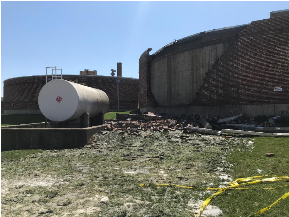
Photo 1. Collapsed brick wall of Digester 2. Photo taken by Ashley Chong.
