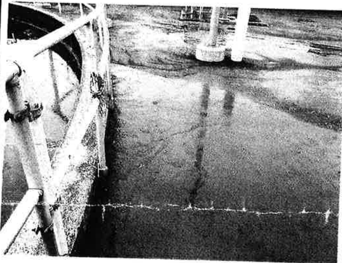
Solids on the ground adjacent to T2 clarifier. Photo taken by Austin Pardoe on 2/25/2016.
