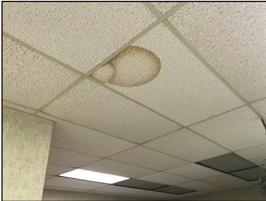
Stained ceiling tile
