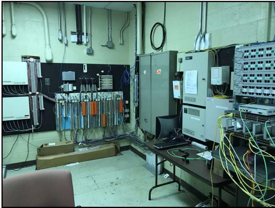
Electrical / Telephone Room
