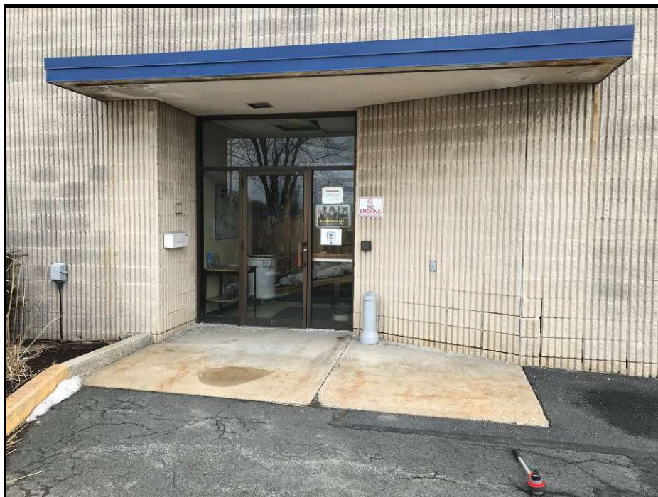
Main west entrance staining and loose exterior brick
