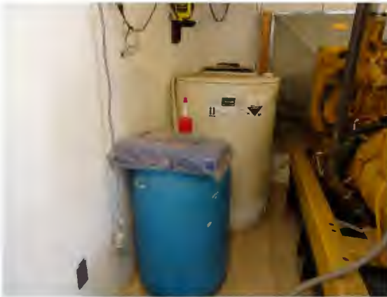
Figure 11 – Chemical Dosing System (abandoned)
