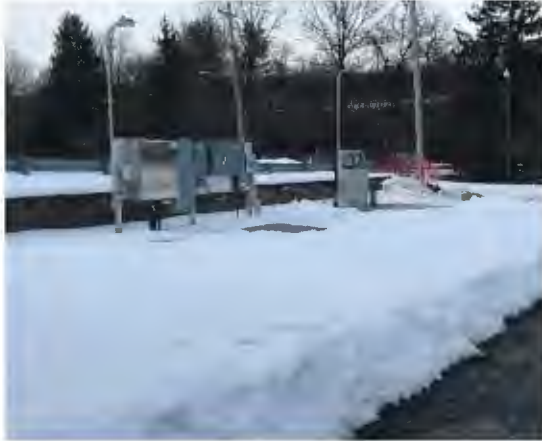
Figure 5 – MCC and Disconnects
