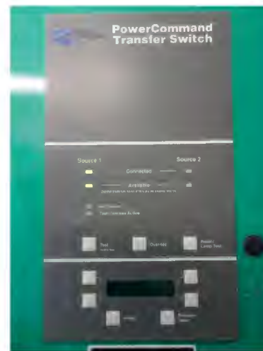
Figure 8 –Automatic Transfer Switch
