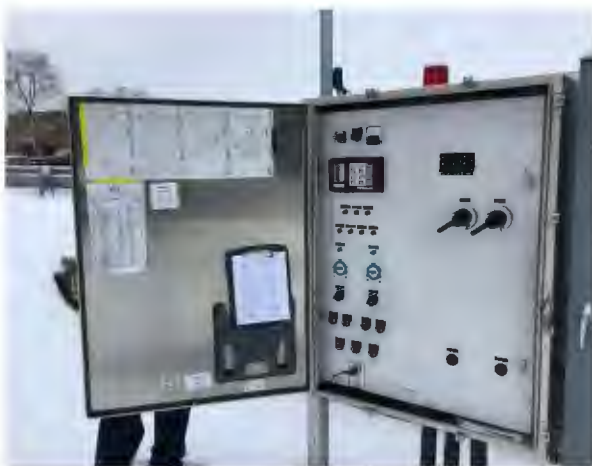
Figure 3 – Pump Control Panel
