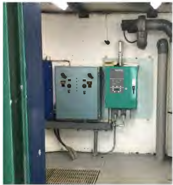
Figure 2 – Pump Control Panel and ATS
