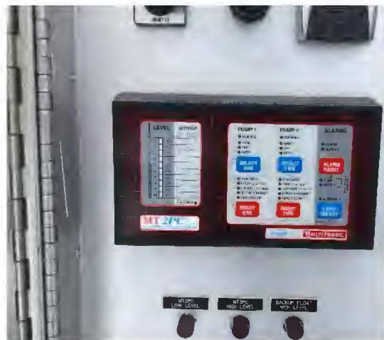
Figure 4 – Pump Control Interface
