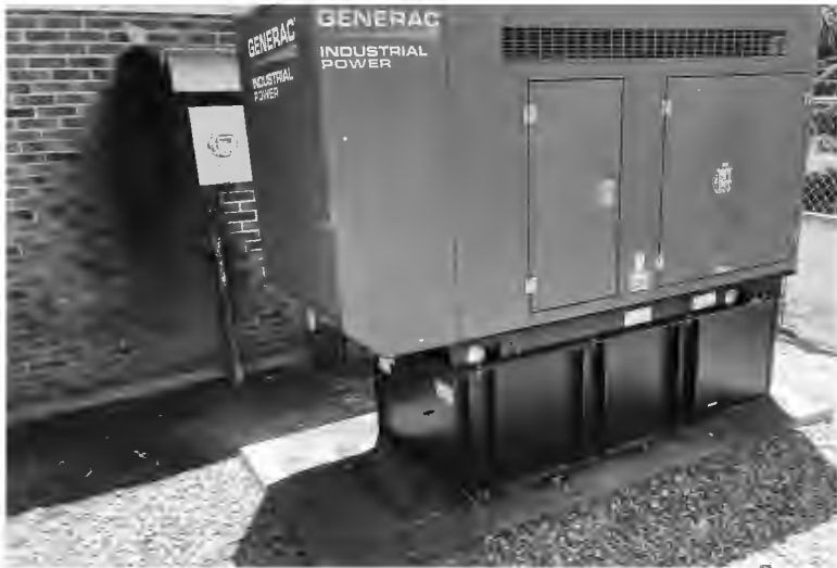
Deer Run Pump Station - P.S. 1
