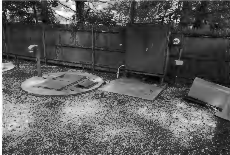
Meadowview Pump Station - P.S. 5
