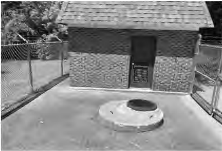
Deer Run Pump Station - P.S. 1
