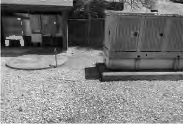
Westgate Pump Station - P.S. 8
