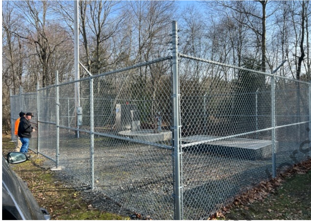
Highland pump station
