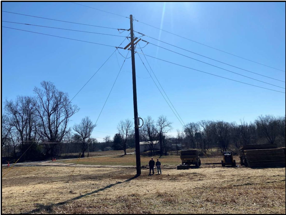
New Poles with guide wires placed across the field from my residence (1965 Sand Hill Rd)
