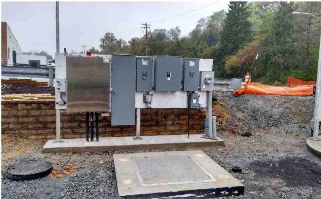
Figure 3 – Valve Vault and Electrical Equipment
