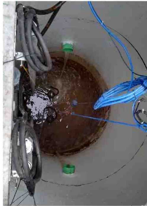
Figure 2 – Wet Well Interior
