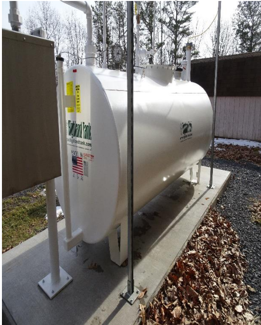
Figure 31 – Heating Oil Tanks
