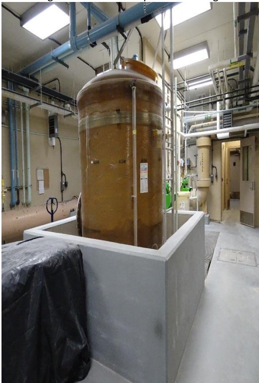
Figure 19 – Alum Storage Tank
