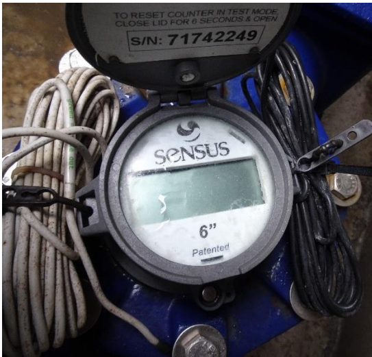
Figure 7 – Vault 2 Flow Meter
