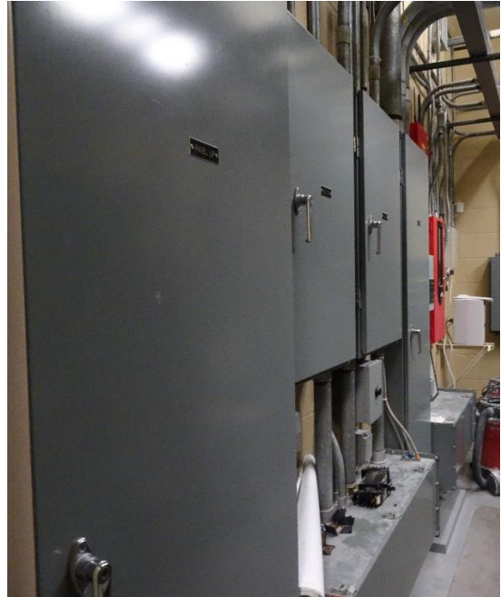
Figure 26 – Plant Electrical Room
