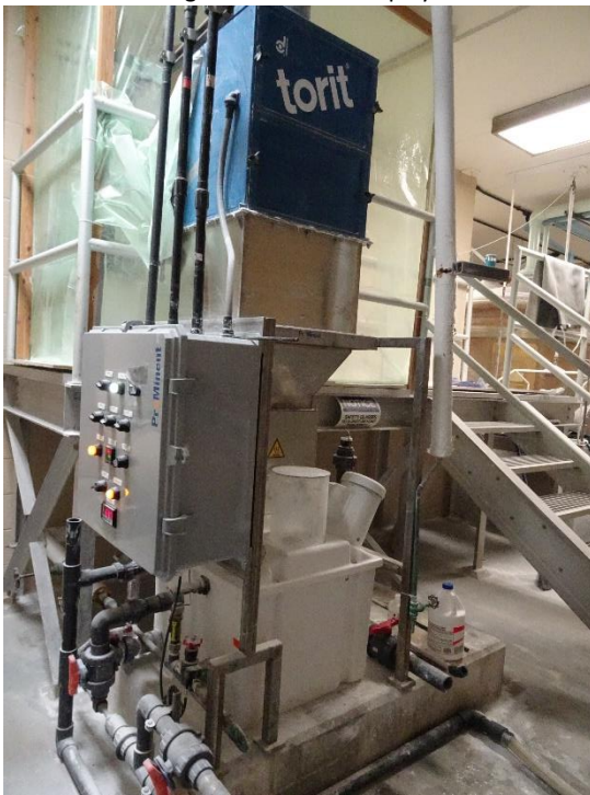
Figure 11 – Lime Mixing System
