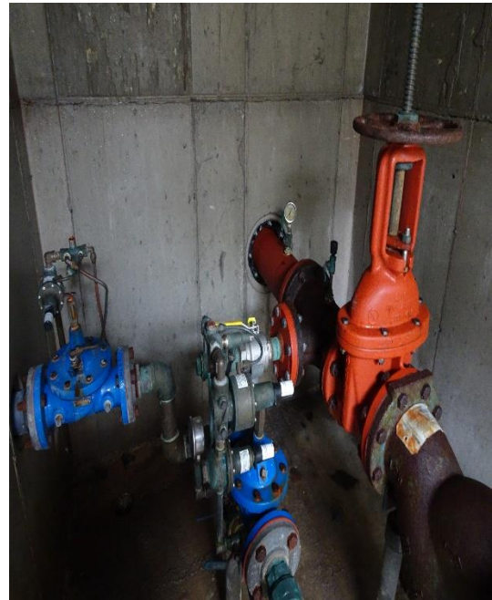
Figure 4 – Vault 2 Pressure Regulator Spur
