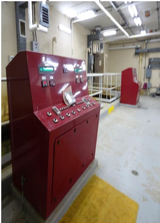
Figure 23 – Clarifier / Sand Filter Room
