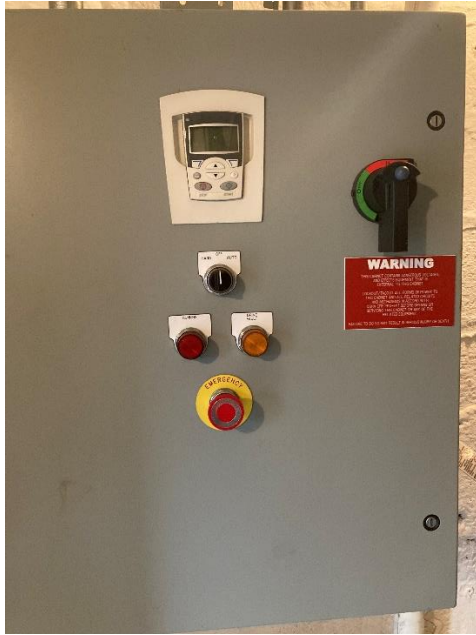
Figure 5 – Pump Control Panel
