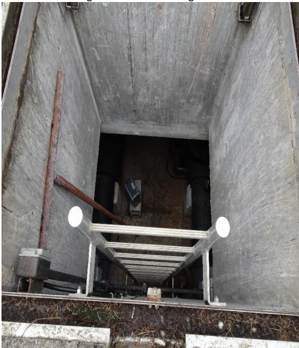
Figure 3 – Entrance to Valve Vault
