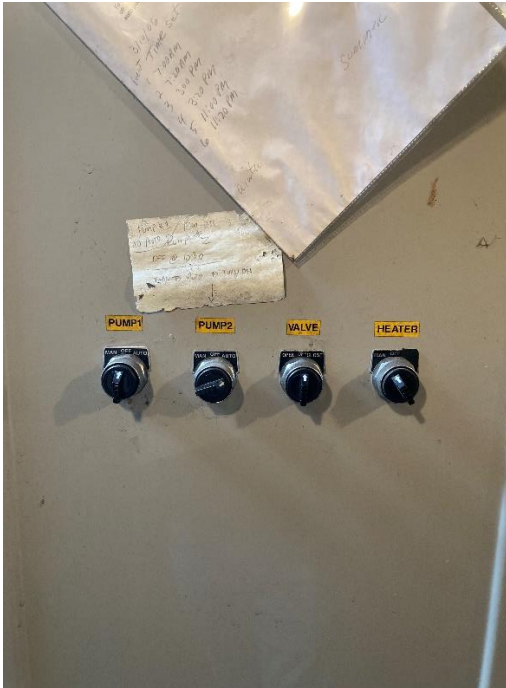
Figure 5 – Pump Control Panel
