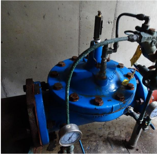
Figure 5 – Vault 2 Pressure Regulator
