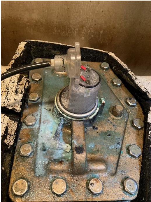
Figure 3 – Vault 1 Pressure Sensor
