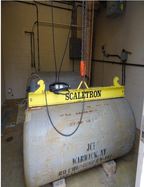
Figure 29 – Chlorine Storage Tanks
