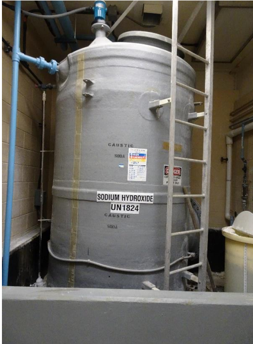
Figure 17 – Sodium Hydroxide Storage
