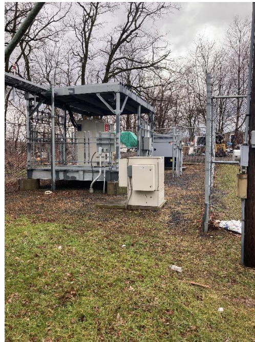
Figure 8 – Generator and Electrical Equipment for Cell Towers
